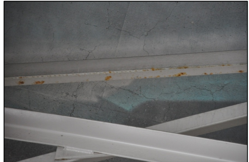
Figure 344. I-65 over Oak St.; Numerous small cracks on bottom of deck
