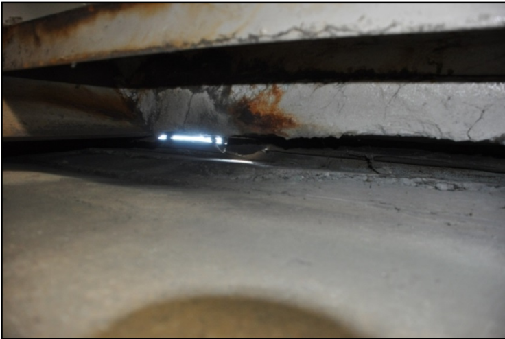
Figure 22. I-65 over Crittenden Drive, Joint seal failure
