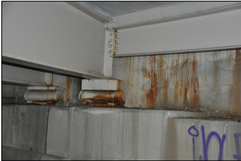
Figure 41. I-65 over Oak St.; Rust staining, deteriorating concrete, and exposed rebar #1
