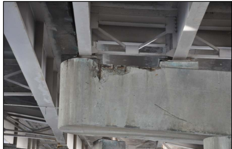
Figure 64. I-65 over Muhammad Ali Blvd. and S. Brooke St., Spalling and exposed rebar
