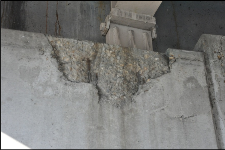
Figure 81. I-65 access ramp over Liberty St., Spalling and exposed rebar
