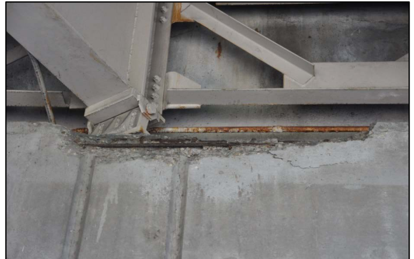
Figure 76. I-65 over Liberty St.; Staining, spalling, exposed rebar, and efflorescence #2
