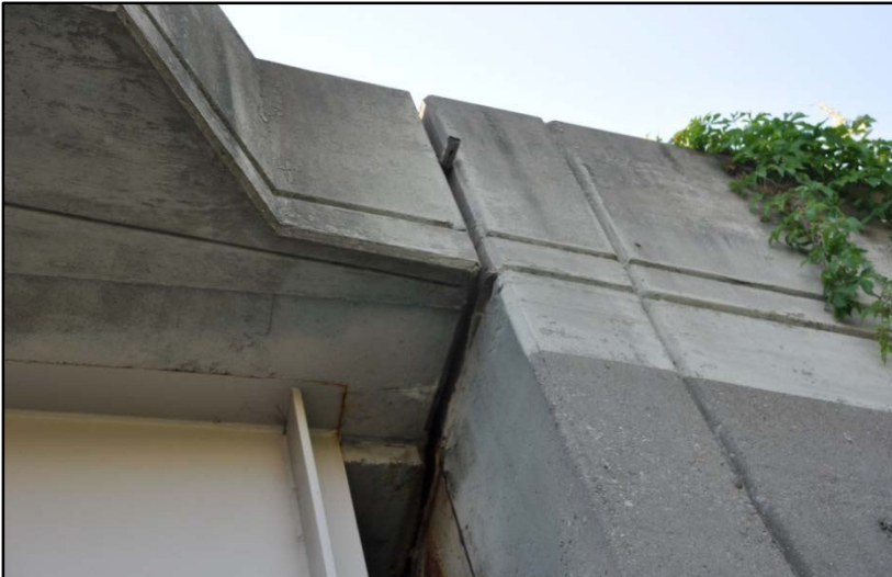
Figure 80. I-65 access ramp over Liberty St., Leaking seals
