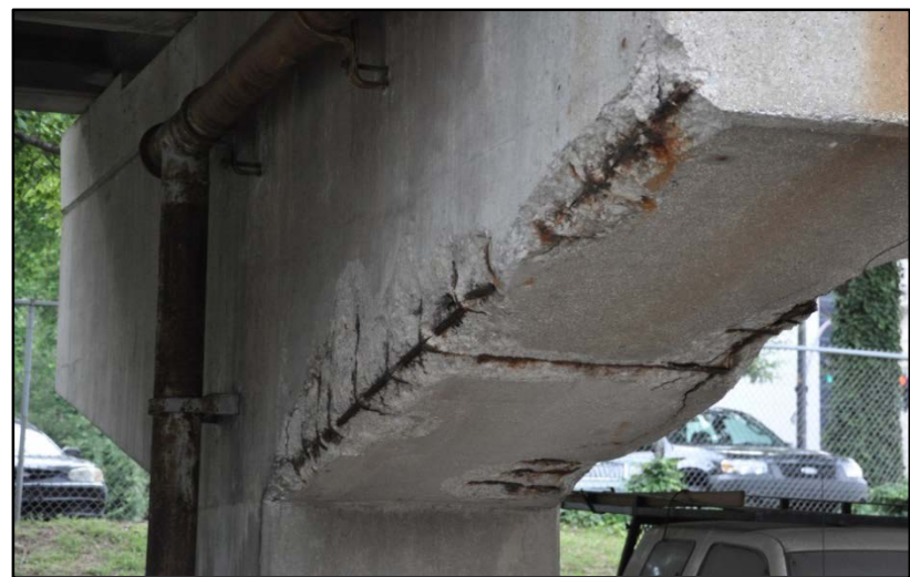
Figure 60. I-65 over E. Jacobs St., Broadway, and E. Gray St.; Drain and joint seal leaking with spalling of concrete
