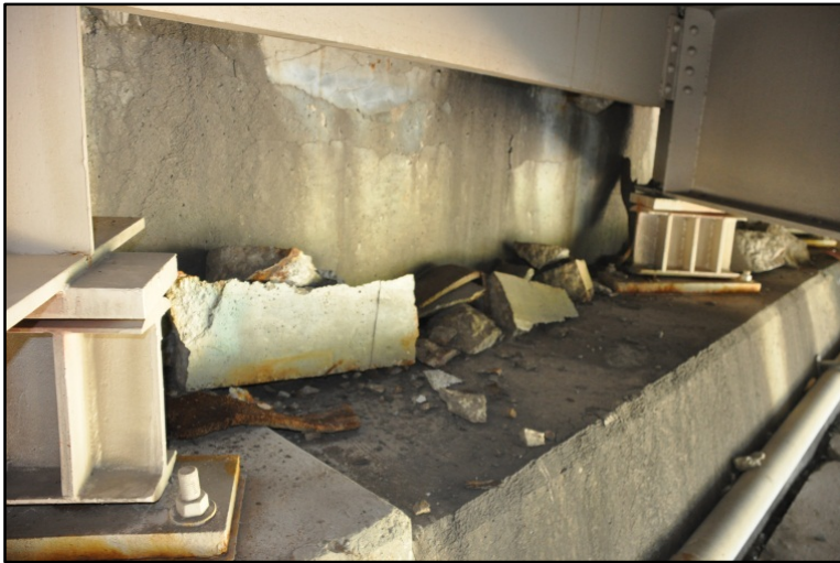
Figure 17. I-65 over Fairgrounds entrance from Bradley Ave., Large pieces of concrete from back wall near joint seal area
