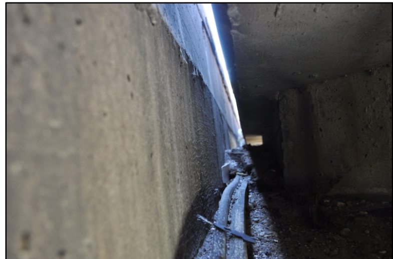
Figure 20. I-65 over Fairgrounds entrance from Bradley Ave., Joint seal failure (lying on abutment)
