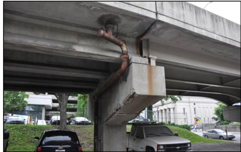
Figure 59. I-65 over E. Jacobs St., Broadway, and E. Gray St.; Drain and joint seal leaking #1
