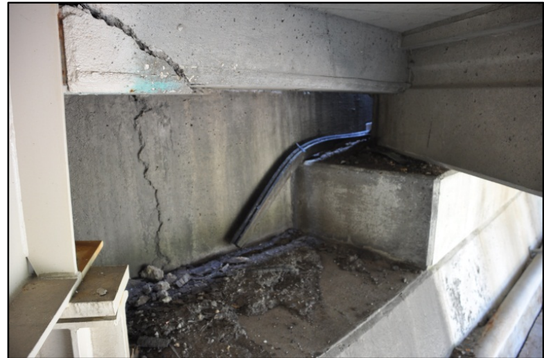
Figure 19. I-65 over Fairgrounds entrance from Bradley Ave., Joint seal failure and cracking
