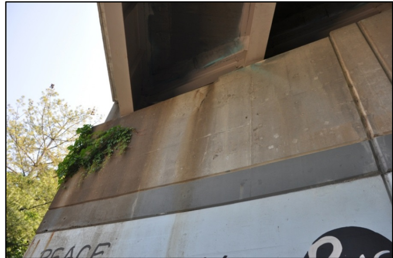
Figure 87. I-65 over S. Jackson St., Staining and cracking
