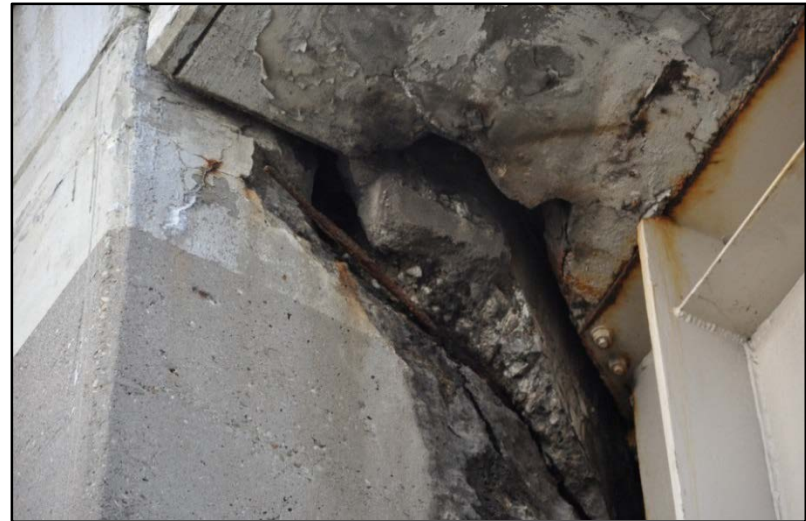
Figure 92. I-65 over E. Market St., Cracking and exposed rebar on abutment #2
