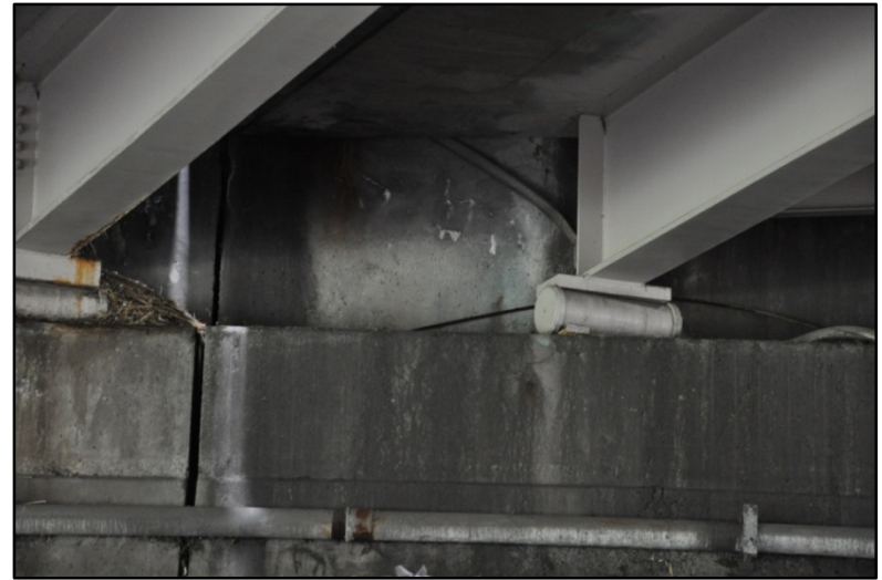
Figure 43. I-65 over Oak St.; Joint seal failure
