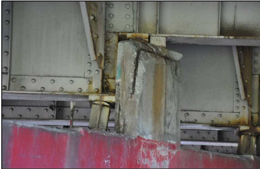
Figure 30. I-65 over Eastern Parkway, Pier cap deterioration
