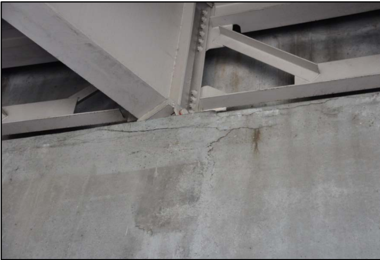
Figure 77. I-65 over Liberty St.; Cracked concrete
