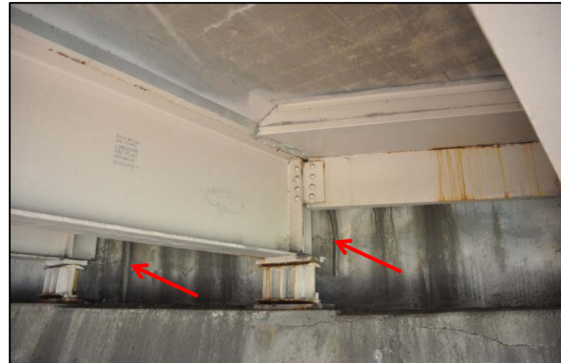
Figure 8. I-65 over Phillips Lane, Transverse cracking on the deck, efflorescence, staining on back wall (note failed joint seal)
