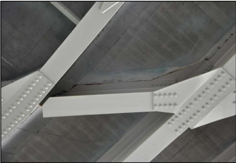
Figure 25. I-65 over Southern Railway (northwest of Crittenden), Transverse and longitudinal efflorescence
