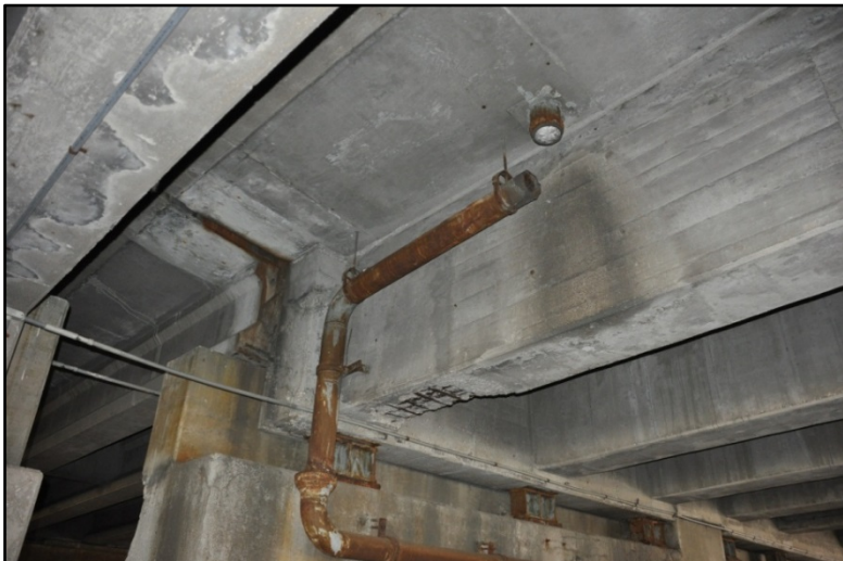
Figure 62 I-65 over E. Jacobs St., Broadway, and E. Gray St.; Leaking joint seal, damaged drain, and exposed rebar
