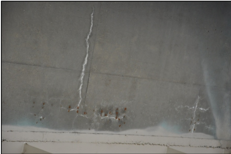
Figure 410. I-65 over S. Jackson St., Cracking and efflorescence on bottom of deck #2
