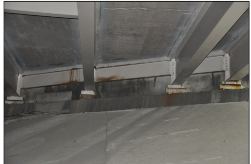
Figure 377. I-65 over E. Saint Catherine St., Staining of back wall and abutment
