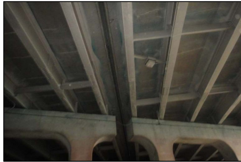
Figure 12. I-65 over Manning Street, Cracking and efflorescence on bottom of deck
