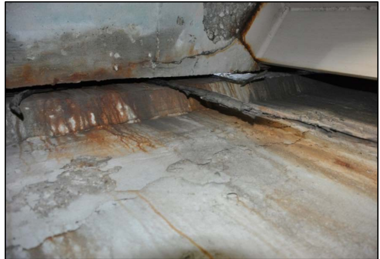
Figure 27. I-65 over Eastern Parkway, Joint seal failure
