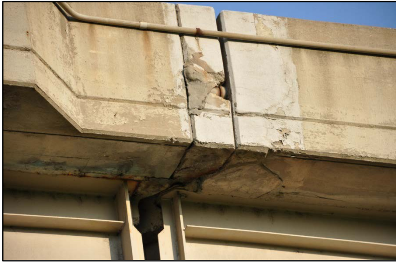
Figure 97. I-65 over E. Main St., Deterioration at joint area #2 (notice patch over conduit)
