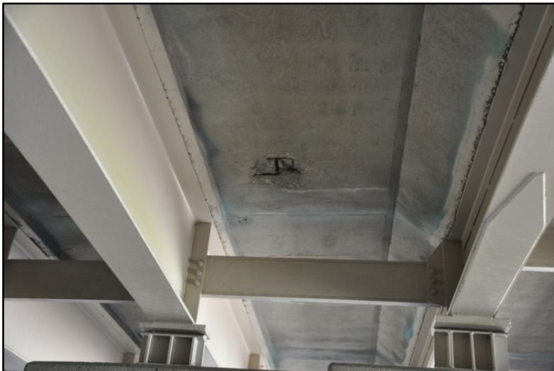
Figure 14. I-65 over East Entrance to KY Fair & Expo Center, Spalling and exposed rebar
