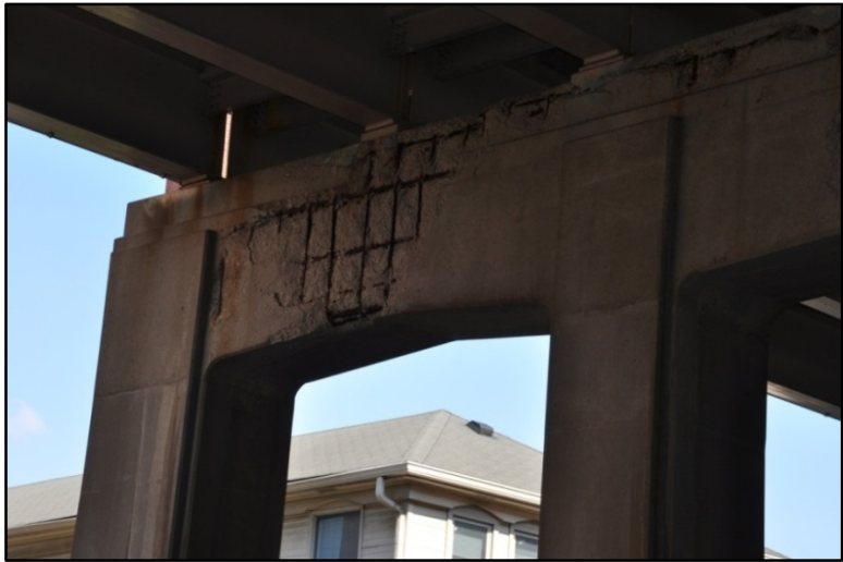
Figure 49. I-65 over E. Kentucky St. and S. Brooke St., Spalling and exposed rebar
