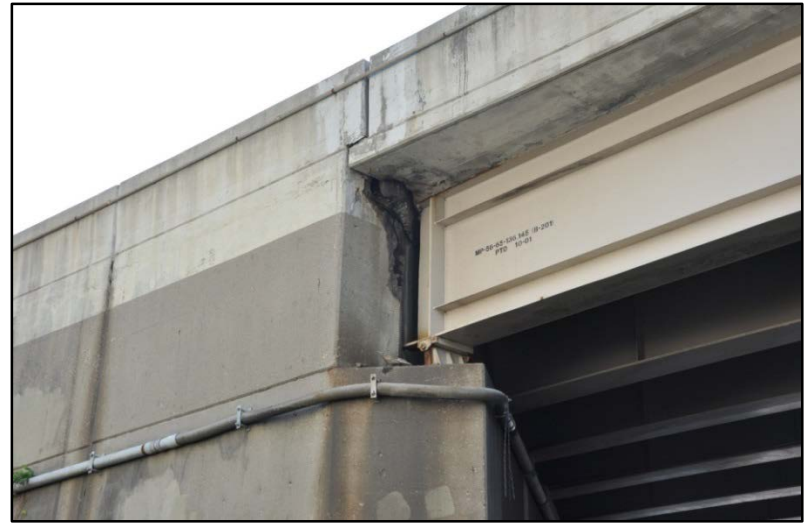
Figure 91. I-65 over E. Market St., Cracking and exposed rebar on abutment #1
