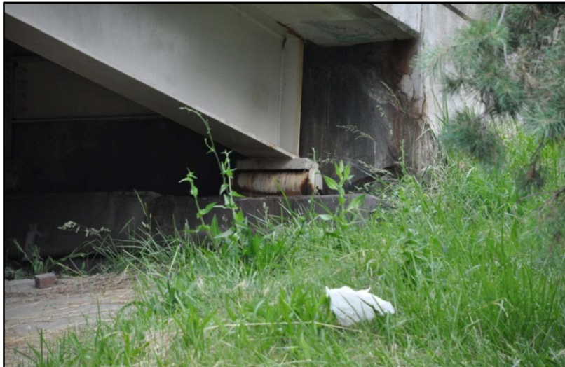
Figure 54. I-65 over Caldwell St., Evidence of failing joint seal
