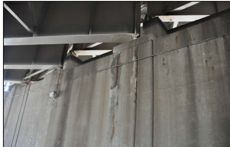
Figure 84. I-65 over Preston St. and Jefferson St., Spalling and exposed rebar
