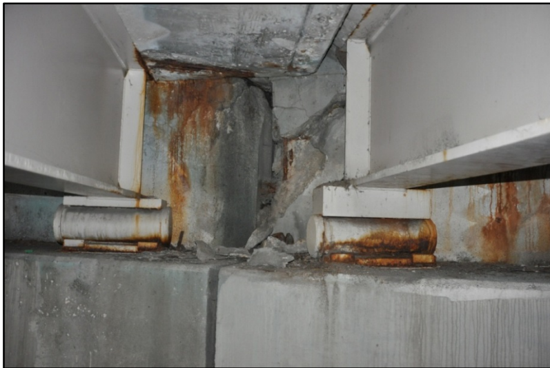
Figure 42. I-65 over Oak St.; Rust staining, deteriorating concrete, and exposed rebar #2
