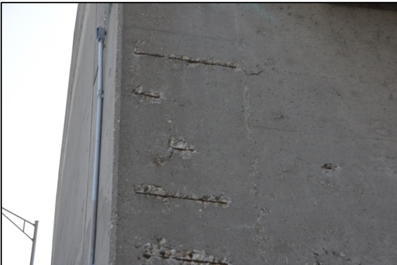
Figure 82. I-65 access ramp over Liberty St., Minor spalling and exposed rebar
