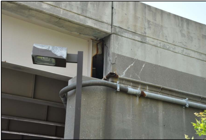
Figure 73. I-65 over S. Floyd St., Cracking and efflorescence
