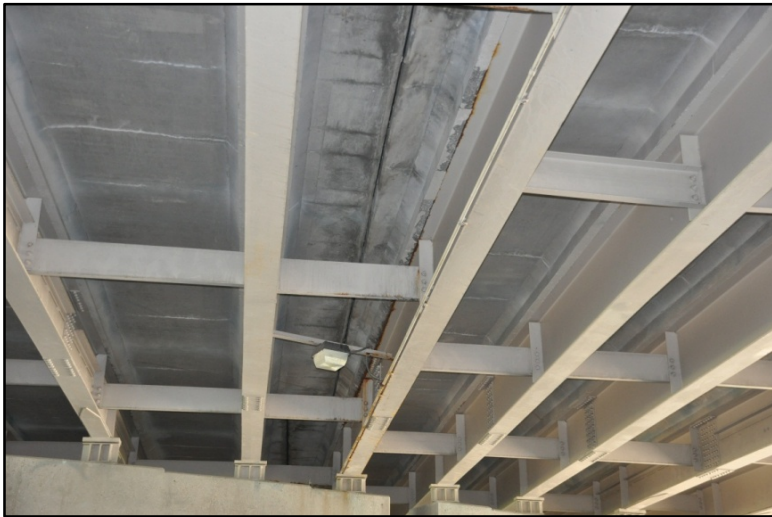
Figure 7. I-65 over Phillips Lane, Transverse cracking and efflorescence on bottom of deck
