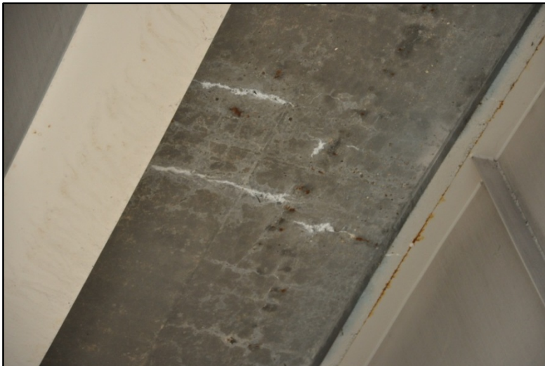
Figure 94. I-65 over E. Market St., Cracking and efflorescence on bottom of deck #2
