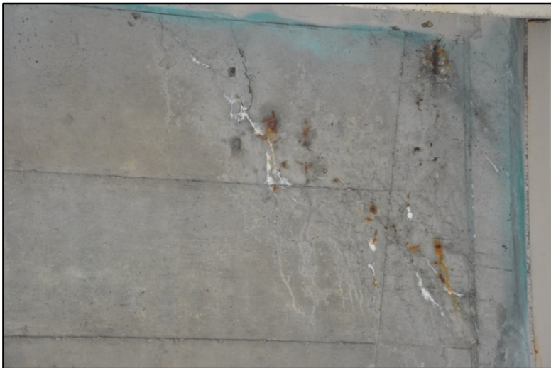
Figure 70. Access ramp from S. 1st St. to I-65 South, Cracking and efflorescence on bottom of deck #2
