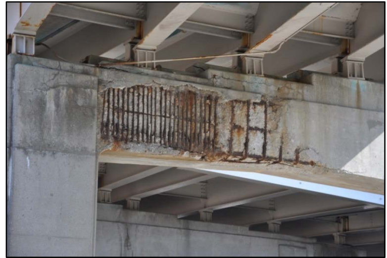
Figure 381. I-65 over E. Kentucky St. and S. Brooke St., Severe spalling #1
