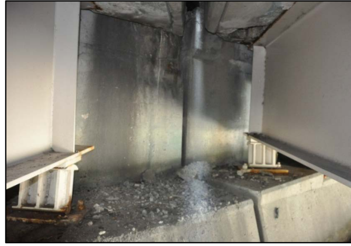
Figure 23. I-65 over Crittenden Drive, Deterioration at longitudinal joint between the north and south bound bridges
