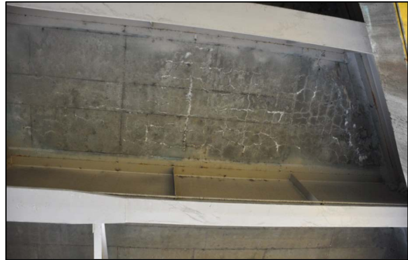
Figure 401. I-65 over S. Floyd St., Cracking and efflorescence of bottom of deck #1
