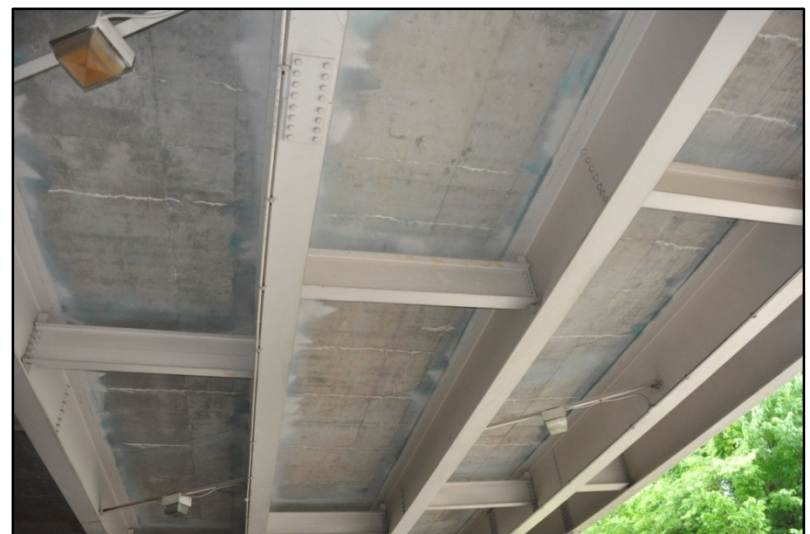
Figure 48. I-65 over E. Saint Catherine St., Transverse deck cracking and efflorescence
