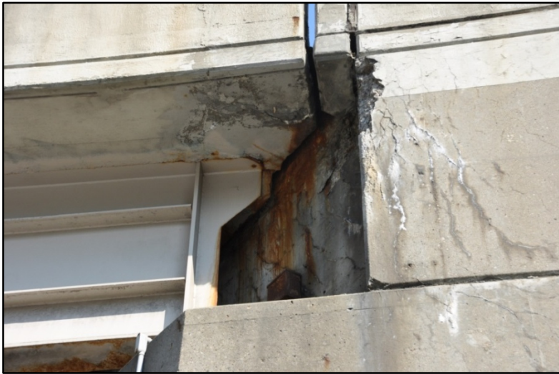
Figure 65. I-65 over Muhammad Ali Blvd. and S. Brooke St.; Staining, cracking, and spalling
