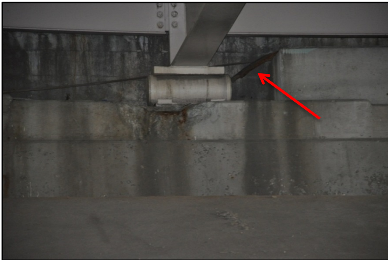
Figure 58. I-65 over College St., Deck joint seal failure
