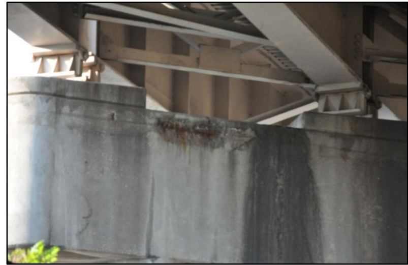
Figure 96. I-65 over E. Main St., Spalling and exposed rebar
