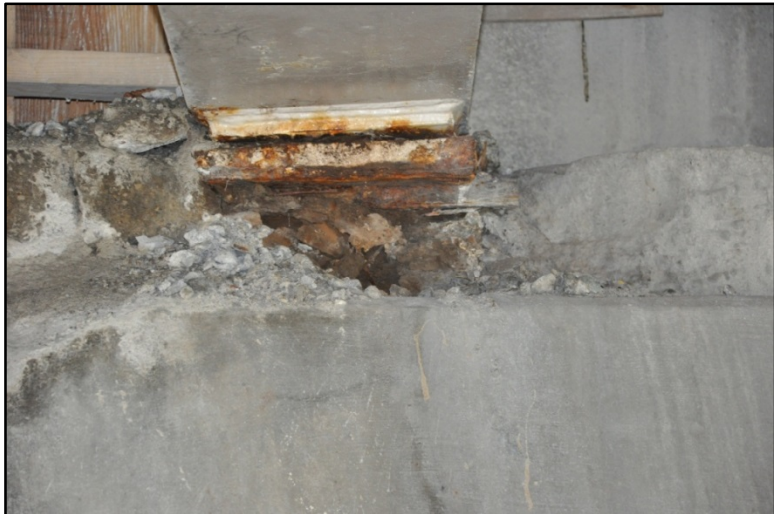
Figure 304. I-65 over East Burnett Ave., East Hill St., & CSX RR; Abutment deterioration with uneven settling
