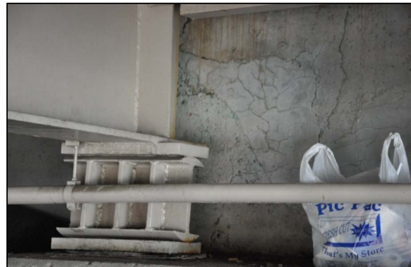
Figure 16. I-65 over East Entrance to KY Fair & Expo Center, Cracking on back wall (possible spalling repair)
