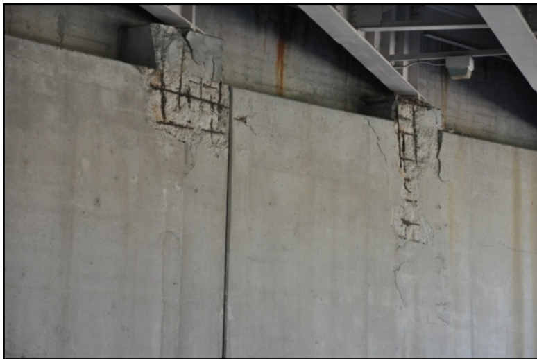
Figure 50. I-65 over E. Kentucky St. and S. Brooke St., Spalling and exposed rebar
