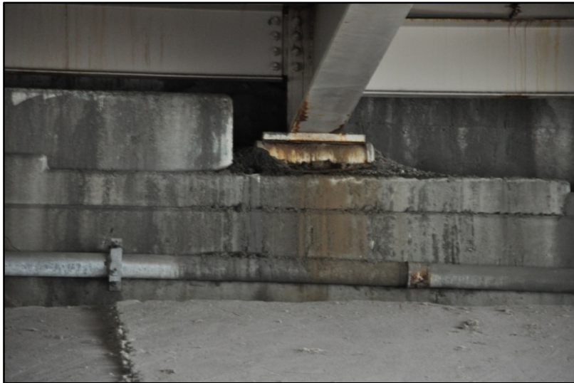
Figure 53. I-65 over Caldwell St., Abutment seat deterioration
