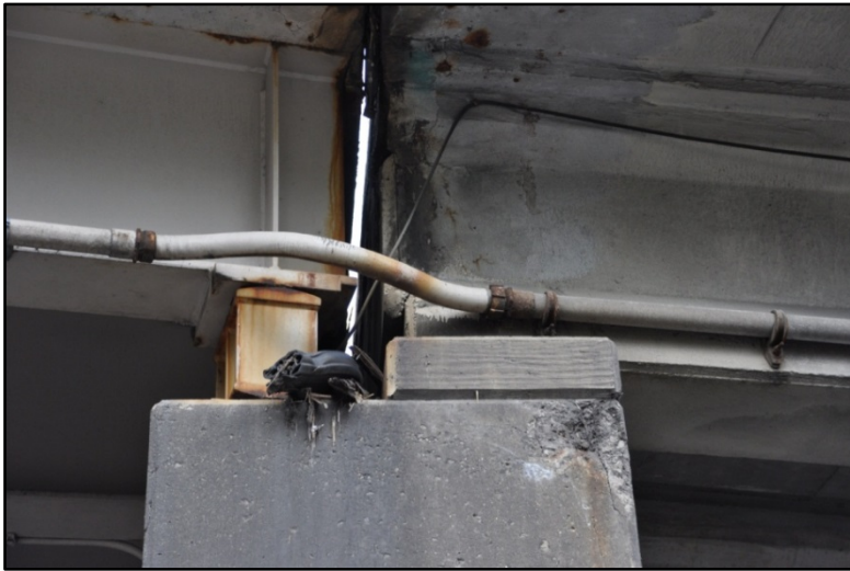
Figure 61. I-65 over E. Jacobs St., Broadway, and E. Gray St.; Joint failure
