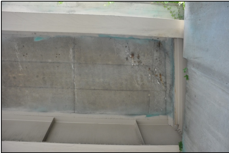
Figure 69. Access ramp from S. 1st St. to I-65 South, Cracking and efflorescence on bottom of deck #1
