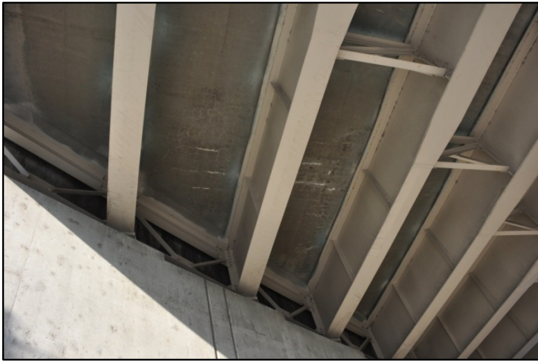
Figure 93. I-65 over E. Market St., Cracking and efflorescence on bottom of deck #1
