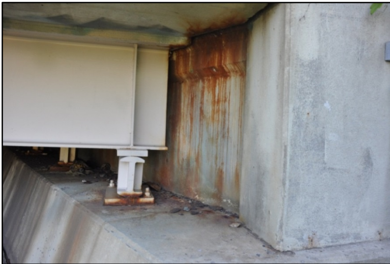
Figure 10. I-65 over Manning Street, Joint seal failure #2
