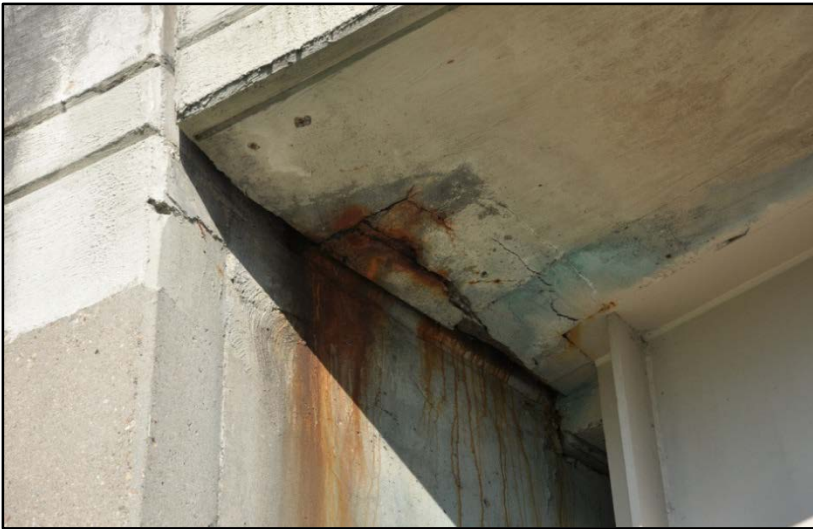
Figure 79. I-65 access ramp over Liberty St., Joint seal failure with cracking and staining
