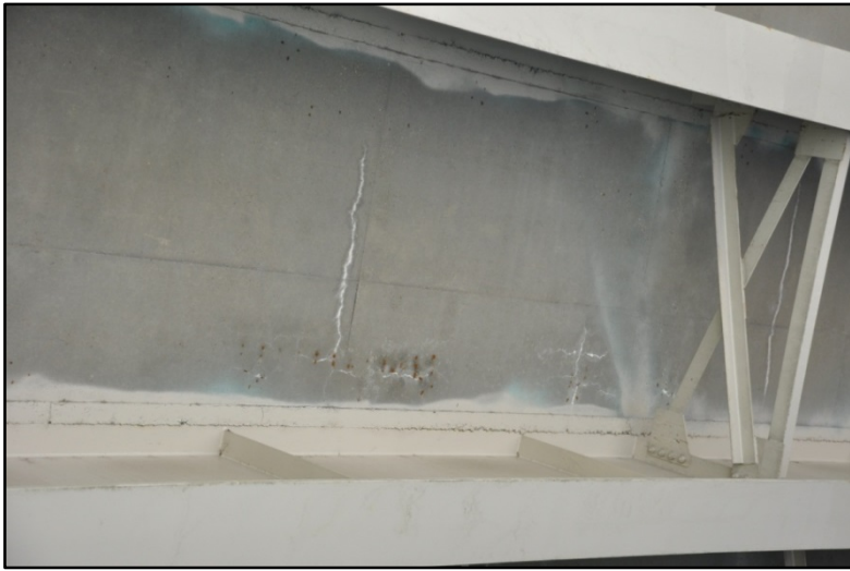
Figure 89. I-65 over S. Jackson St., Cracking and efflorescence on bottom of deck #1
