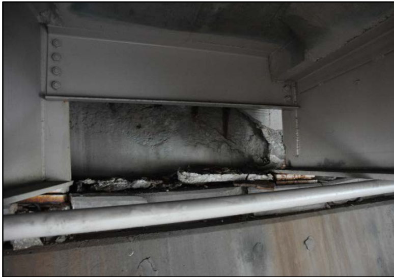
Figure 293. I-65 over East Burnett Ave., East Hill St., & CSX RR; Abutment deterioration with spalling and exposed rebar
