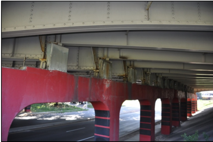
Figure 29. I-65 over Eastern Parkway, Pier cap deterioration
