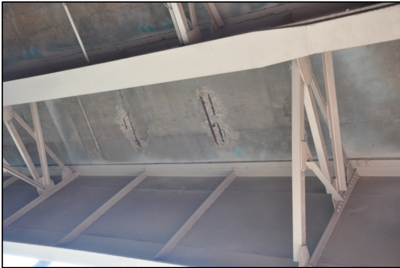
Figure 85. I-65 over Preston St. and Jefferson St., Spalling and exposed rebar #1
