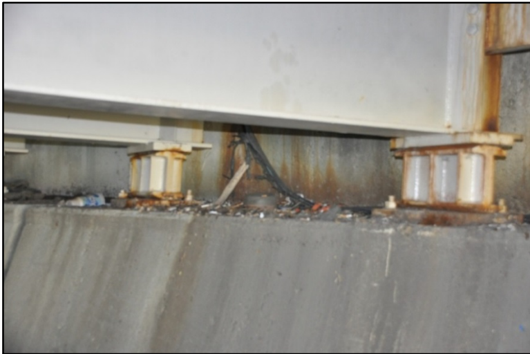
Figure 9. I-65 over Manning Street, Joint seal failure #1
