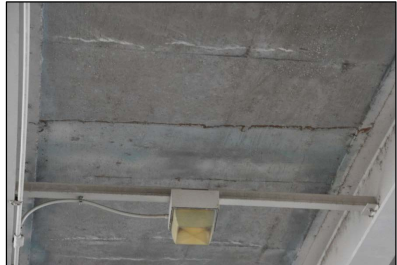
Figure 396. I-65 over Caldwell St., Transverse deck cracking and efflorescence #2
