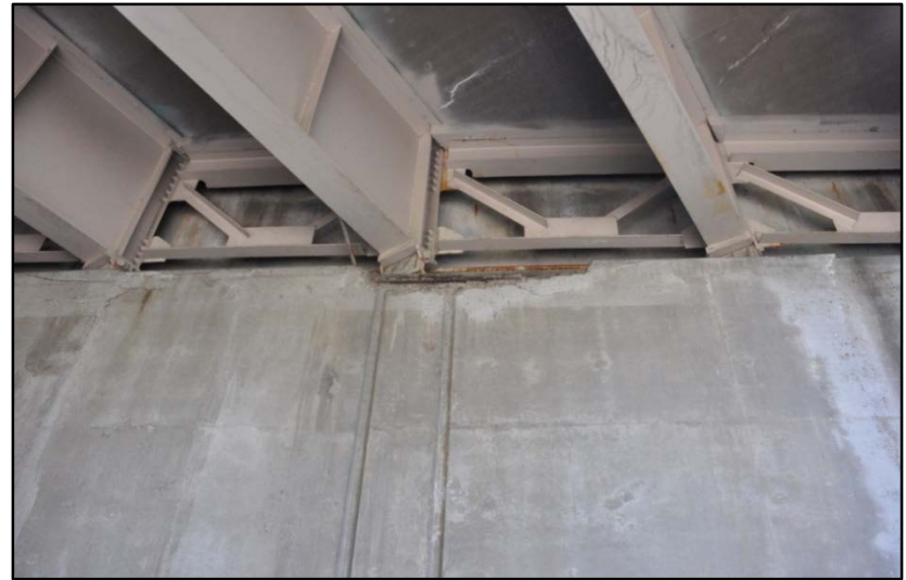
Figure 75. I-65 over Liberty St.; Staining, spalling, exposed rebar, and efflorescence #1
