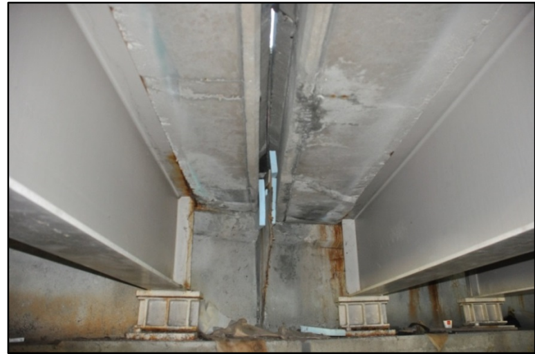
Figure 11. I-65 over Manning Street, Cracking and efflorescence on bottom of deck
