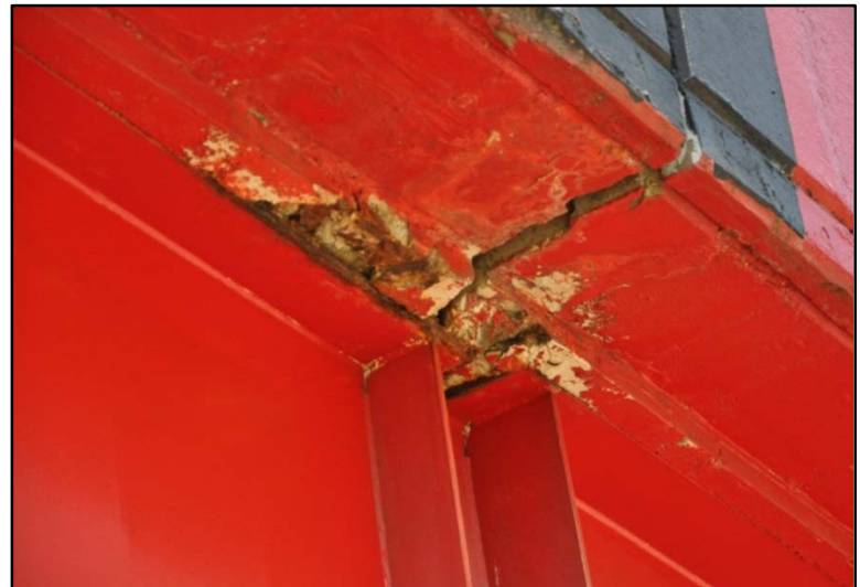
Figure 28. I-65 over Eastern Parkway, Deterioration adjacent to joint
