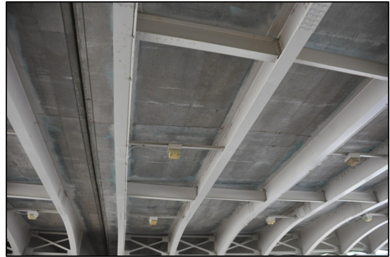
Figure 55. I-65 over Caldwell St., Transverse cracking and efflorescence #1
