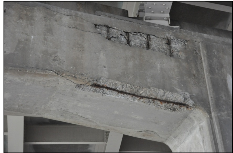
Figure 326. I-65 over East Burnett Ave., East Hill St., & CSX RR; Several areas cracking and spalling with exposed rebar
