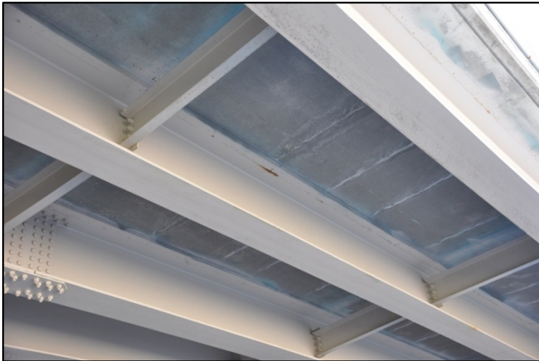
Figure 13. I-65 over East Entrance to KY Fair & Expo Center, Transverse cracking with evidence of efflorescence
