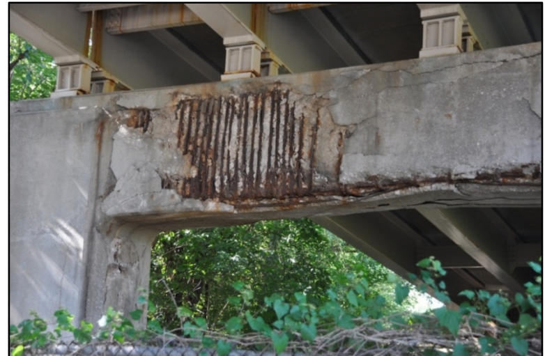
Figure 52. I-65 over E. Kentucky St. and S. Brooke St., Severe spalling #2
