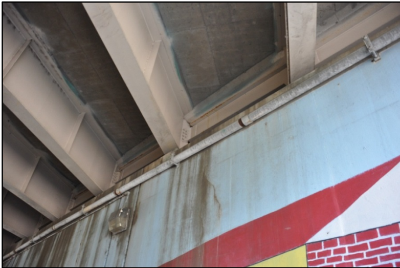
Figure 74. I-65 over S. Floyd St., Cracking and staining
