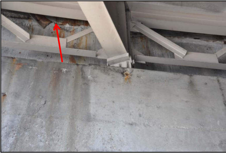
Figure 78. I-65 over Liberty St.; Joint seal failure
