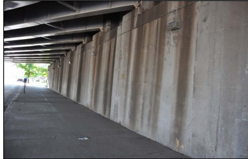
Figure 83. I-65 over Preston St. and Jefferson St., Staining of abutment wall
