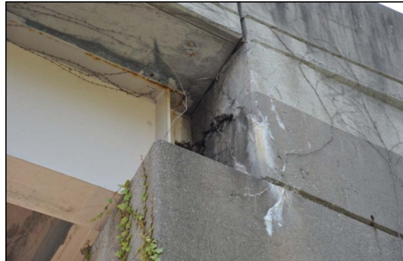
Figure 68. Access ramp from S. 1st St. to I-65 South, Cracks and efflorescence on abutment #2
