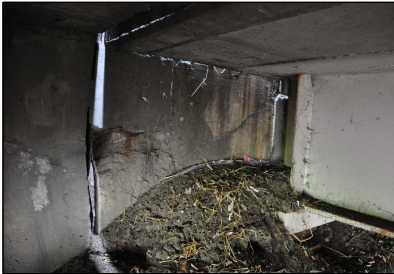
Figure 337. I-65 over East Ormsby Ave., Large amount of debris created due to missing joint seal
