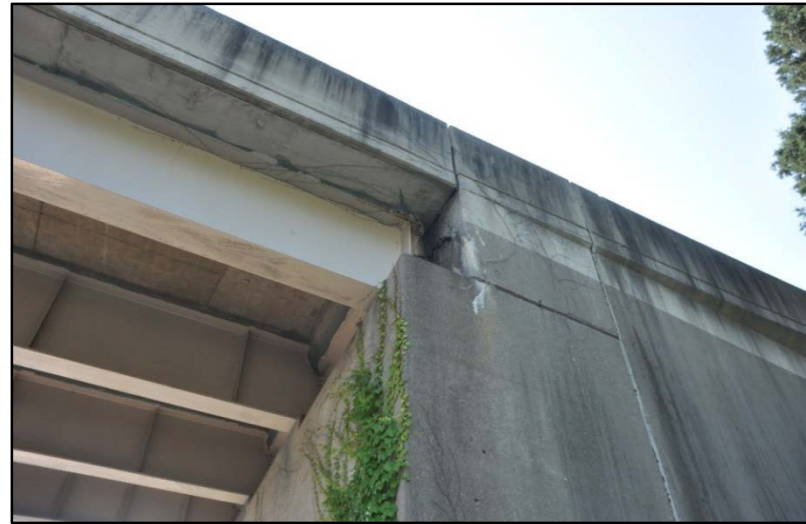
Figure 67. Access ramp from S. 1st St. to I-65 South, Cracks and efflorescence on abutment #1
