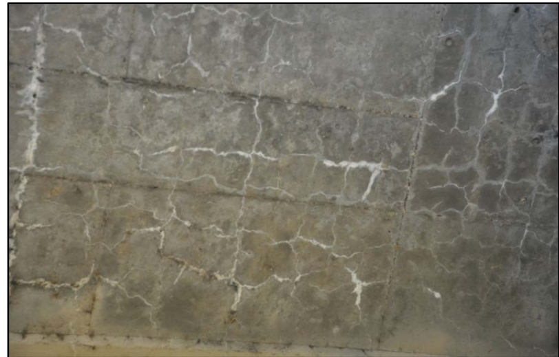
Figure 72. I-65 over S. Floyd St., Cracking and efflorescence of bottom of deck #2
