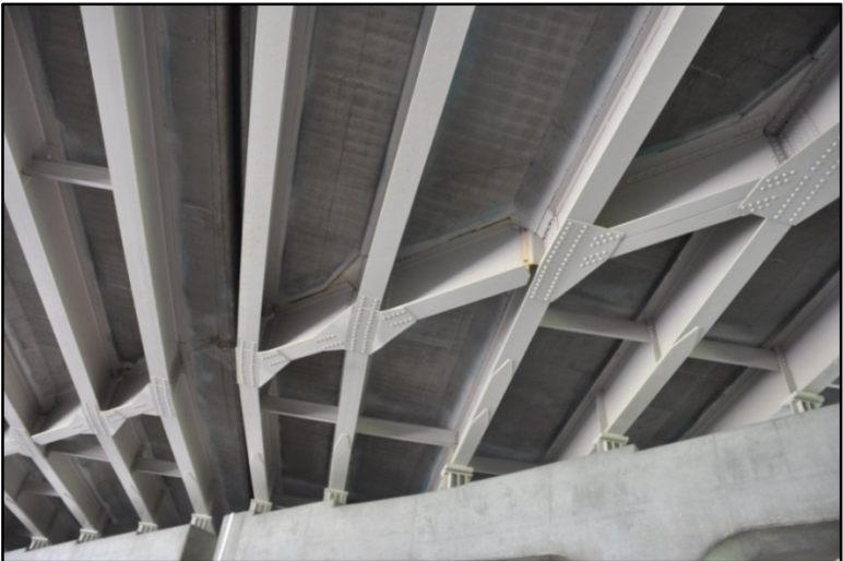
Figure 26. I-65 over Southern Railway (northwest of Crittenden), Transverse and longitudinal efflorescence
