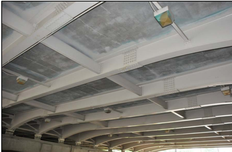
Figure 38. I-65 over East Ormsby Ave., Transverse cracking on bottom of deck
