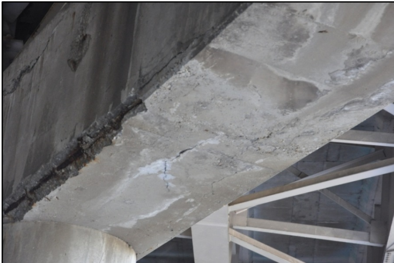
Figure 66. I-65 over Muhammad Ali Blvd. and S. Brooke St., Cracking, spalling, and efflorescence on pier
