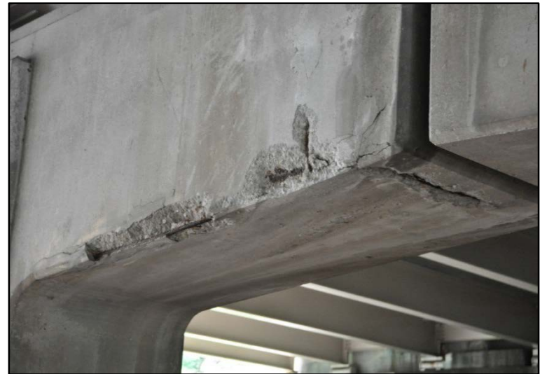
Figure 40. I-65 over East Ormsby Ave.; Cracking, spalling, and exposed rebar on pier #2
