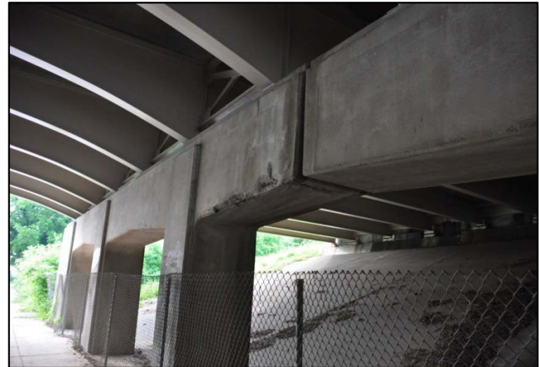
Figure 39. I-65 over East Ormsby Ave.; Cracking, spalling, and exposed rebar on pier #1
