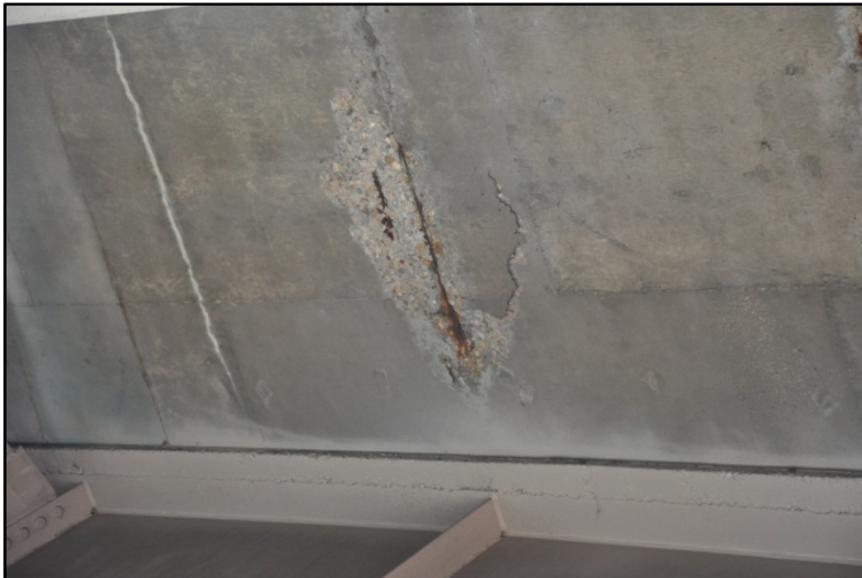
Figure 86. I-65 over Preston St. and Jefferson St., Spalling and exposed rebar #2
