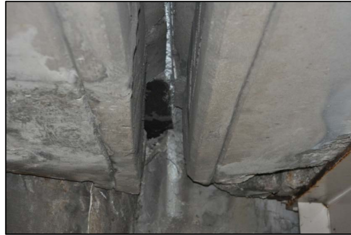
Figure 24. I-65 over Crittenden Drive, Deterioration at longitudinal joint between the north and south bound bridges
