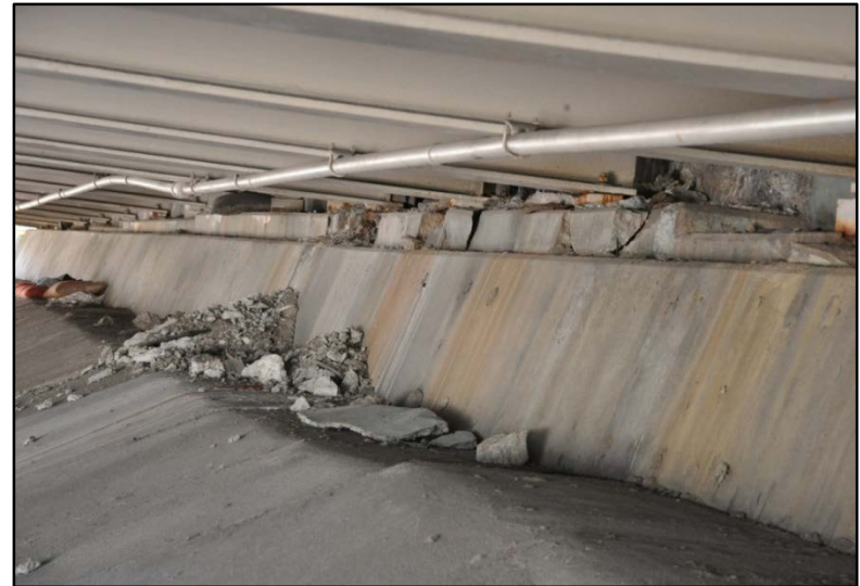
Figure 31. I-65 over East Burnett Ave., East Hill St., & CSX RR; Deterioration of the abutment seats #1
