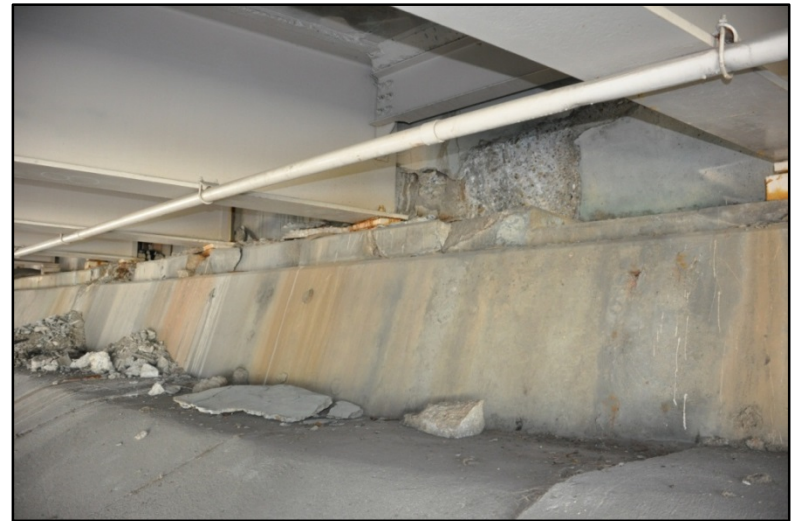
Figure 282. I-65 over East Burnett Ave., East Hill St., & CSX RR; Deterioration of the abutment seats #2
