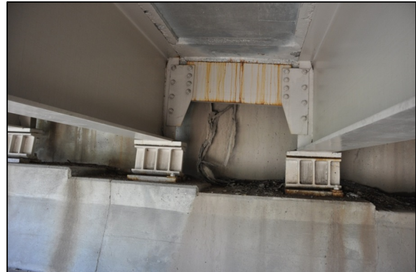
Figure 15. I-65 over East Entrance to KY Fair & Expo Center, Joint failure
