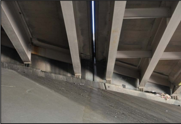
Figure 21. I-65 over Crittenden Drive, Staining from leaking joint seal
