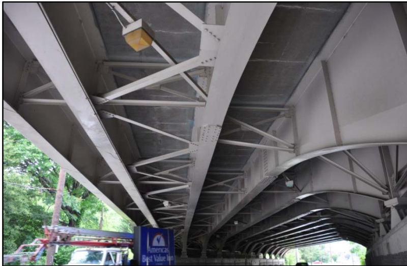
Figure 355. I-65 over S. Floyd St., Cracking and efflorescence on bottom of deck
