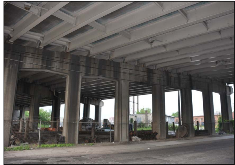
Figure 315. I-65 over East Burnett Ave., East Hill St., & CSX RR; Piers show evidence of staining from leaking joint
