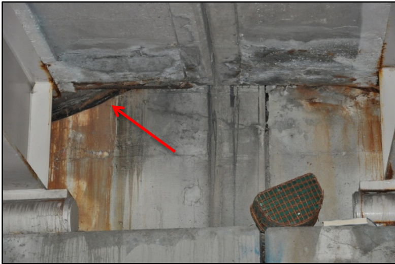
Figure 57. I-65 over College St., Spalling, exposed rebar and joint failure
