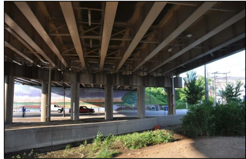
Figure 95. I-65 over E. Main St., Staining on piers
