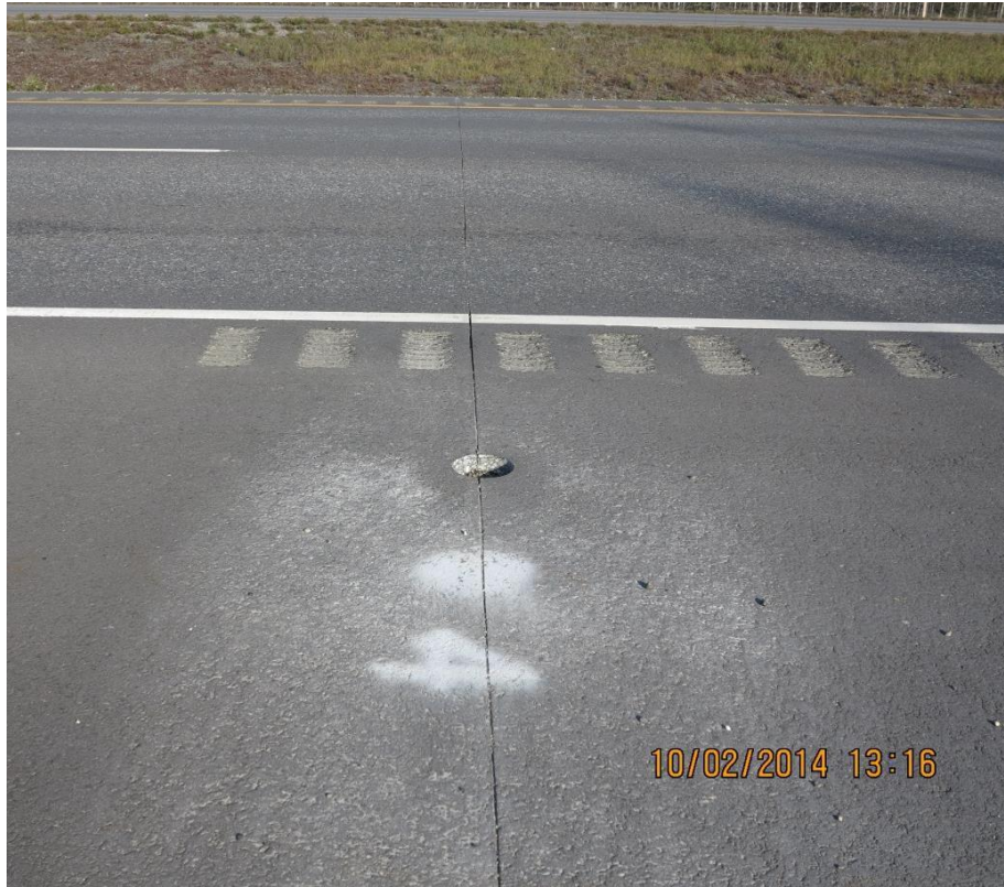
Figure 9. Precut non-active crack at ~ Station 1005+24
