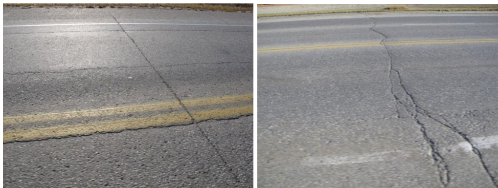
Figure 1. 25+ year old major transverse thermal cracks, precut (lt.) natural (rt.)
