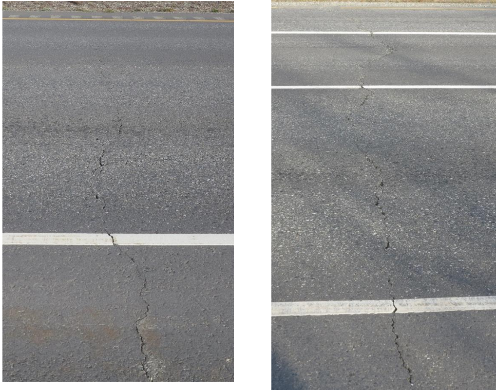
Figure 8. Natural transverse cracks at ~ Stations 999+27 (lt.) & 1029+13 (rt.)
