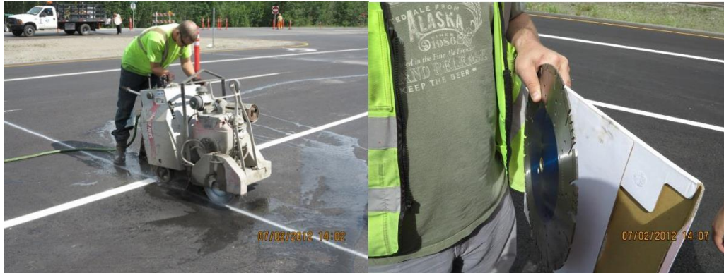
Figure 5. Saw Devil equipment and operator (lt) and thin diamond saw blade used (rt)
