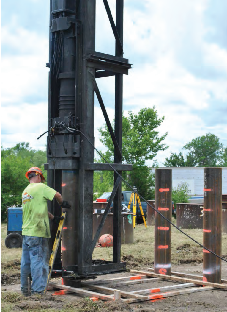
Figure 3.13. Crew marked piles every 5 blows once the piles began penetrating shale. Pile driving was terminated when the piles penetrated 2 in. or less in 5 blows.
