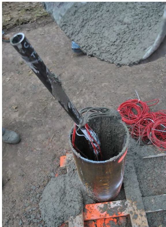
Figure 3.19. Damaged bar for CIP-1.
