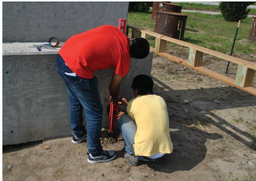
Figure 3.48. Installing wireline device.
