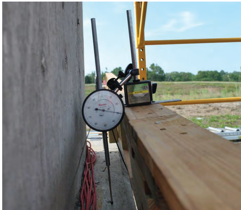
Figure 3.46. Dial gages used to measure uplift at the back of the pile cap.
