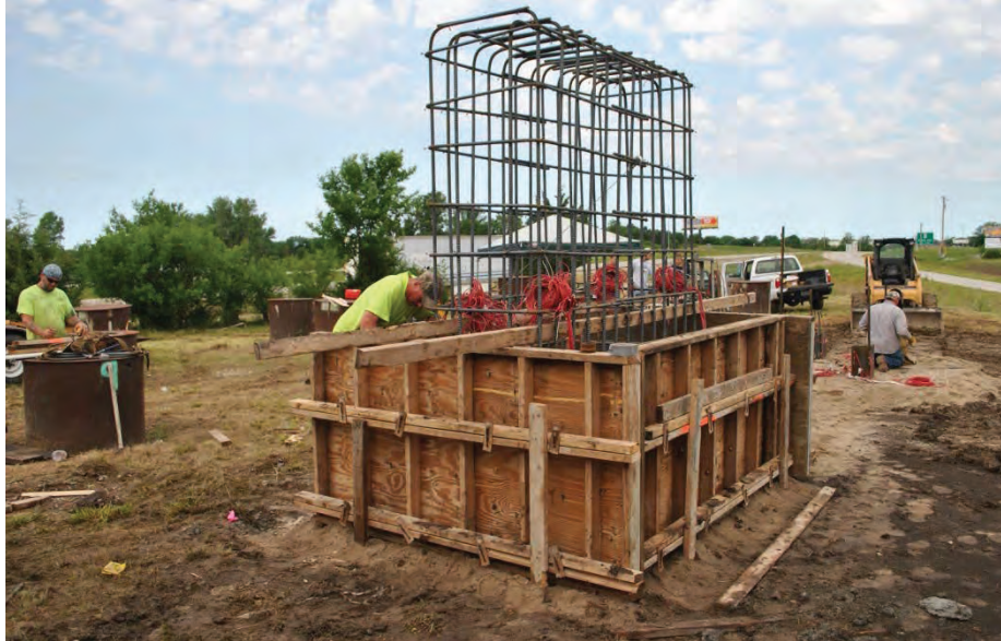
Figure 3.25. Stem cage formed with pile cap cage prior to placement of concrete for pile cap.
