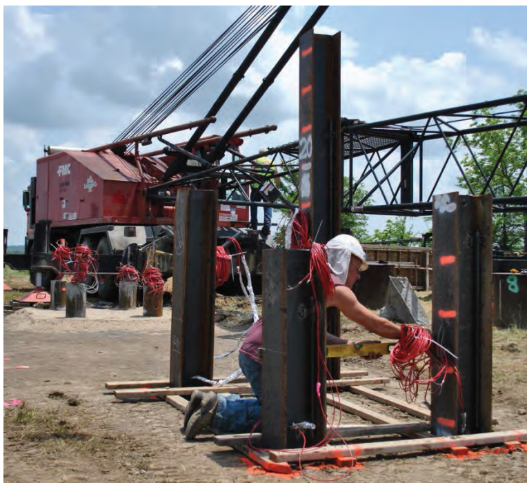
Figure 3.16. Marking pile lengths to be removed. (H-Piles were delivered in various lengths; variation in stickup shown is not an indication of variation in penetration.)
