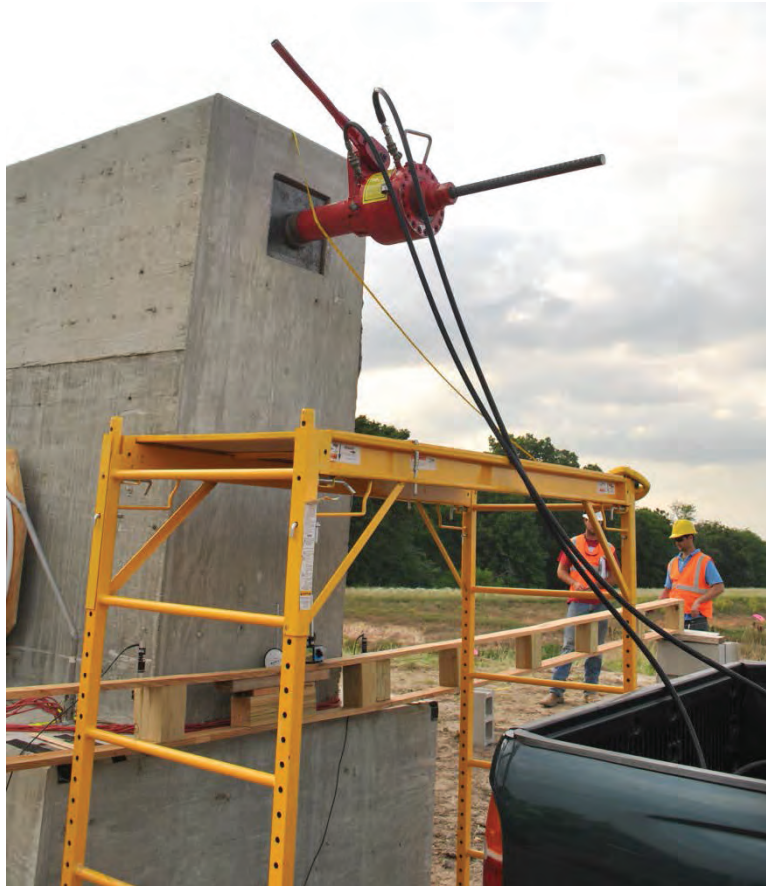
Figure 3.49. Hydraulic jack on threadbar applying load to pile structure through a bearing plate.
