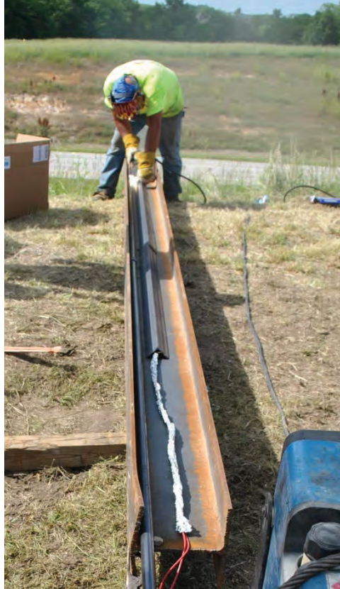
Figure 3.36. Welding angle section above installed gages. Gage cables were wrapped in aluminum foil to protect from heat.
