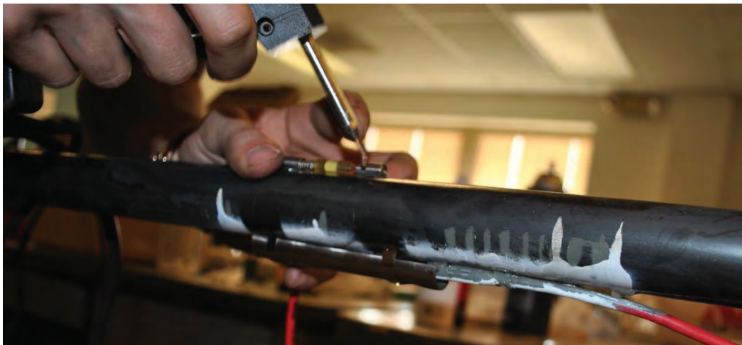
Figure 3.38. Spot welding Geokon 4150 gage to instrumented pipe. Completed gage with protective cover can be seen on bottom of pipe.
