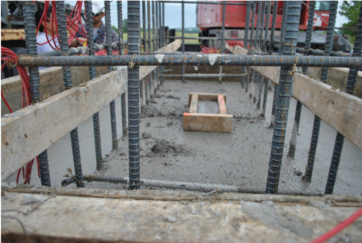
Figure 3.29. Finished concrete for pile cap with beveled keyway at joint between cap and stem.
