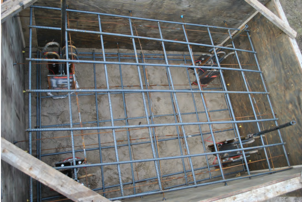
Figure 3.23. Forms and cage in place for H-pile cap prior to placing concrete.
