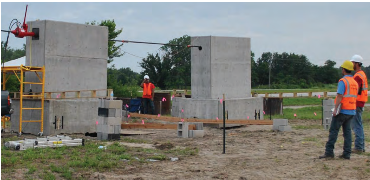
Figure 3.54. Pile structures during final load step. CIP pile cap is at left and H-pile cap is at right.
