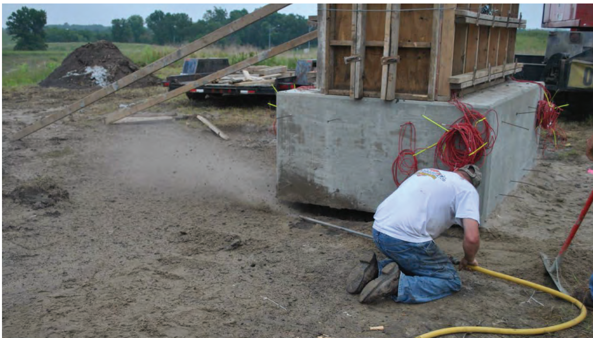
Figure 3.32. Removing sand from beneath pile cap to create a gap between cap and ground surface. The gap prevents the cap from bearing on the ground surface during the application of overturning loads.
