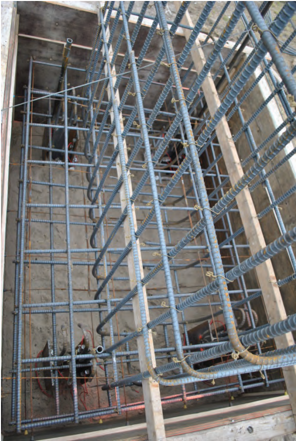
Figure 3.24. H-pile cap and stem cages formed together prior to placing concrete for the pile caps.
