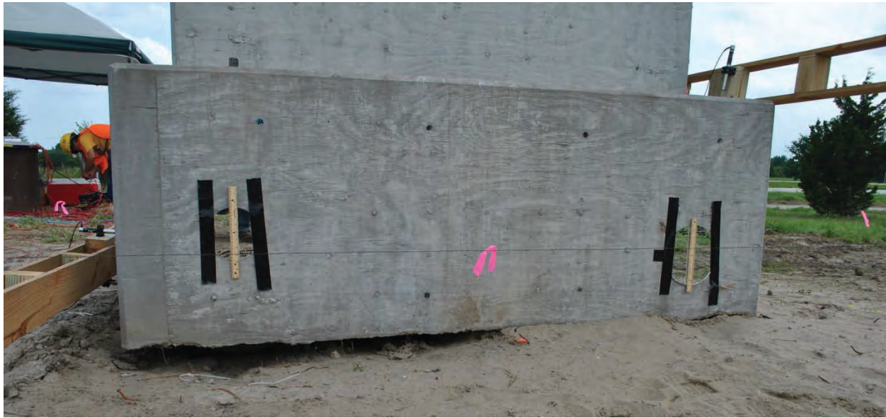
Figure 3.47. Wireline devices on the CIP pile group. Devices were installed in line with compression (left) and tension (right) piles.
