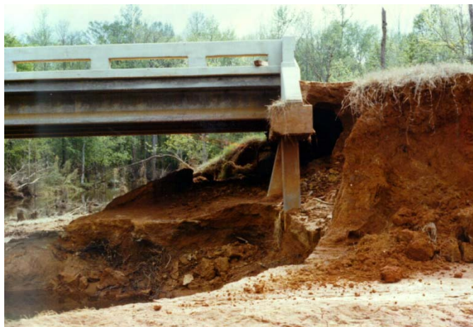
Figure 1-1. Example of Bridge Scour
