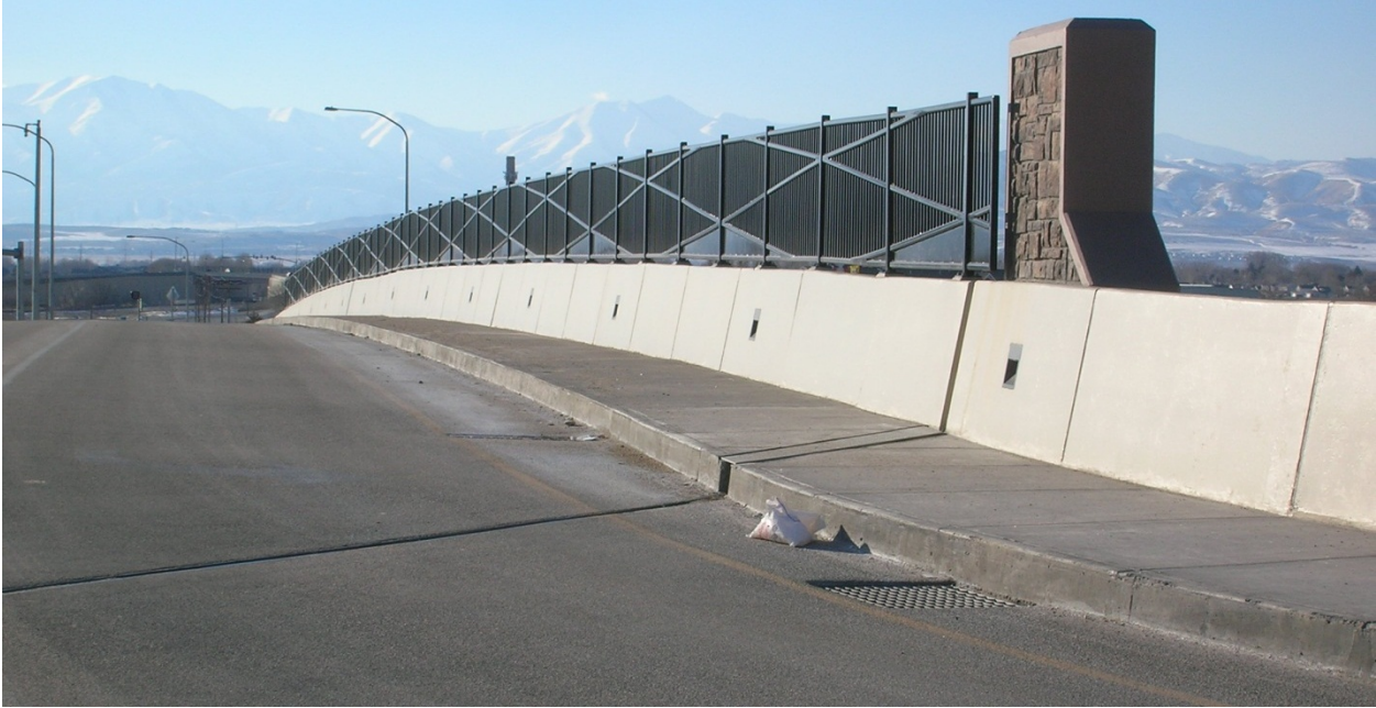
Exhibit 1-10. Sidewalk and recessed lighting located on the bridge at the Pioneer Crossing and Interstate 15 DDI (American Fork, UT). (6)
