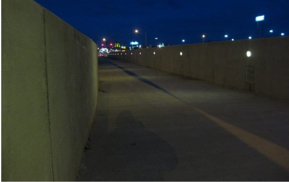
Exhibit 8-34. Recessed lighting in DDI center walkway. (14)
