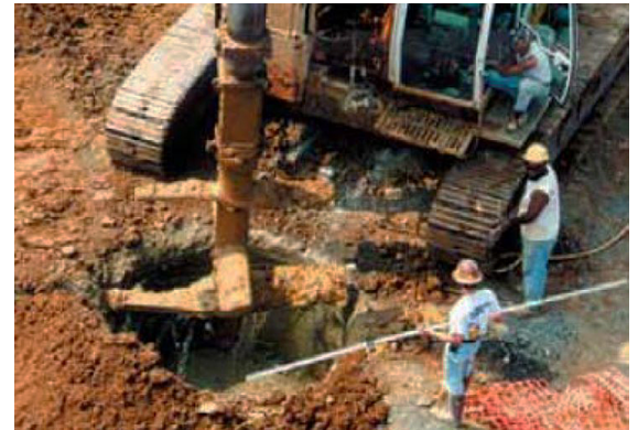
A soil-mixing operation in progress. An auger drills down to mix soil with binder, creating supporting columns.
