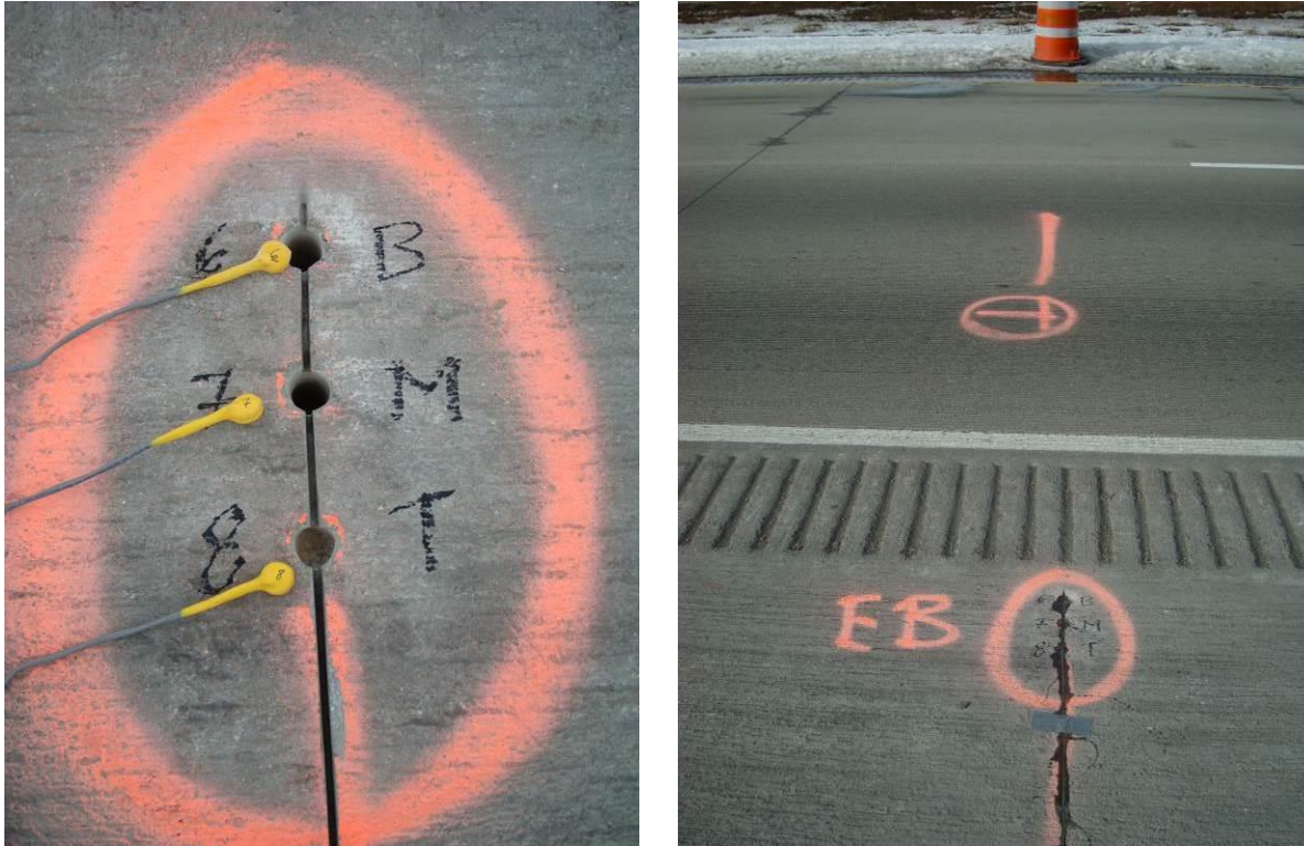
Figure 5. Data logging temperature sensors installed prior to profiling.
