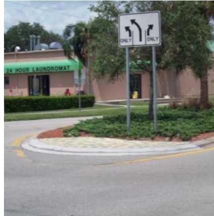
EB median nose at plaza just east of 41st St. SW (after). Nose cut back.
