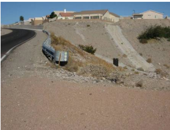
Out-of-date end terminals.
