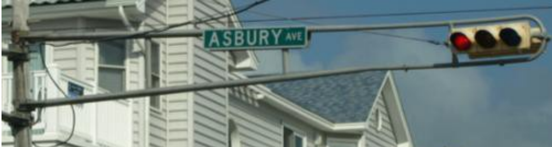
Traffic signal mast arms and signal display alignments prior to improvements.
