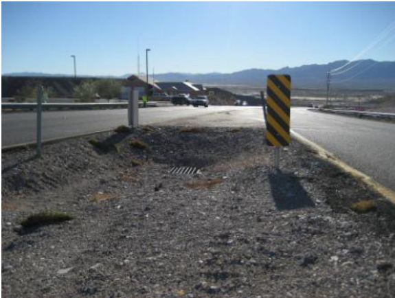
Nontraversable median drains.
