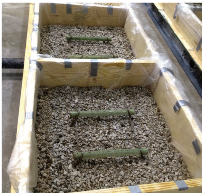
Figure 3.2 Slab molds, lined with plastic, containing 1.25" of gravel base and dowel bars.
