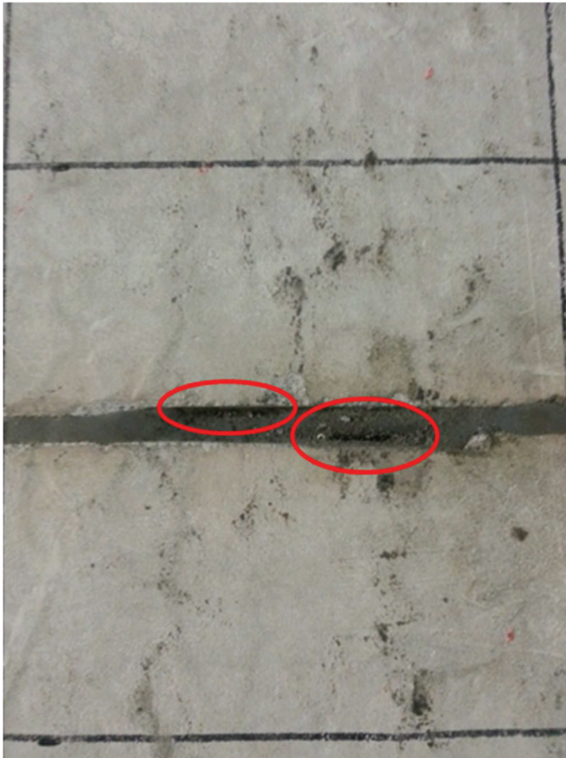
Figure 2.3 Silicone sealant debonding from concrete at the surface of a joint.
