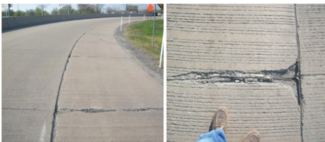
Figure 1.1 Photograph of field observation showing damage in pavement joints.
