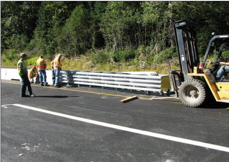
← The fork lift, at the front of the attenuator, uses its fork blade to finish the alignment.
