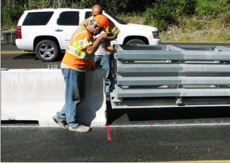
← A workman guides the fork lift operator to correct placement of the crash barrier.
