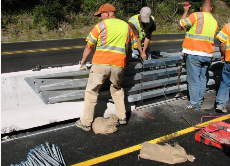
← The transition panel is being positioned for attachment to the jersey barrier and attenuator frame.
