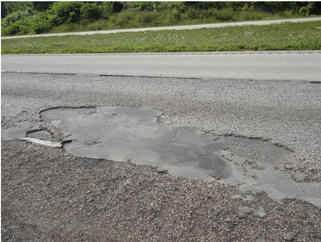
Figure 111. Surface distress at Sta. 664 of WAY-30.
