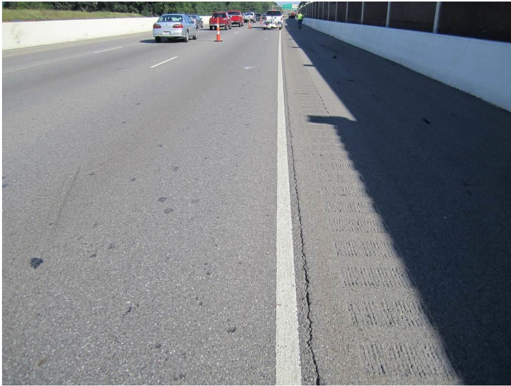
Figure 114. Longitudinal cracks on STA-77.
