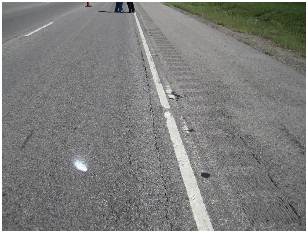
Figure 115. Longitudinal cracks on STA-77.
