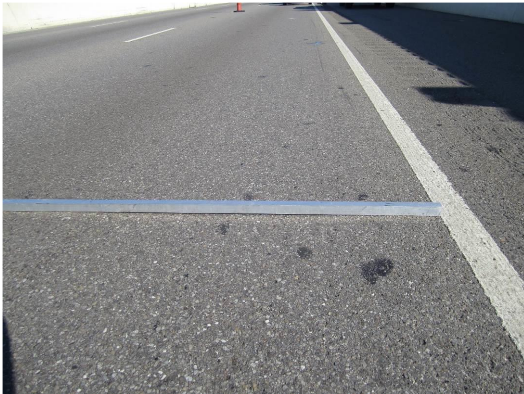
Figure 113. Rutting measurement on STA-77.
