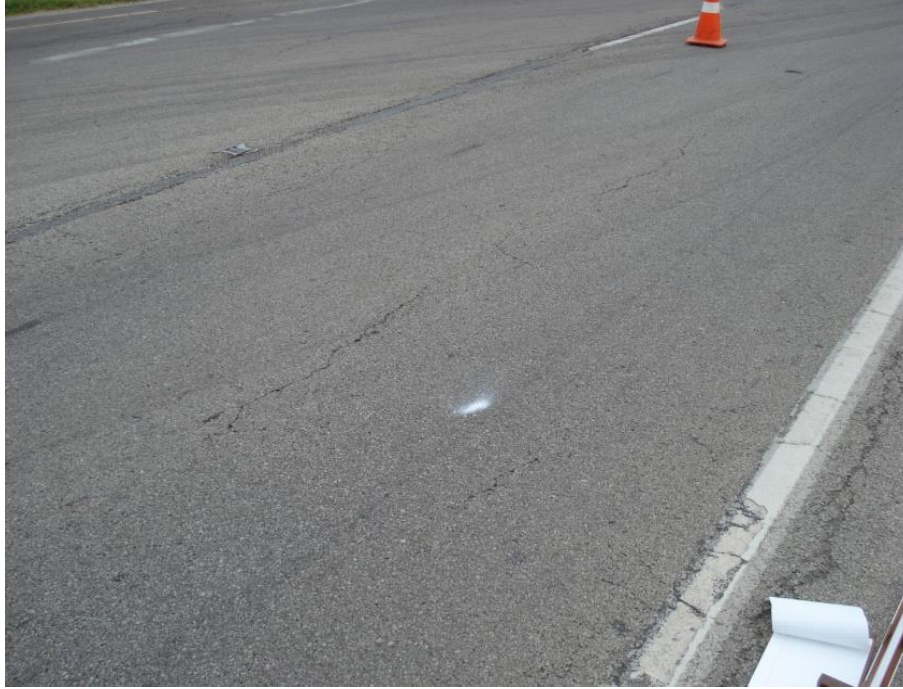
Figure 83. Cracking on PIK 32-15W.
