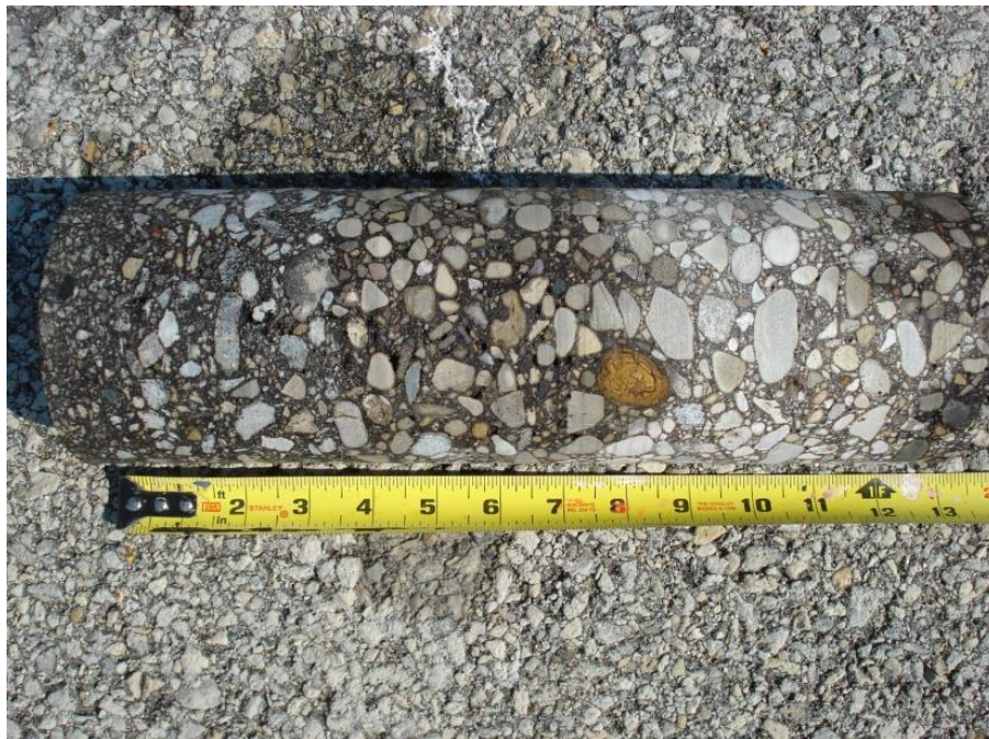
Figure 93. Core sample obtained from an AC pavement. The surface is at the left.
