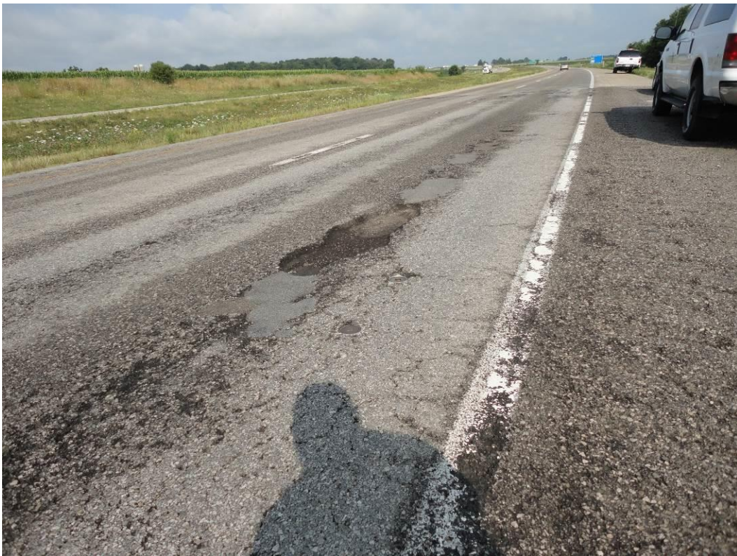
Figure 109. Surface distress at Sta.876 of WAY-30.
