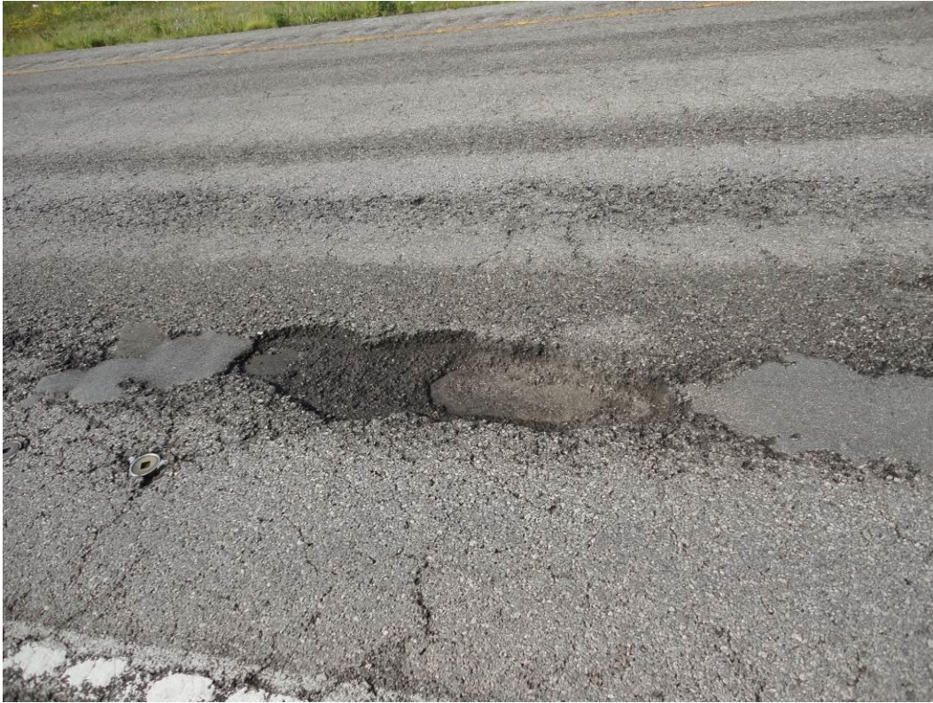
Figure 108. Surface distress at Sta. 876 of WAY-30.
