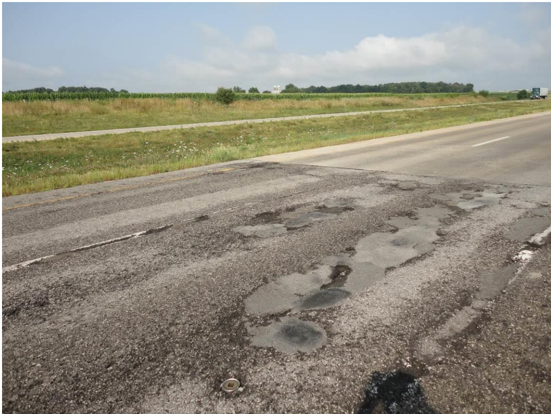
Figure 107. Surface distress at Station 876 of WAY-30, including test section and WIM.
