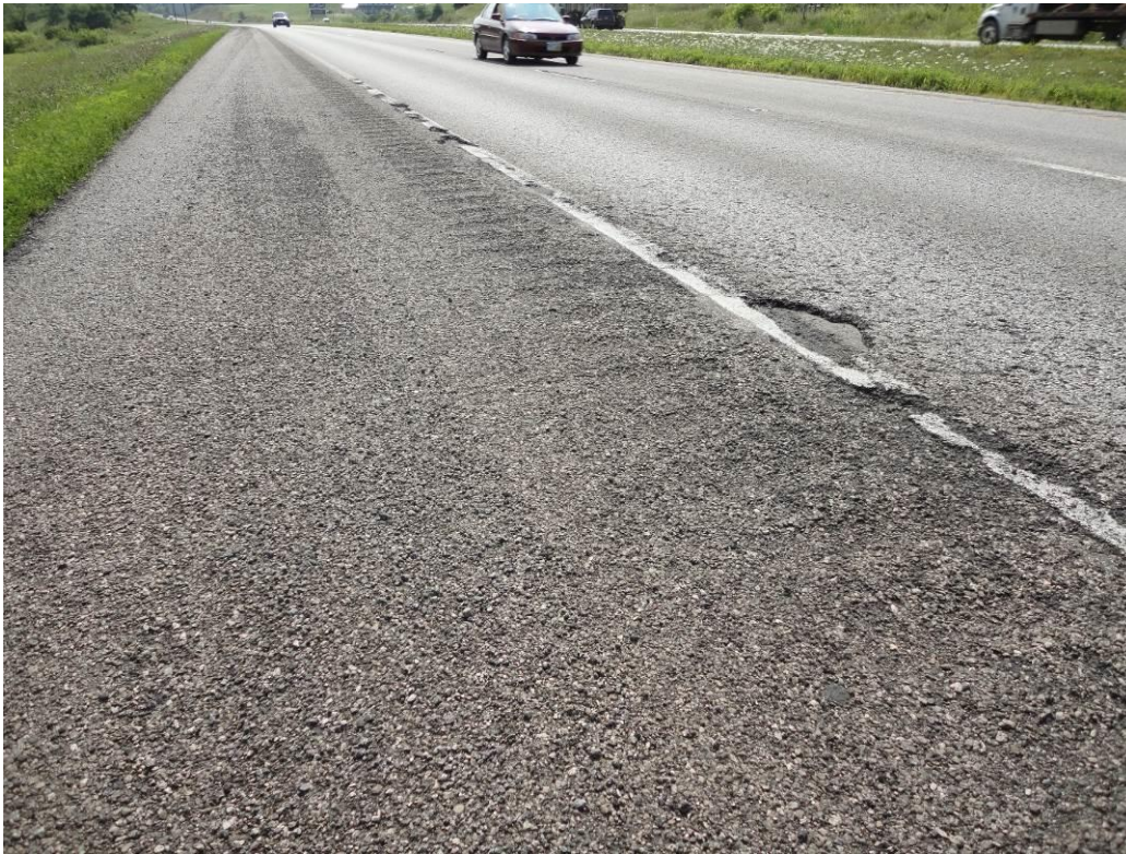
Figure 112. Surface distress at Sta. 664 of WAY-30.
