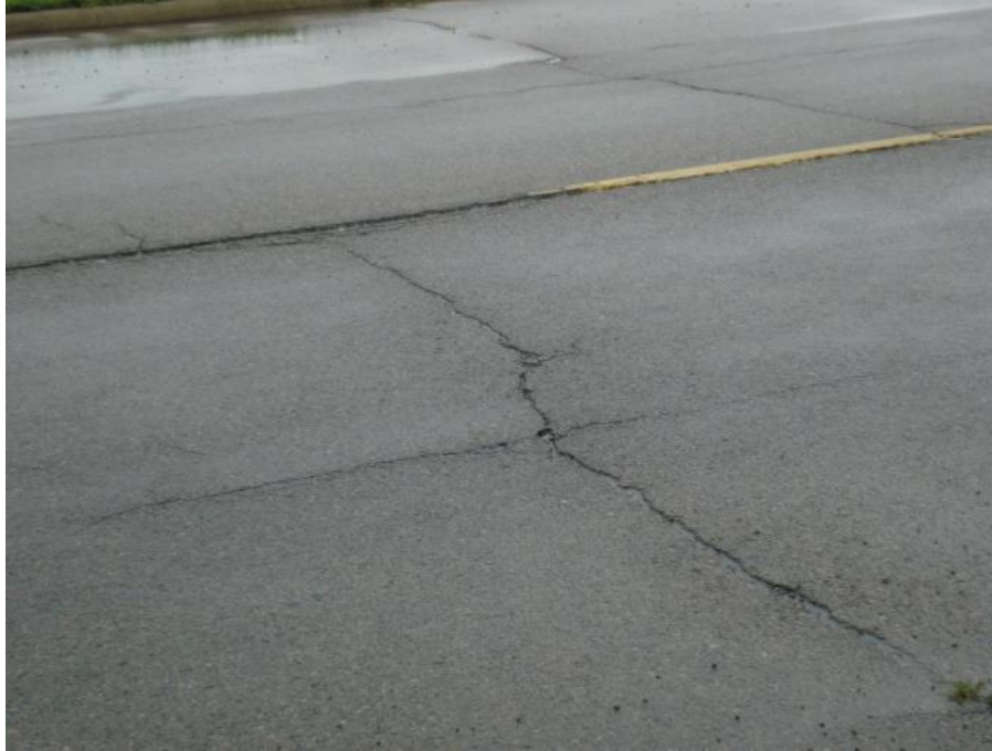
Figure 89. Cracking on CLA 41-3N.
