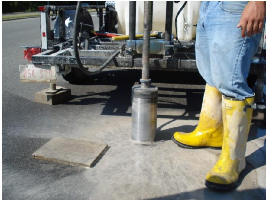
Figure 92. Using a core drill to obtain a sample core of AC pavement.
