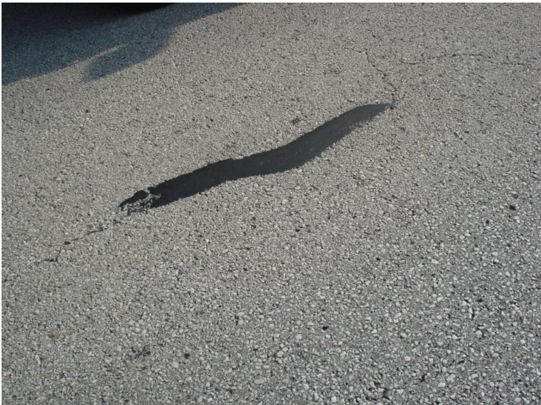
Figure 91. Cracking on BUT 129-22E.
