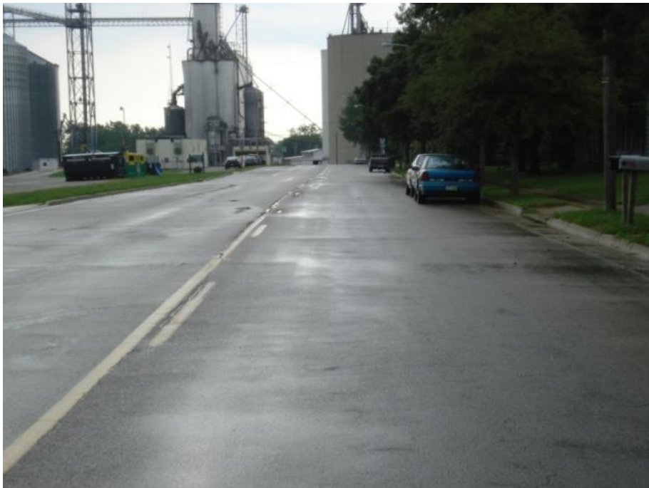
Figure 88. General view of CLA 41-3N.
