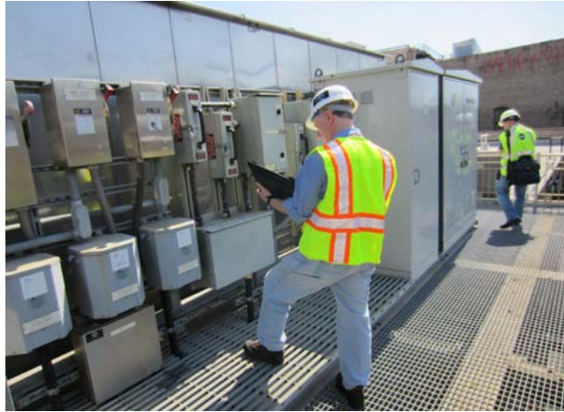
Signal House at Damen Station on Blue Line
