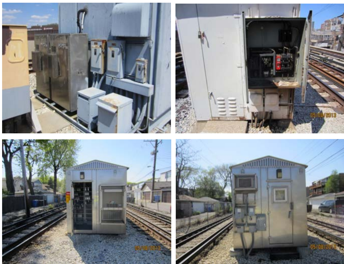
Figure 2-8 Examples of Signal Houses: Orange Line Pulaski Station (top left), Red Line Bryn Mawr Station (top right), Brown Line Rockwell Station (bottom left), Brown Line Sacramento Station (bottom right)
