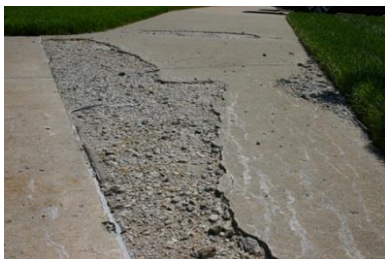
Figure 2.17 Crumbling in concrete (picture from www.greenpiece1.com )
