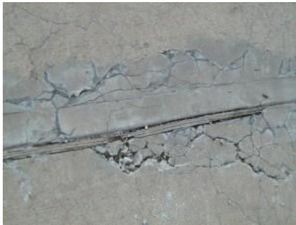
Figure 2.16 D-cracking in concrete pavement (picture from www.civildigital.com )
