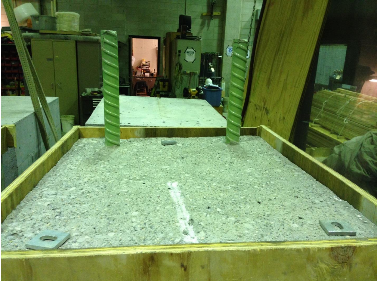
Figure 7. Dam around the top of the bottom specimen to contain the grout for the grout bed
