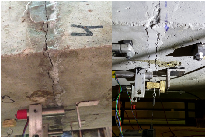
Typical cracks during loading of specimen with standard grout (left) and specimen using UHPC (right)
