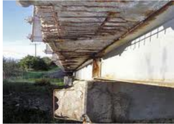
Fig. 1: Corrosion of rebar in a bridge deck overhang
