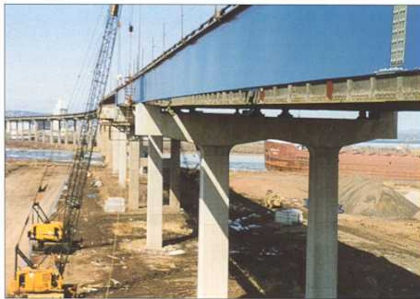
New steel girders are erected as part of Minnesota DOT Blatnik Bridge widening project
