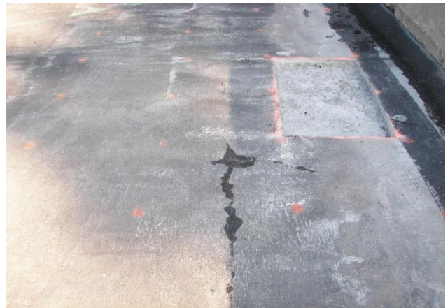
longitudinal cracks at mid deck
