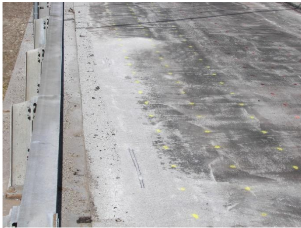
Exposed anode strands in rotted concrete
