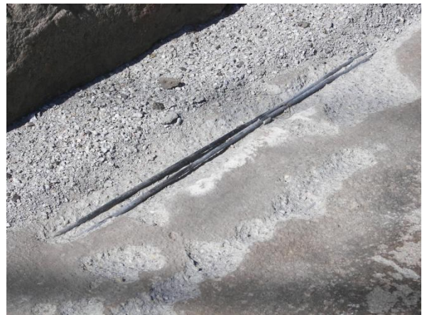
close-up of left photo, poor anode cover
