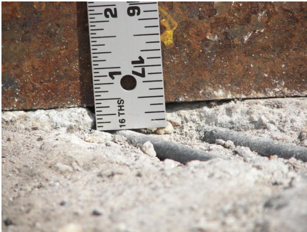
Poor anode strand cover <3/8 inch
