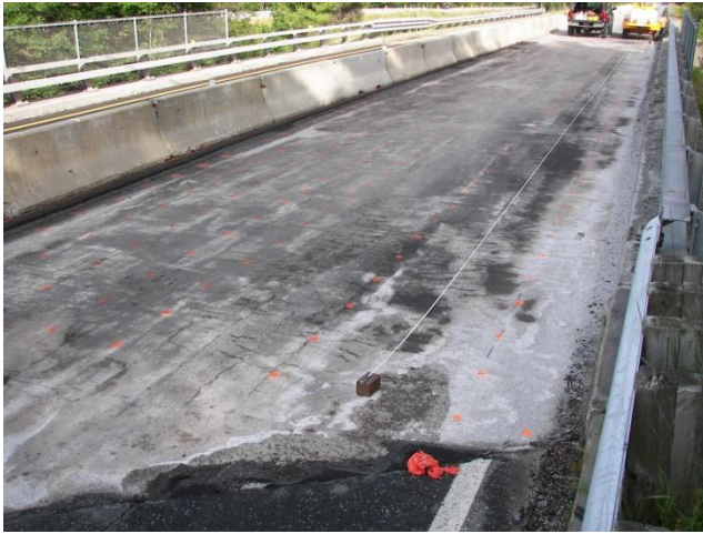
Deck with crack pattern
