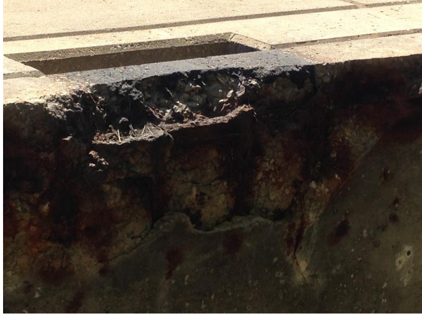
Figure 39. Rebar spacing shown underneath the bridge in corroded section
