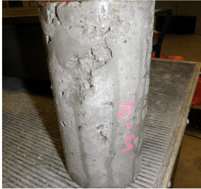
Figure 19. Route 364 paving concrete with surface voids
