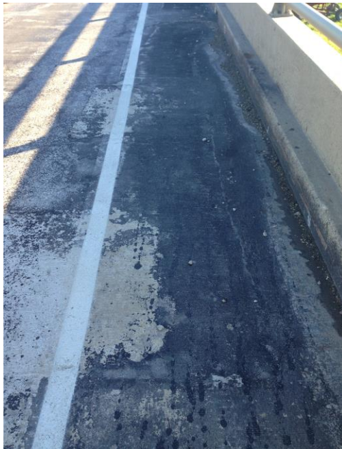
Figure 42. Example of a worn off spot of asphalt emulsion showing concrete underneath
