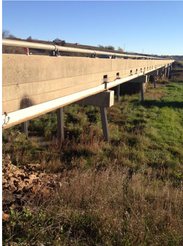
Figure 36. Side view of deteriorating bridge
