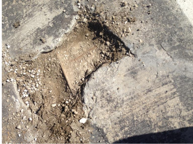
Figure 40. Concrete popout revealing rebar
