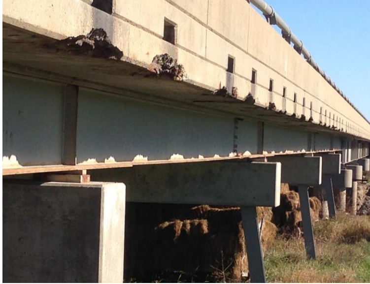
Figure 37. Numerous holes shown corroding throughout the span of the bridge
