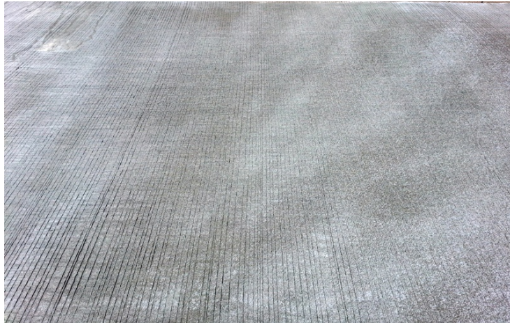
Figure 23 - The water-wax based curing compound applied by the contractor approximately 30 minutes after paving
