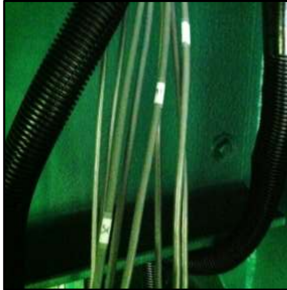
Figure C-4: Photograph of the Installed Labeled Wires
