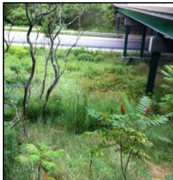
Figure C-2: Photo of Sloped Terrain and Vegetation Growing Around Eastern Abutment at BRB
