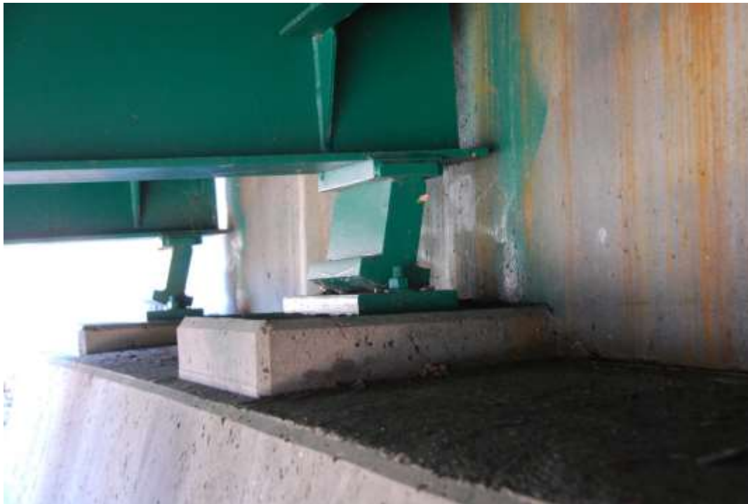
Figure 60: Fully tipped rocker bearings at North Abutment.
