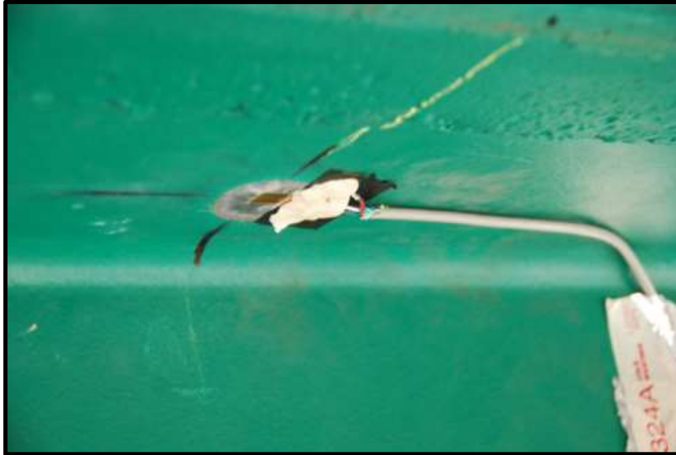
Figure G-3: Photograph of Full Bridge Strain Gauge Installed on the Top Flange of Beam D, South Face
