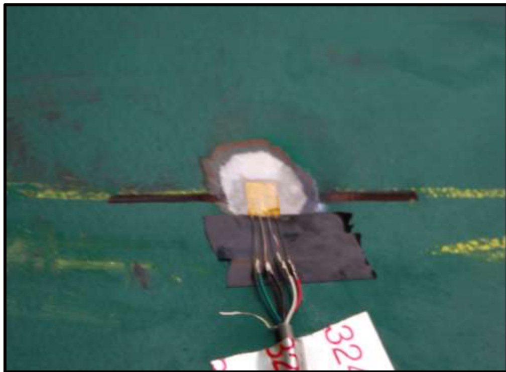
Figure G-8: Photograph of Full Bridge Strain Gauge Installed on the Web of Beam E, North Face
