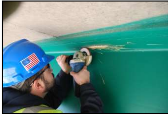
Figure C-7: Photo of the Grinding Step of the Strain Gauge Installation Process at the BRB
