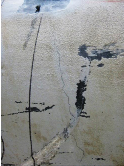
Figure 37: Cracks in Constant Moment Region
