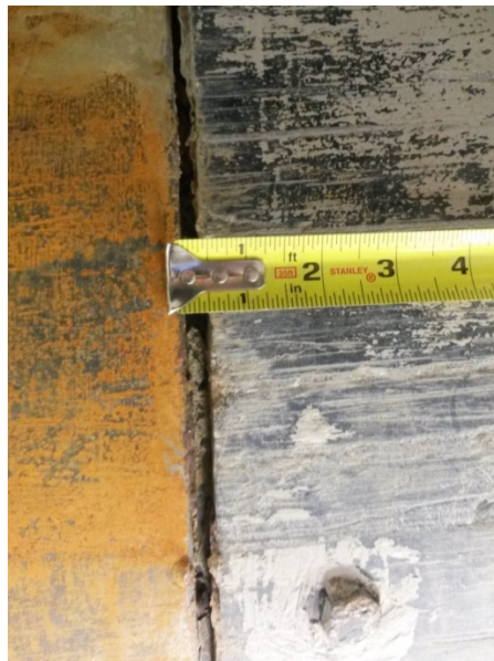
Figure 29: Loss of Composite Action in Pile A
