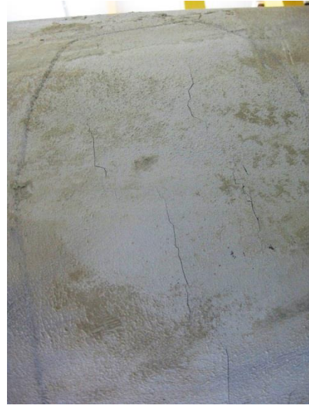
Figure 38: Cracks Out of Constant Moment Region
