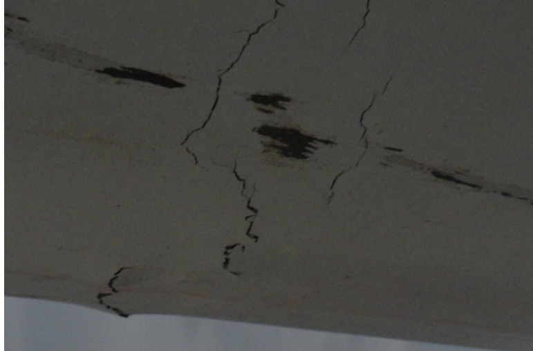
Figure 30: Cracks Due to Cyclic Loading
