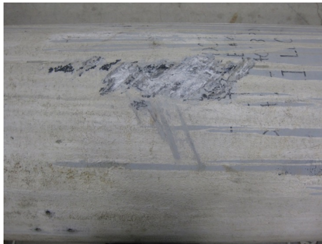
Figure 23: Scrapes at Top of Pile C
