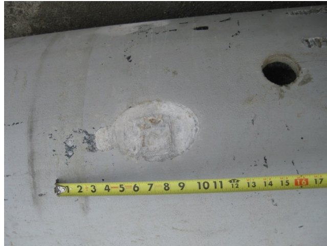
Figure 18: Circular Gouges at Top of Pile B
