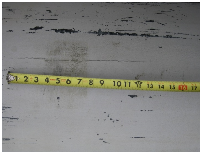
Figure 17: Crack near Tip of Pile B
