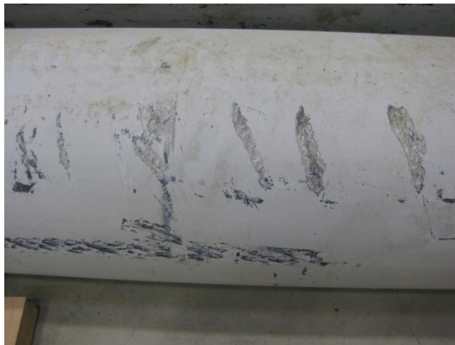
Figure 13: Series of Gouges on Pile A
