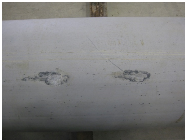
Figure 11: Gouges Near Top of Pile A
