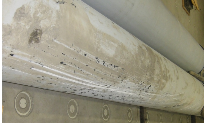
Figure 24: Long Scratches on Pile C
