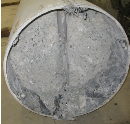
Figure 10: Damage to Top of Pile A
