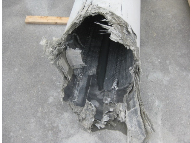
Figure 29: Damage to Bottom of Pile D
