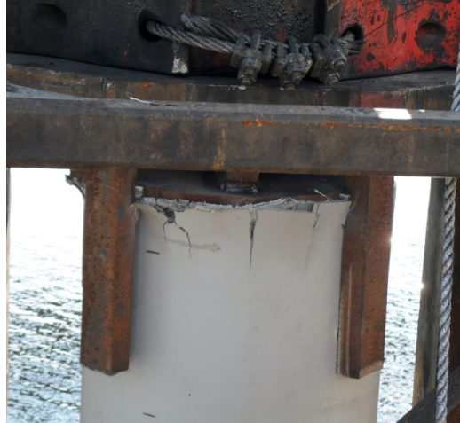
Figure 28: Driving Damage to Pile D
