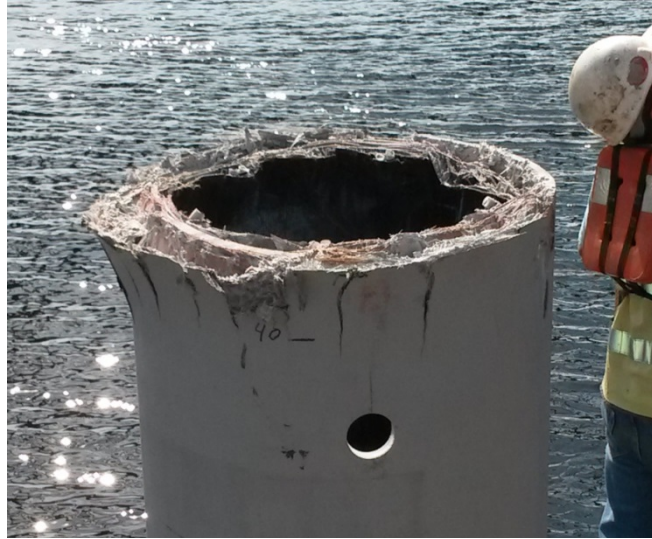
Figure 21: Driving Damage to Pile C
