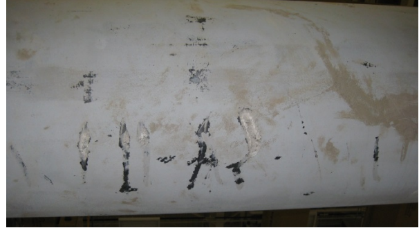
Figure 27: Series of Gouges on Pile C
