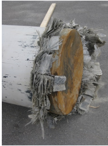
Figure 16: Damage at Tip of Pile B
