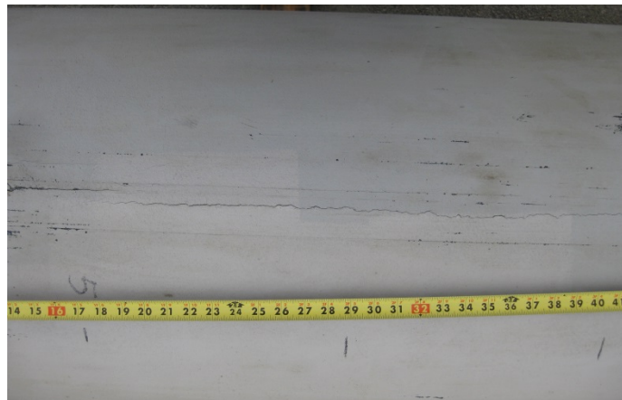
Figure 30: Longitudinal Cracking at Bottom of Pile D
