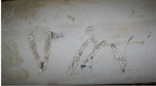
Figure 26: Series of Gouges on Pile C
