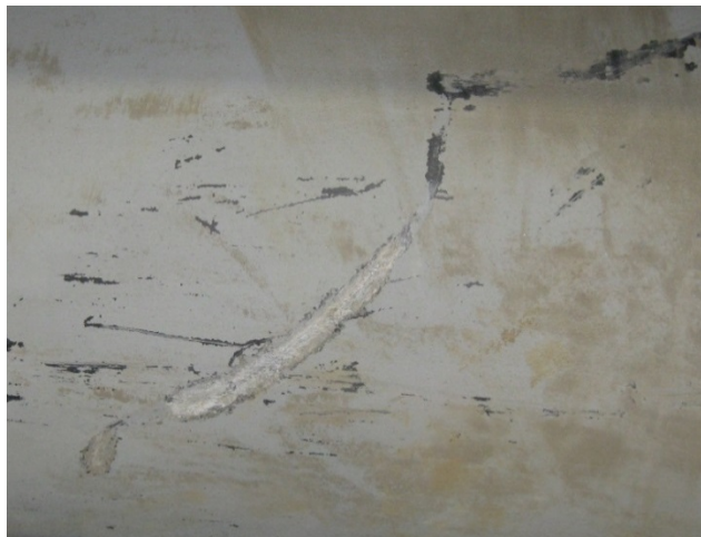
Figure 25: Gouge on Pile C
