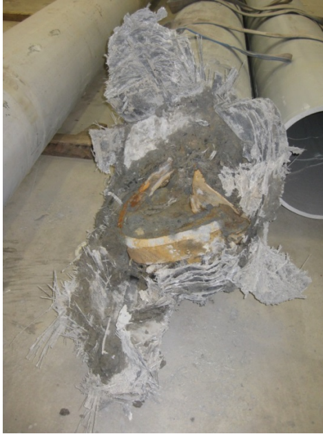
Figure 22: Damage to Bottom of Pile C
