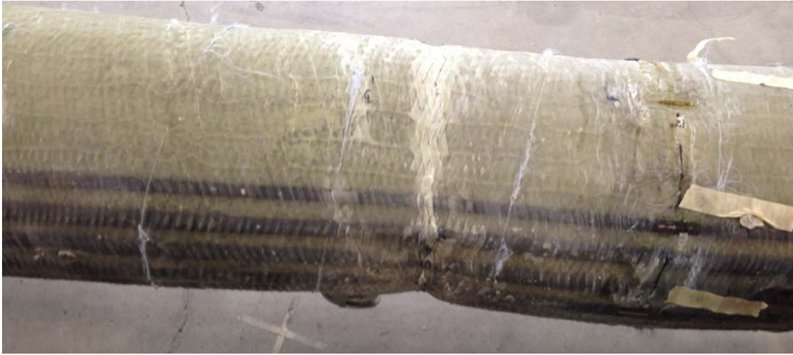
Figure 23 – Top of arch near midspan due to void in concrete
