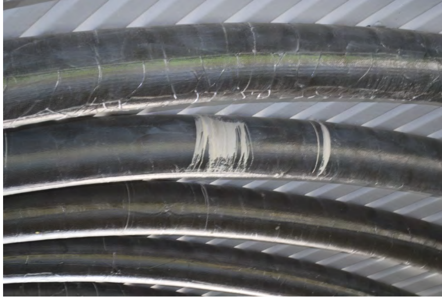
Figure 31: Concrete leakage near crown
