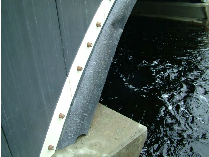
Figure 36- Damaged outside arch (2011)
