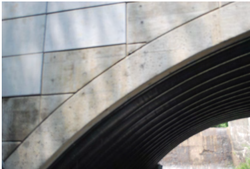
Figure 35: Concrete discoloration between T-Wall and CIP concrete
