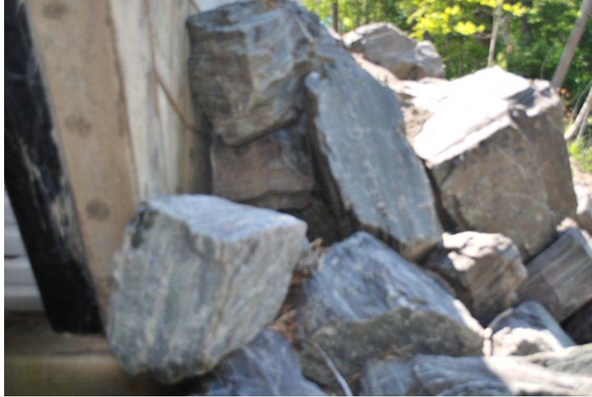
Figure 34: Debris in heavy rip rap indicating high water mark above base of tubes
