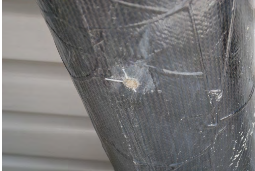
Figure 30: Plugged hole in tube
