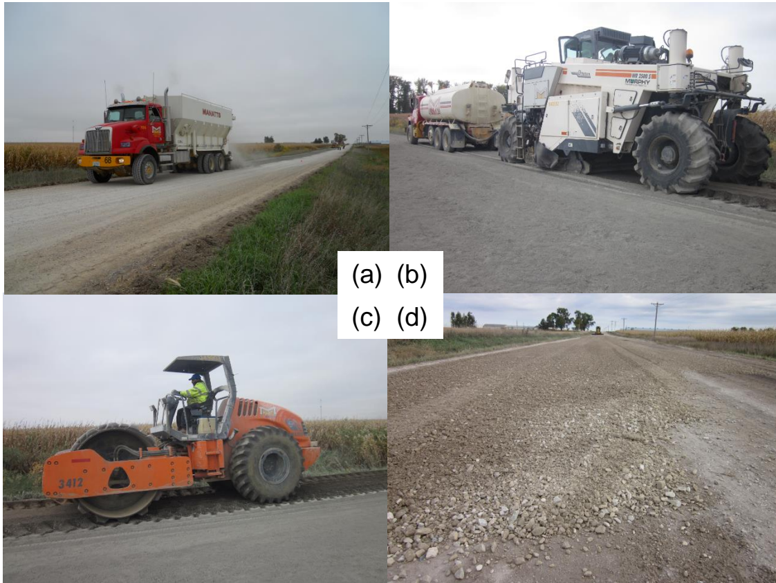
Figure 40. Construction procedures and equipment for chemically stabilized Sections 15, 16, and 17: (a) powder truck for spreading bentonite, fly ash, and cement, (b) full depth reclaimer connected to water truck milling chemical stabilizers to the specified depth and water content, (c) vibratory pad-foot roller following the full depth reclaimer, and (d) 1 in.-thick road-stone wearing surface
