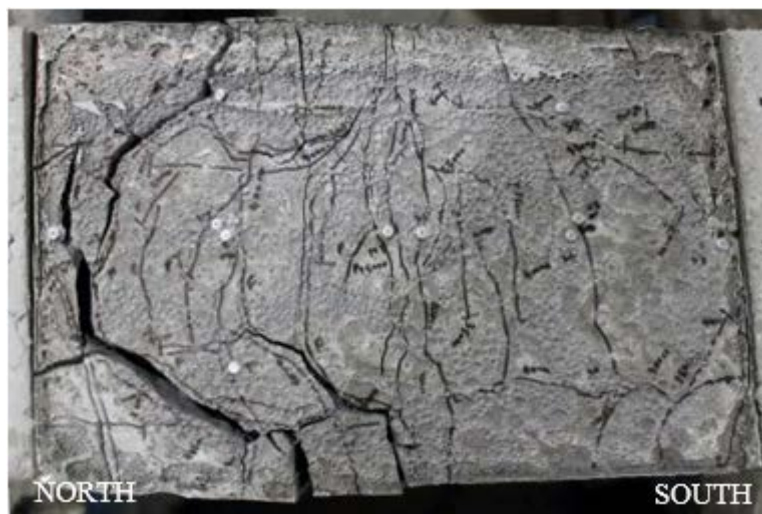
Figure 52. Top of the UHPC Pocket in Specimen U-6-7-I After Failure
