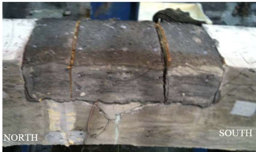
Figure 41. VHPC Pocket in Specimen V-4-4-I at End of Load Application Showing Interface Separation
