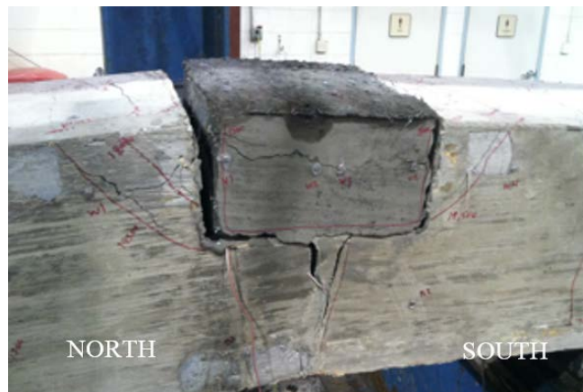
Figure 39. VHPC Pocket in Specimen V-4-4-II Showing Interface Separation and Splitting Cracks
