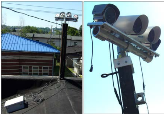
Figure 2: WISESight™ prototype on IEM rooftop
