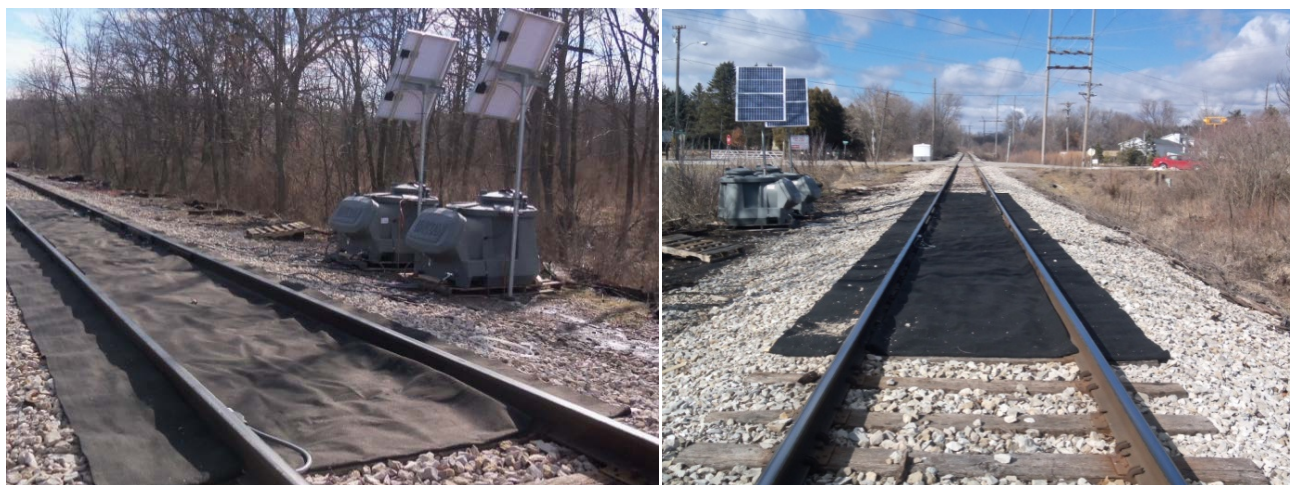
Figure 15: The two new lubricators from the OEM were installed at the Cedar Rapids site
