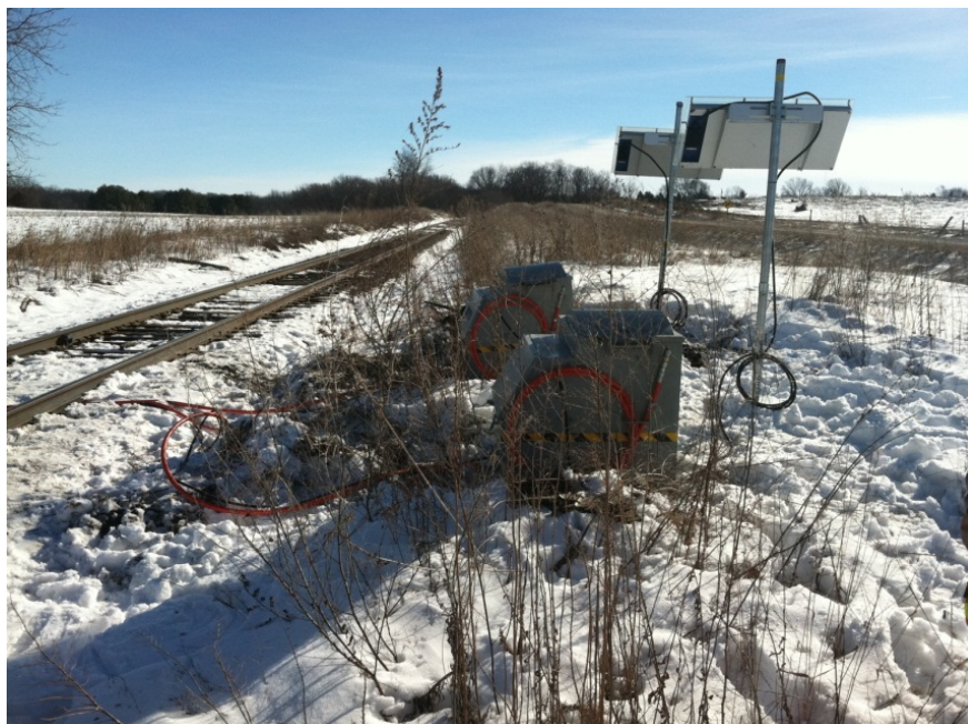
Figure 14: The two refurbished lubricators were installed on the Cedar Falls test site; each lubricator had its bars on a different side of the track
