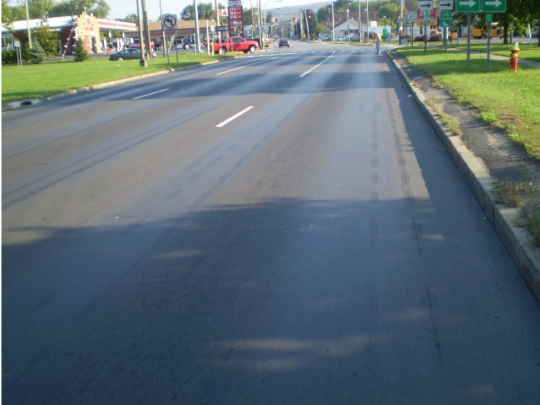
Figure 3 - Flushing at Intersection of Rt 921C (< 30 Million ESAL's)
