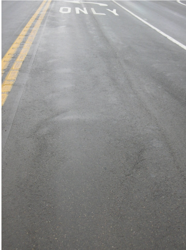
Figure 57 – Slippage Cracking in Dedicated Left Turn Lane in Region 3 (Rt 96B)
