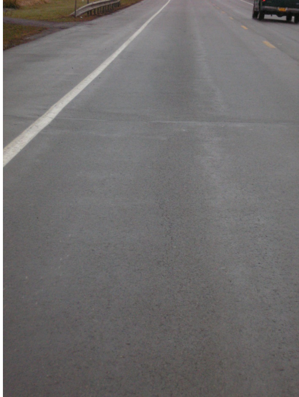
Figure 56 – “Wash-boarding” of 9.5 mm Surface Course in Region 3 (Rt 96B)
