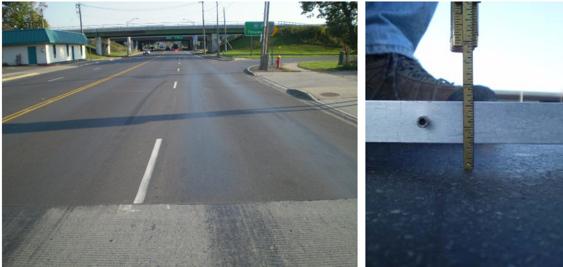
Figure 5 – Flushing and Rutting Located on Rt 921C, Utica, NY
