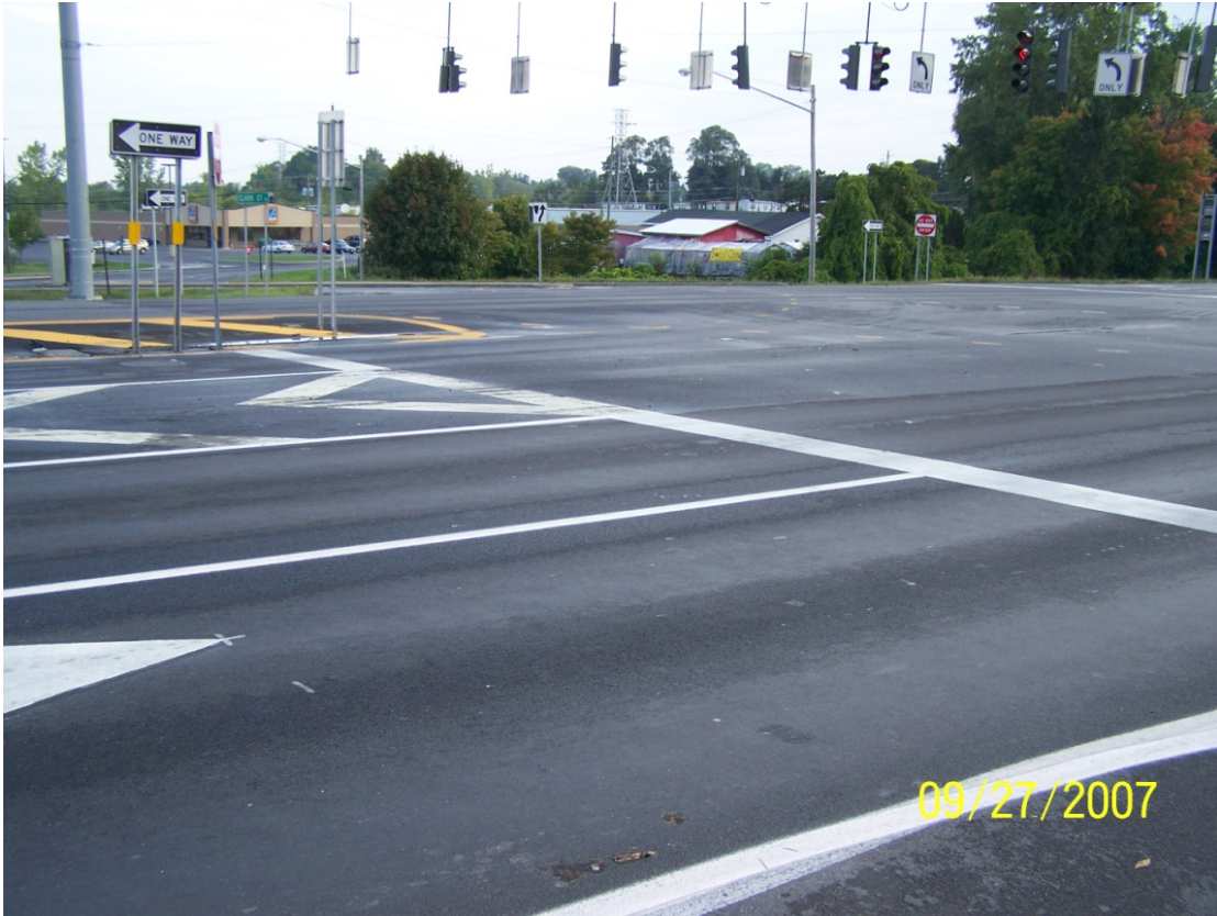
Figure 4 - Flushing at Intersection of Rt 5 (< 30 Million ESAL's)
