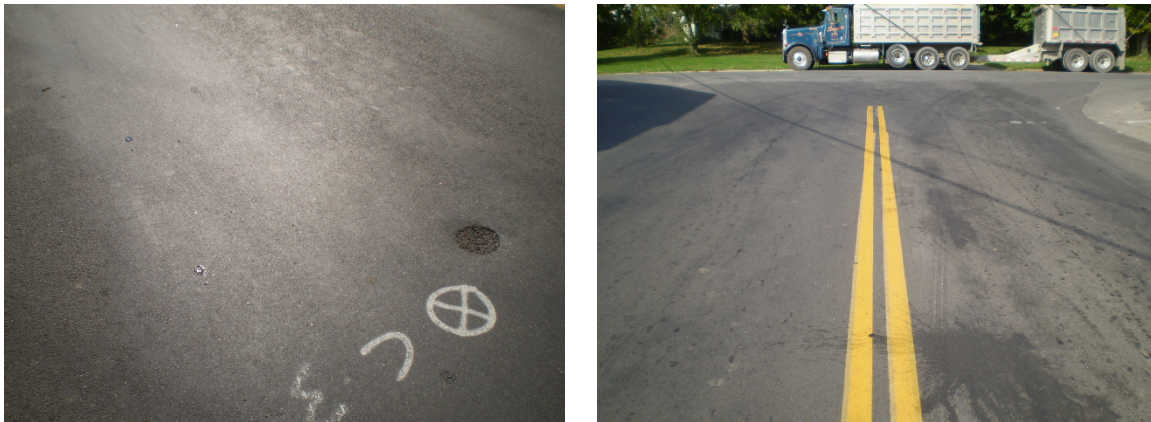
Figure 8 – Flushing at the Intersection of Rt 315 in Deansboro, NY (Region 2)
