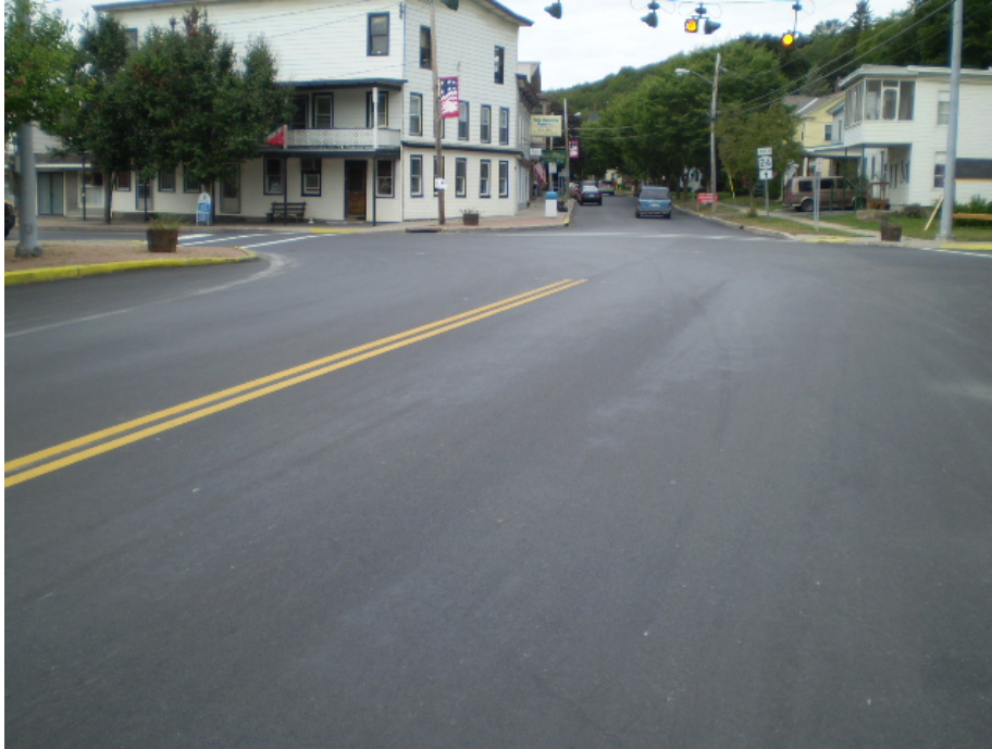
Figure 9 – Flushing at the Rt 12B Intersection in Oriskany Falls, NY
