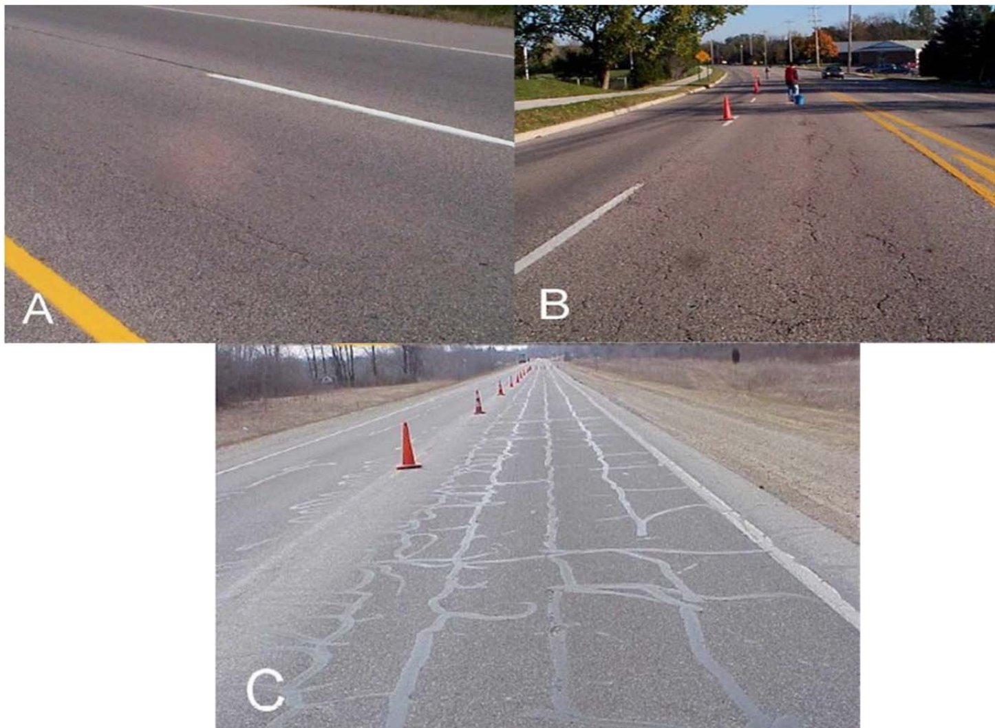
Figure 2.3: Photographs Illustrating the Development of Top-Down Cracking (Svasdisant et al. , 2002)
