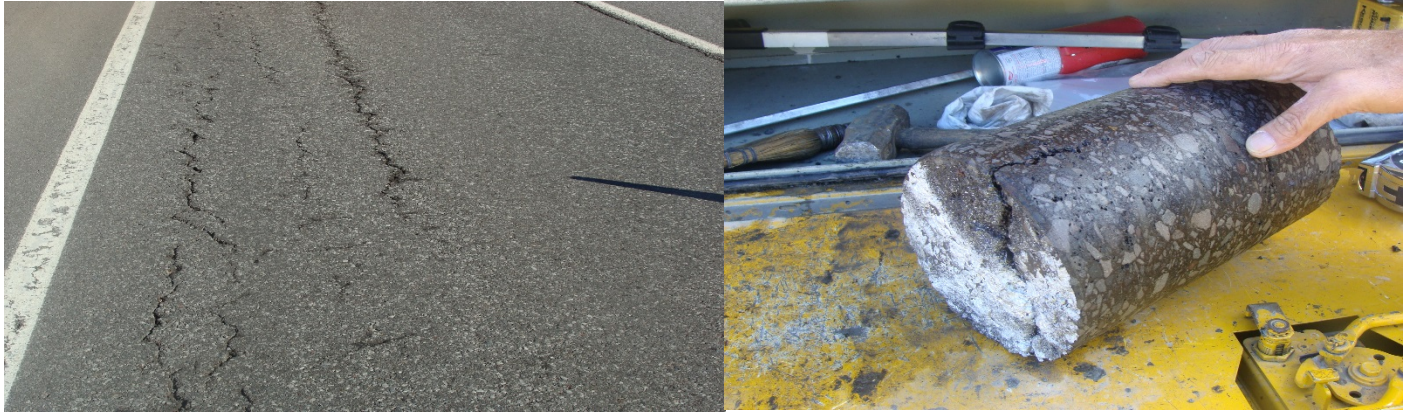
Figure 1.1: Pictures Showing the Development of Top-Down Cracking
