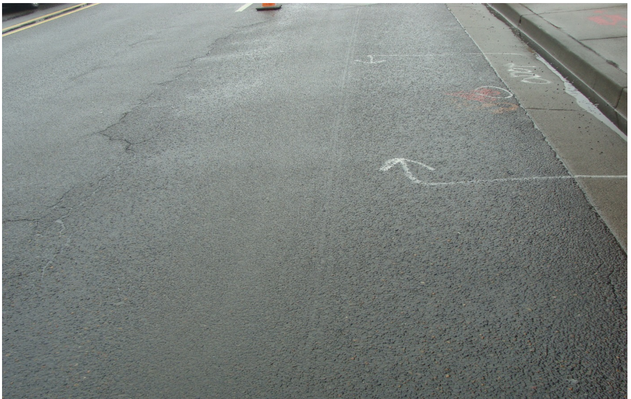
Figure 4.3: Tow-Down Cracking on Section OR99*-C
