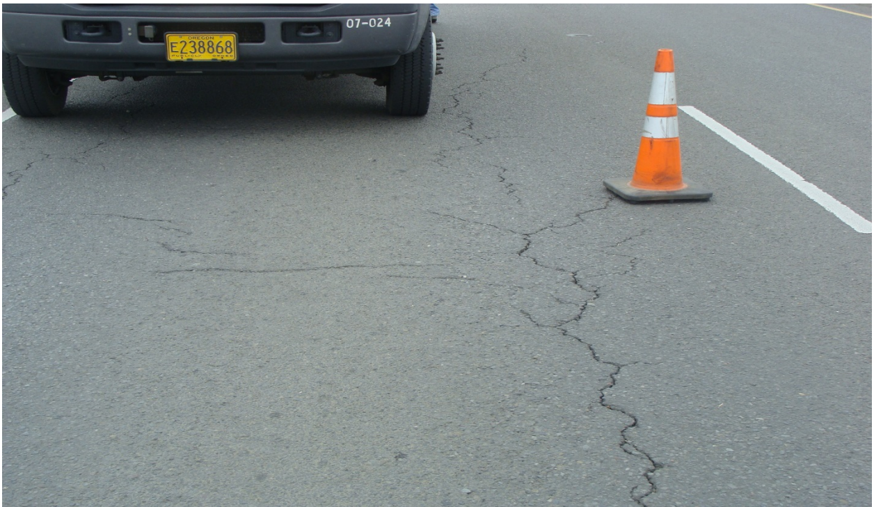
Figure 4.1: Top-Down and Transverse Cracking on Section OR238-C
