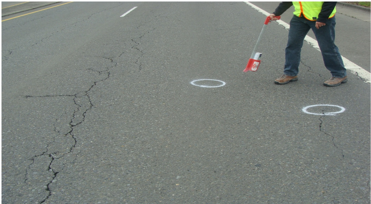
Figure 4.2: Top-Down Cracking on Section OR221-C
