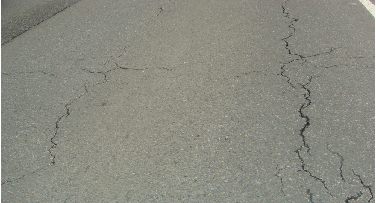
Figure 4.4: Top-Down and Transverse Cracking on Section OR99EB-C
