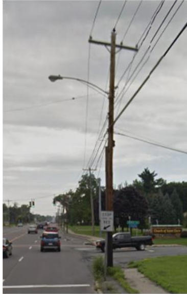
Figure 3. Luminaire type used to illuminate the Central Avenue section.
