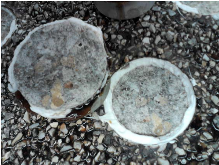
Figure 2.1: Failures in the Concrete
