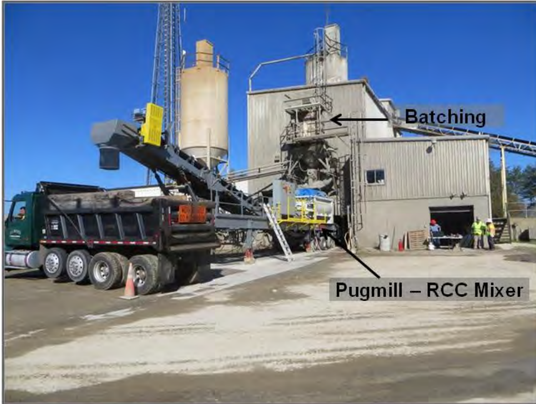
Figure 4. RCC Production Plant With Pugmill Attachment
