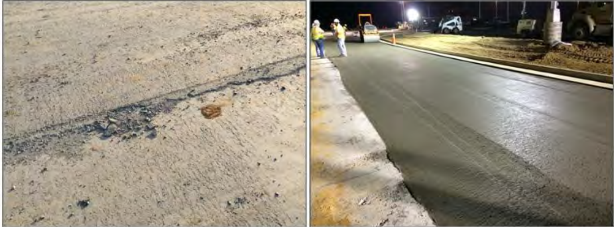
Figure 12. Uneven Longitudinal Joints and Raveling
