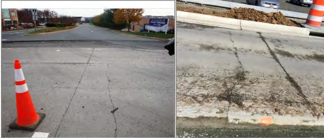
Figure 16. Transverse Cracks on Staffordboro Boulevard (left: northbound; right: southbound)
