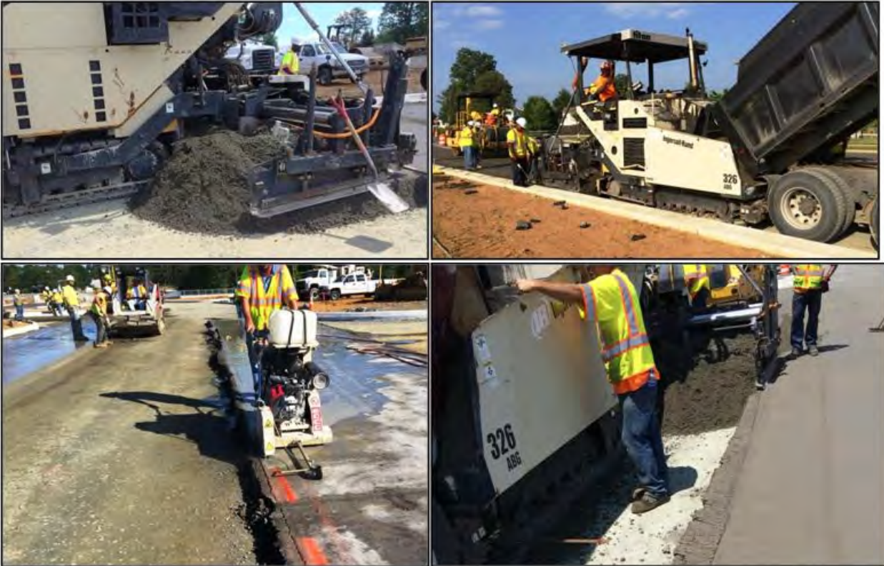
Figure 9. Paver Operation of 12- to 17-ft-Wide Placement; Preparation for Fresh and Cold Joints
