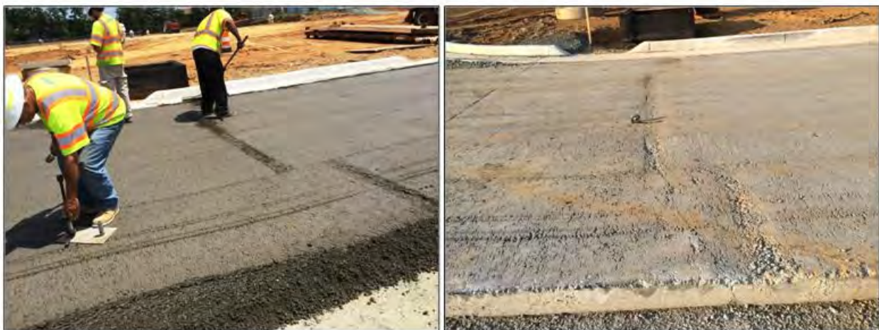
Figure 11. Cracks and Dips Attributable to Stop-and-Go Paving Operations
