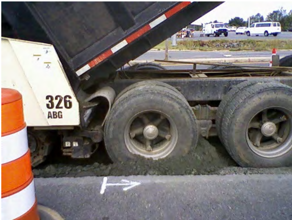
Figure 7. Settlement of Unstabilized Base During Paving
