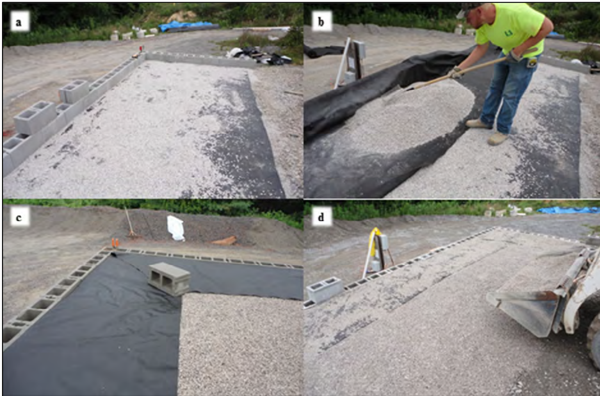
Figure 11. Placing the Protective Wrap. (a) Thin Layer of Aggregate Placed Over Primary Reinforcement; (b) Placing Protective-Wrap Geotextile and Fill; (c) Fill Compacted and Wrap Completed; (d) Thin Layer of Aggregate Placed Over Protective-Wrap Geotextile, Prior to Placement of Next Level of Primary Reinforcement
