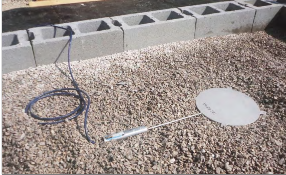
Figure 22. Example of Earth Pressure Cell in Level 1 Fill
