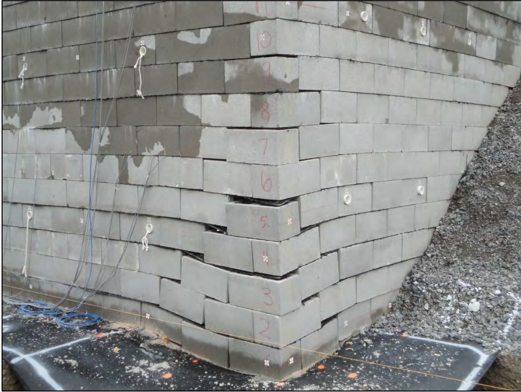
Figure 27. Corner a of Abutment After Test A1
