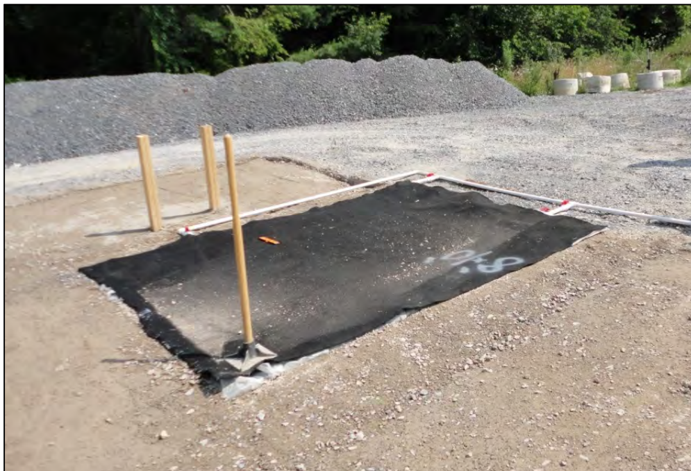
Figure 9. Fill Compacted Around Geofoam on Side b, Solvent Delivery System in Place, and Foam Covered With Protective Non-Woven Geotextile
