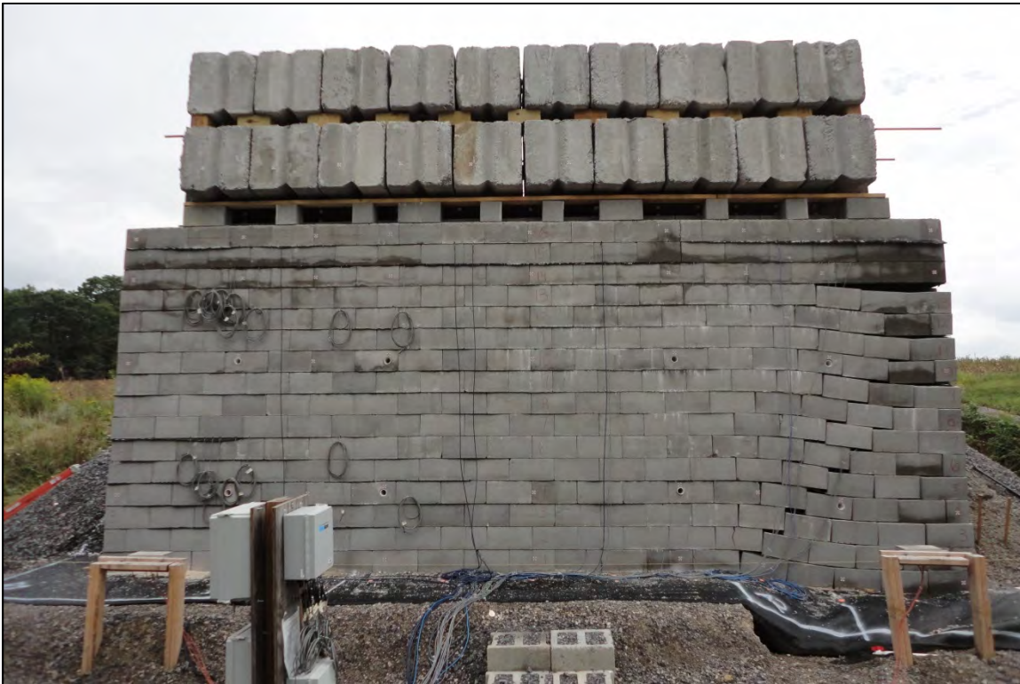
Figure 28. Front View of Abutment After Test A2
