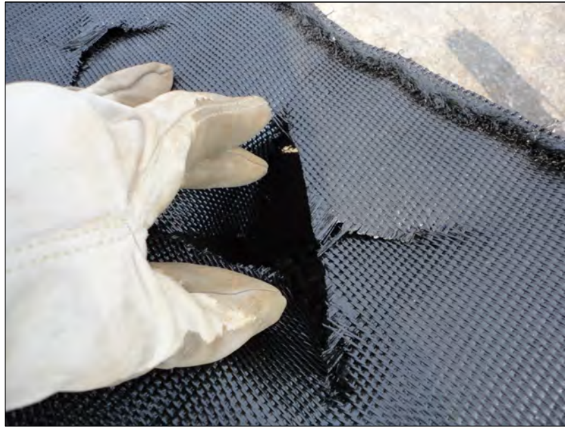
Figure 13. “X”-Shaped Slit in Reinforcement at Level 15
