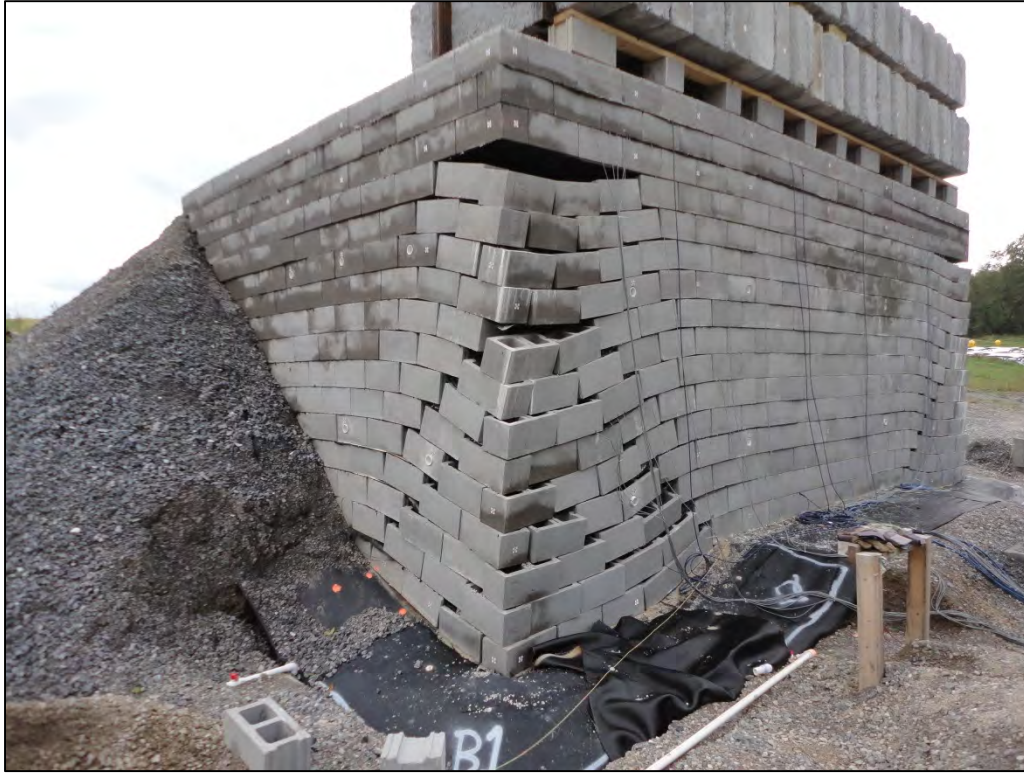
Figure 33. Corner B of Abutment After Test B2
