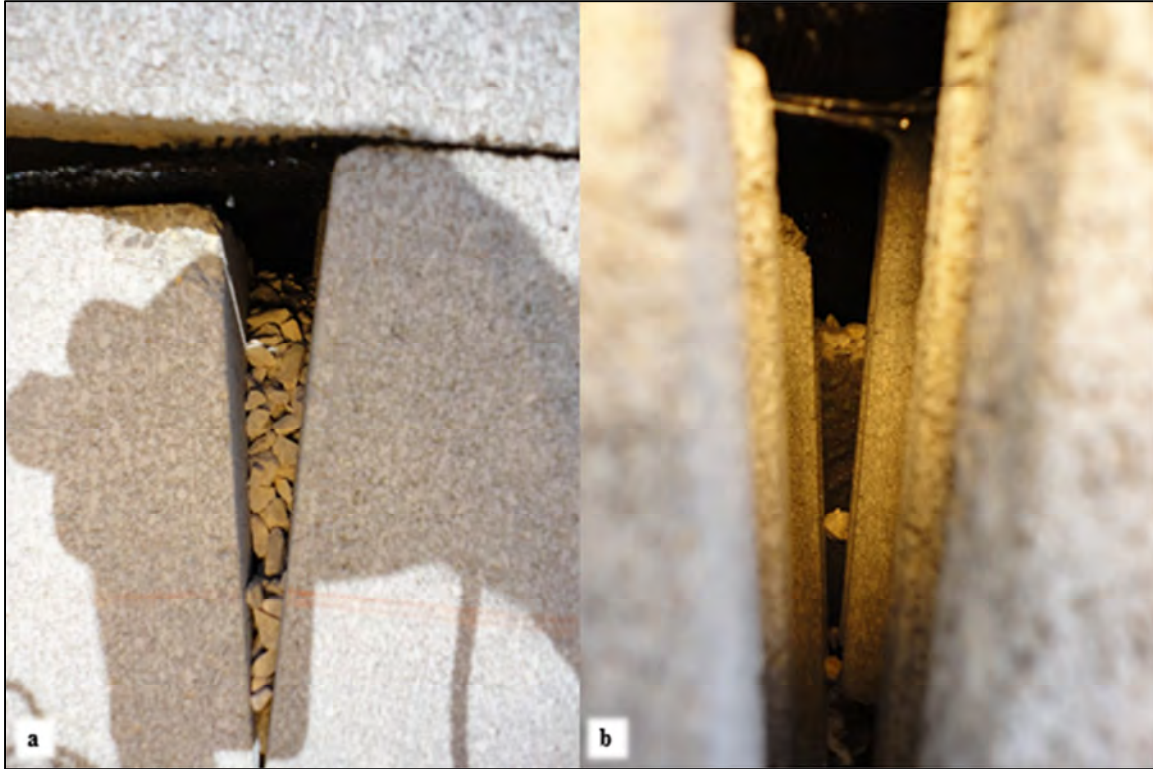
Figure 100. Second Comparison of Unwrapped and Wrapped Fill. (a) Unwrapped Fill at Wing Wall A, Level 5 Near Corner A; (b) Wrapped Fill at Level 6, Above and to the Left of the Vertical Gap in (a).
