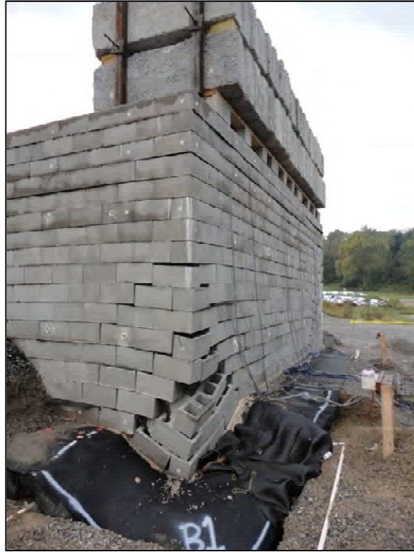
Figure 31. Corner B of Abutment After Test B1
