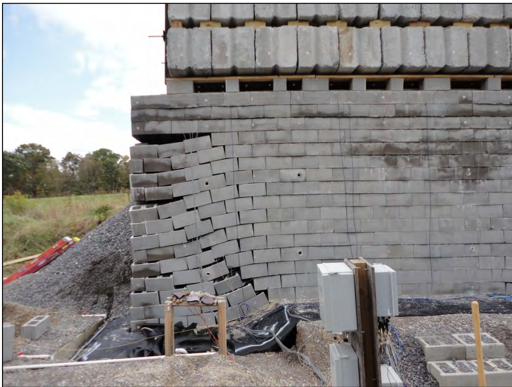
Figure 32. Front View of Abutment After Test B2
