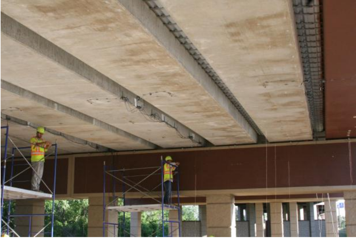
(a) Instrumentation Installation Underneath the Bridge
