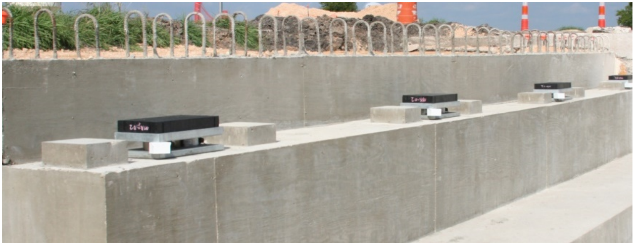
(b) North End Load Cell Assembly
