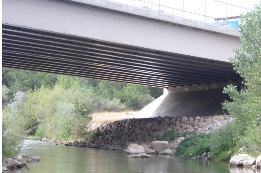
Figure 2-3: Riprap Used to Protect a Bridge Abutment. Flow from Left to Right (Photo by Evan Cope).
