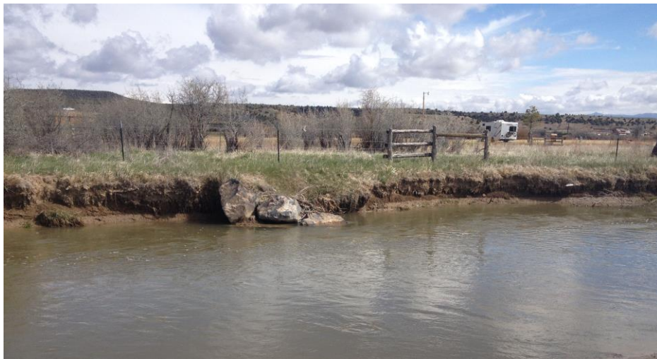
Figure 3-5: Large Vane Angle that Created a Recirculating Eddy and has Actually Increased Streambank Erosion. Flow from Right to Left. (Photo by Evan Cope).
