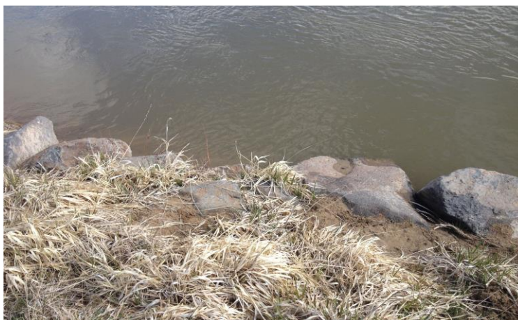
Figure 3-7: Tight Vane Angle Protected and Stabilized the Streambank. Flow from Right to Left (Photo by Evan Cope).
