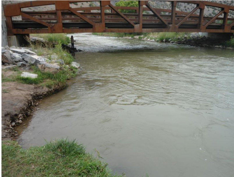
Figure 2-4: Abrupt Change from Riprap to Streambank, Causing Downstream Scour. Flow from Top to Bottom (Photo by Evan Cope).
