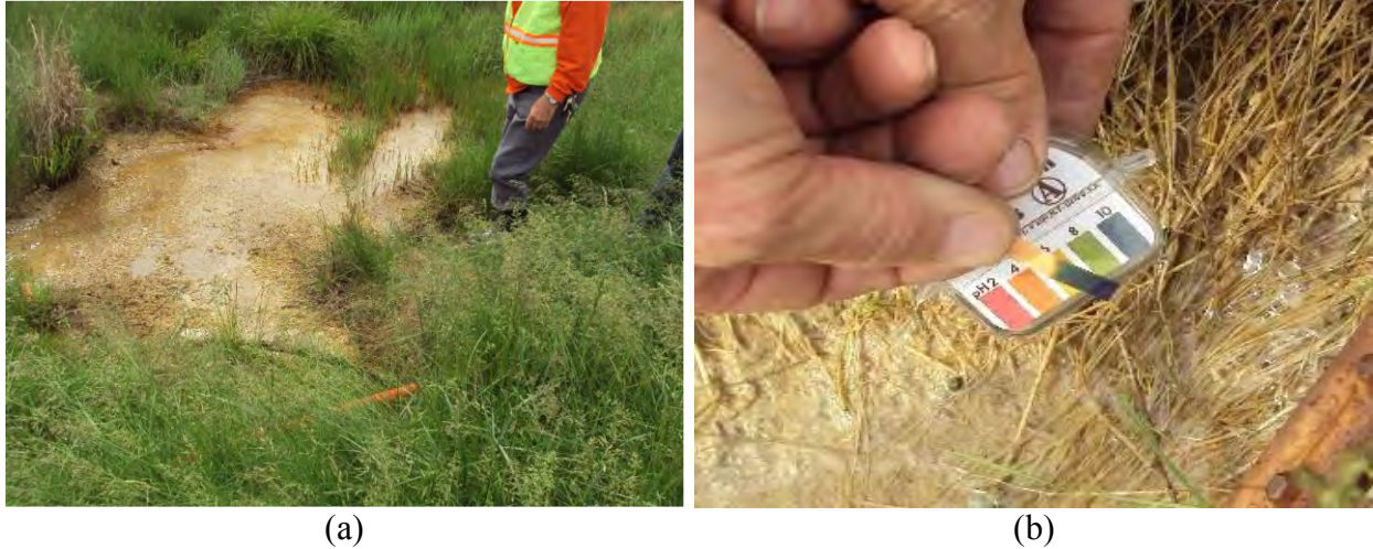
Figure 11. Vegetation condition in the vicinity of drain outlets carrying tufa materials (I-35/N/MP141.30): (a) vegetation kill (dead zone), (b) water from the drainage outlet pipe showing a pH value of 10
