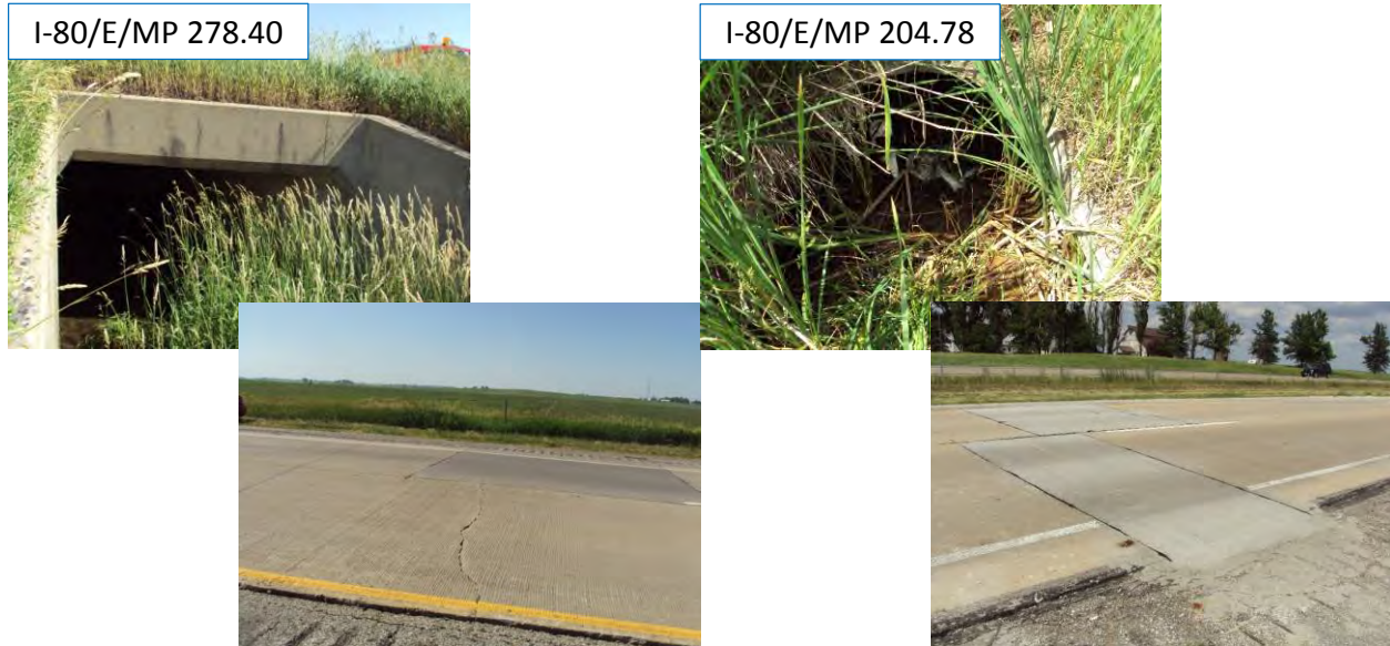
Figure 17. Cracking/patching observed near culvert-only/culvert with drainage outlet locations in newly constructed JPCP sites
