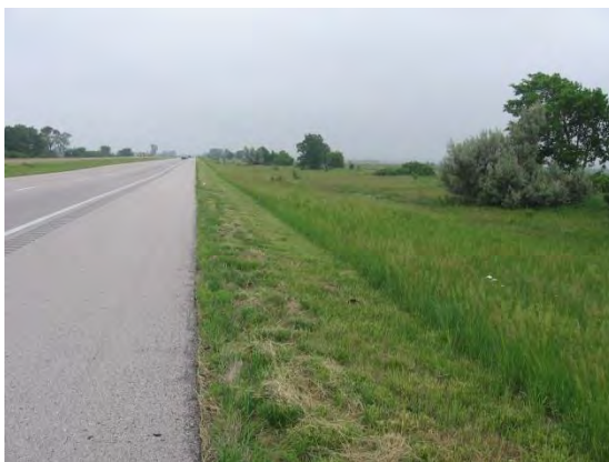
No drainage outlet
