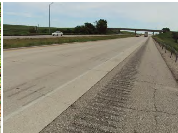
Transverse cracking due to culvert
