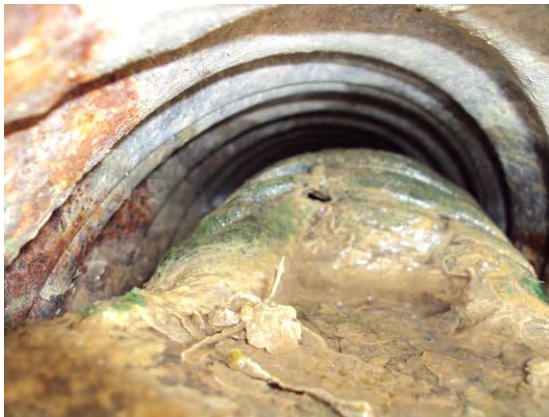
Tufa blockage extends back into the pipe
