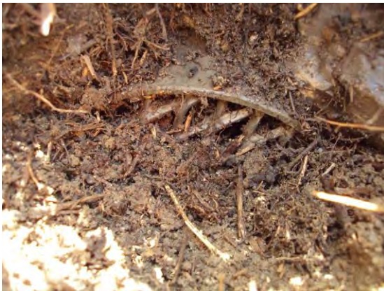
Had to dig to find drain
