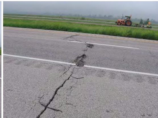
Transverse and alligator cracking
