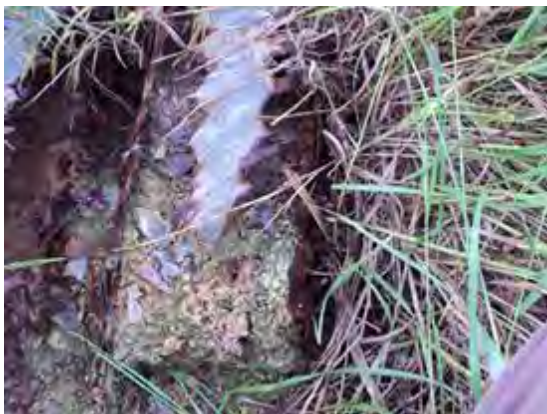
Tufa blockage/damaged outlet pipe
