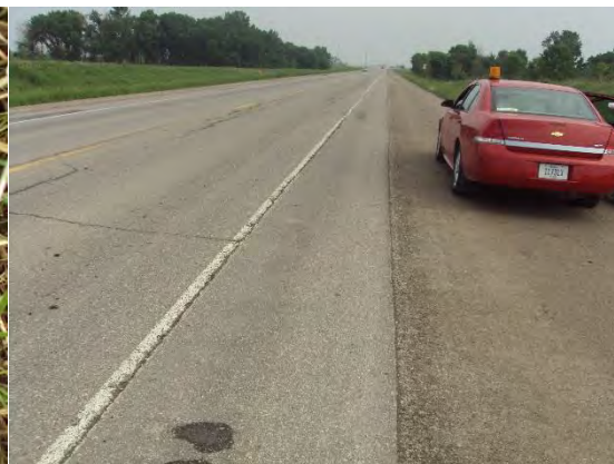
Longitudinal and reflection cracking
