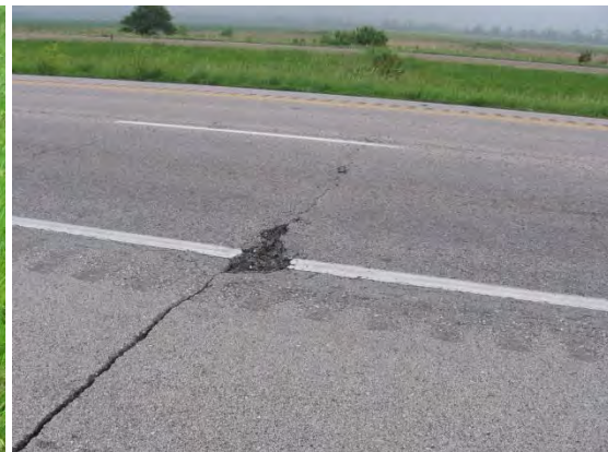
Transverse and alligator cracking
