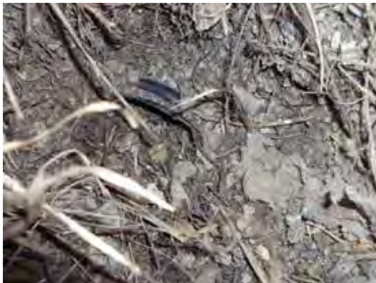
Soil blockage/damaged outlet pipe
