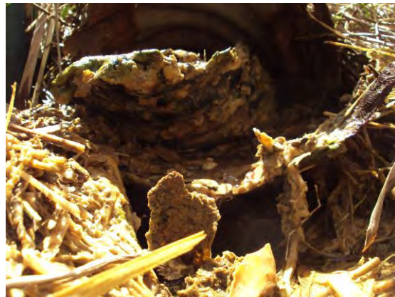
Damaged and tufa formation at outlet
