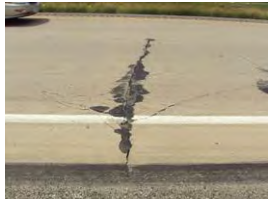
Longitudinal and transverse cracking
