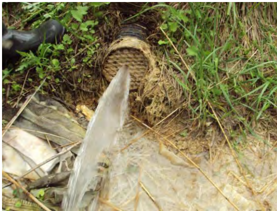
Water backup in pipe
