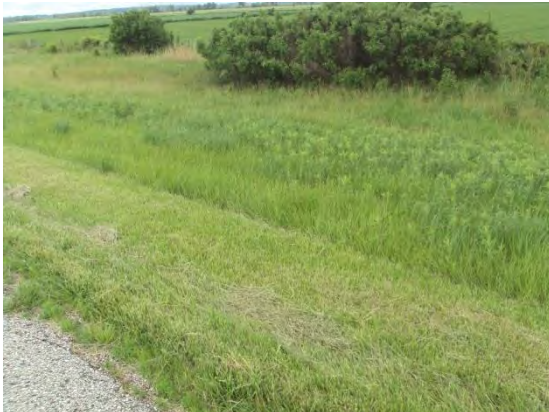
No drainage outlet
