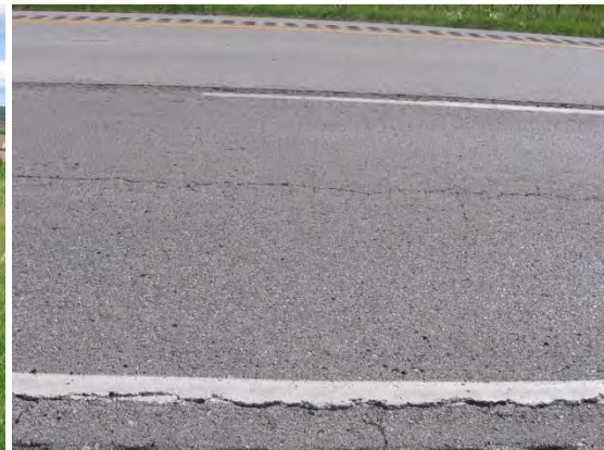
Alligator and transverse cracking
