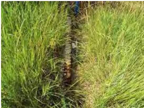
Tufa blockage and damage
