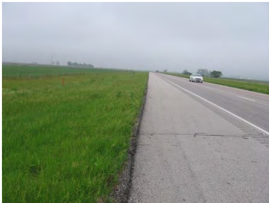
No drainage outlet
