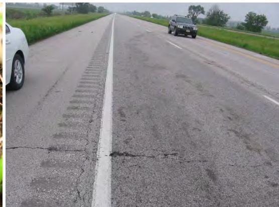
Longitudinal and transverse cracking/rutting
