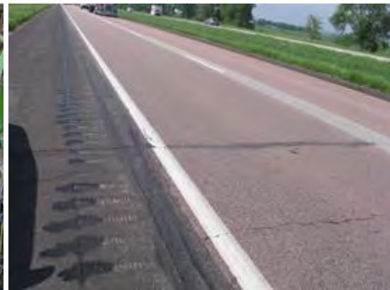
Reflection and transverse cracking
