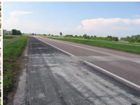
Reflection cracking/concrete patching
