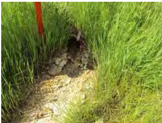
Pipe damaged during tufa removal
