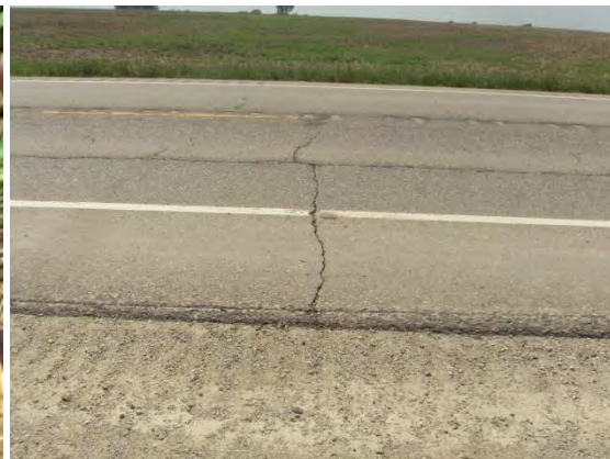
Longitudinal and transverse cracking
