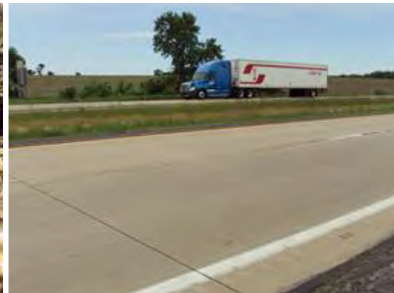
Longitudinal cracking along centerline
