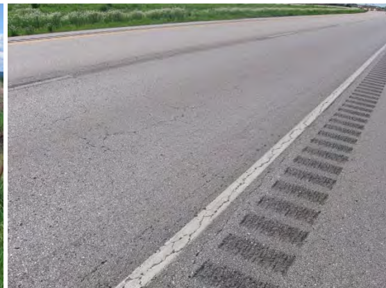
Alligator cracking/corner erosion damage
