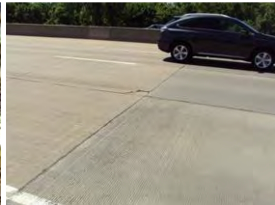
Small corner crack
