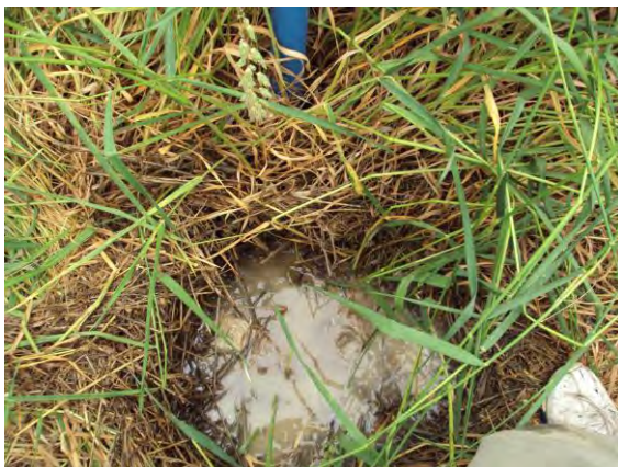
Soil blockage with standing water
