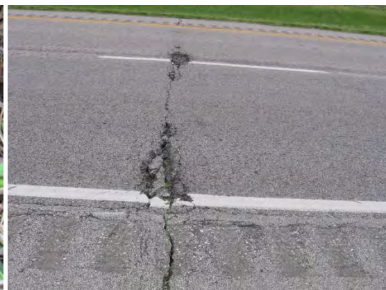
Transverse and alligator cracking
