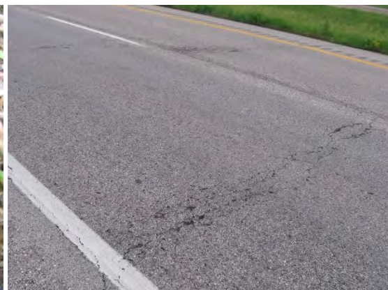
Transverse and alligator cracking/rutting
