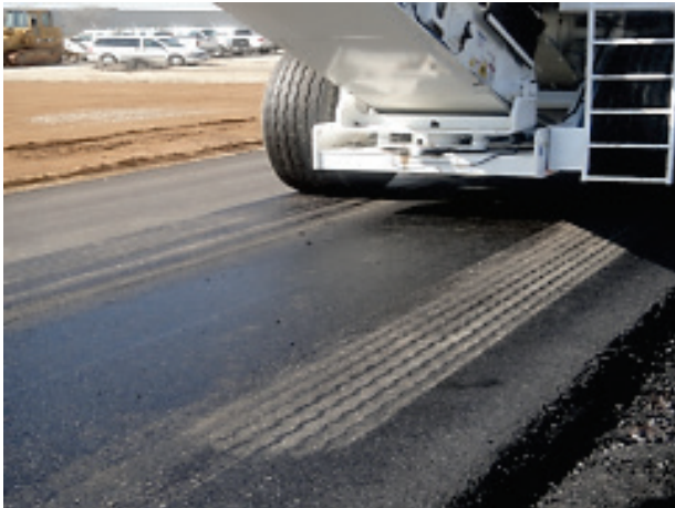
FIGURE 9 – Poor Performance of Conventional Tack Coat Material under Heavy Loads.
