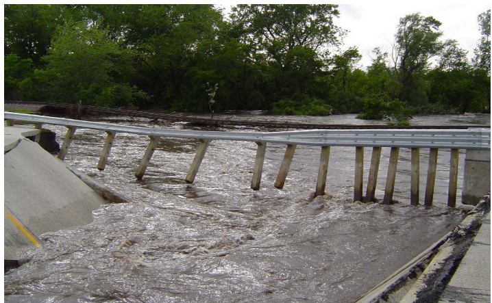
IA 6 (top) and IA 24 bridge in Winneshiek County (bottom) during 2008 flood (Images: ©Iowa Department of Transportation)
