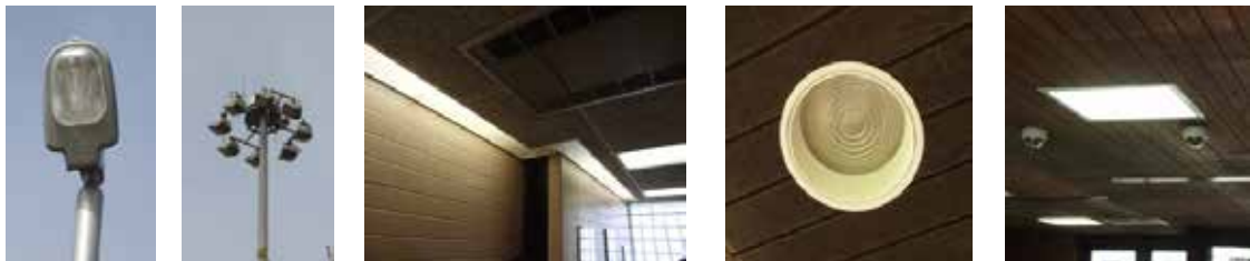
Figure 69. Lighting fixture in Cumberland Road rest area.
