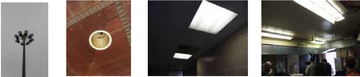
Figure 49. Lighting fixtures in southbound Coalfield rest area.
