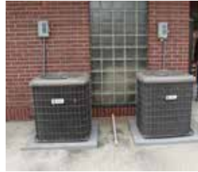
Air-cooled condensing units
