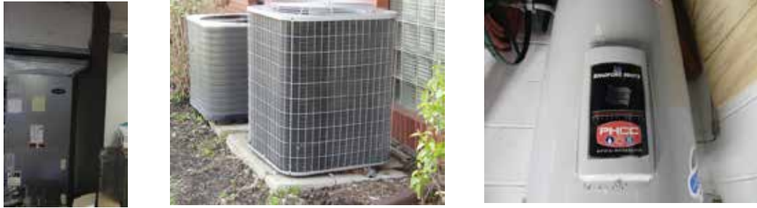
Figure 70. Air-conditioning units and water heater in Cumberland Road rest area.
