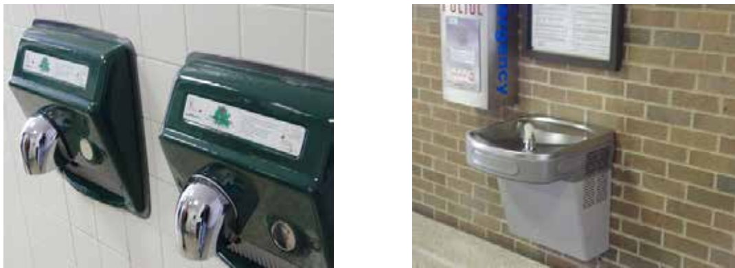
Figure 79. Hand dryers and water coolers in Turtle Creek rest area.
