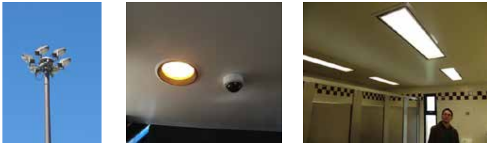
Figure 55. Lighting fixtures in westbound Great Sauk Trail rest area.
