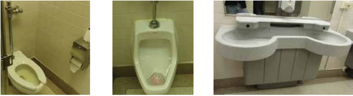
Figure 67. Water fixtures in Mackinaw Dells rest area.
