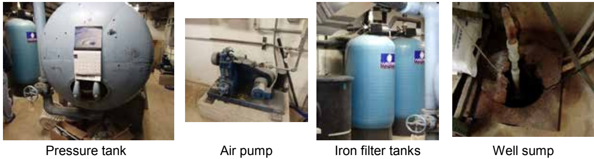
Figure 57. Water-treatment system components in Great Sauk Trail rest area.
