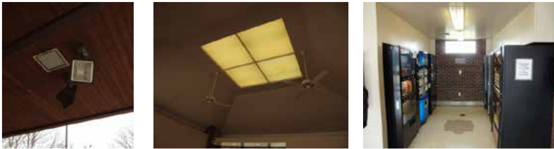
Figure 62. Lighting fixtures in Mackinaw Dells rest area.
