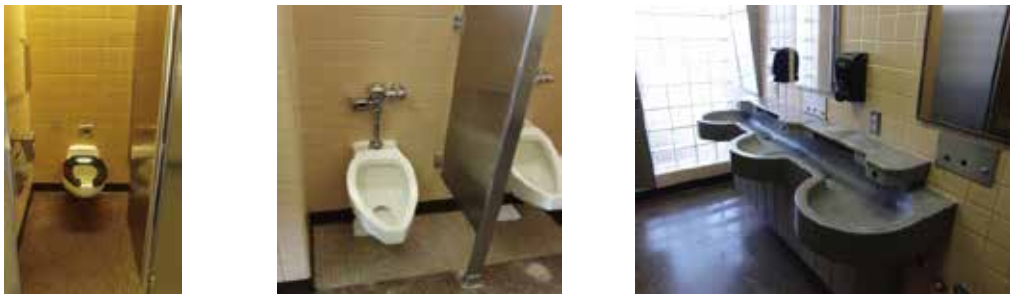
Figure 73. Water fixtures in Cumberland Road rest area.
