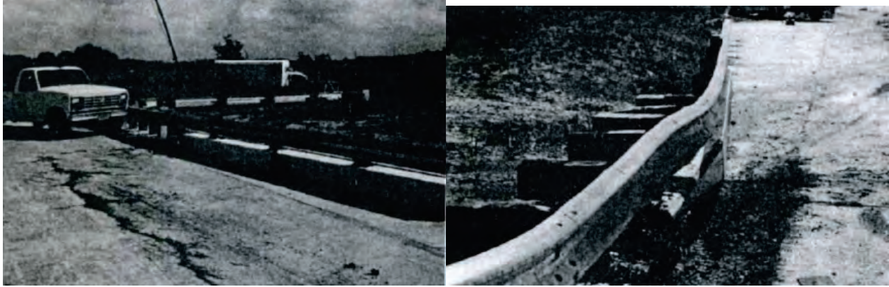
Figure 1.13. Impact Conditions and System Damage for YC-7 (3).
