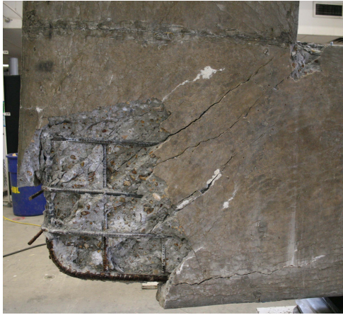
(c) Interior and Exterior Corner after Removal of Spalled Concrete (Opposite Face Shown in b)
