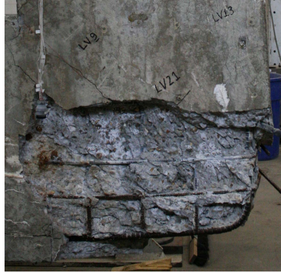
(b) Exterior Corner after Removal of Spalled Concrete (Opposite Face Shown in c)
