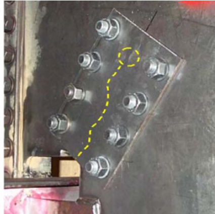
Figure 2-24. Bolted doubler plate retrofit (the dashed line and the circle represent a crack and a drilled hole to remove the crack tip) (Dexter and Ocel 2013)
