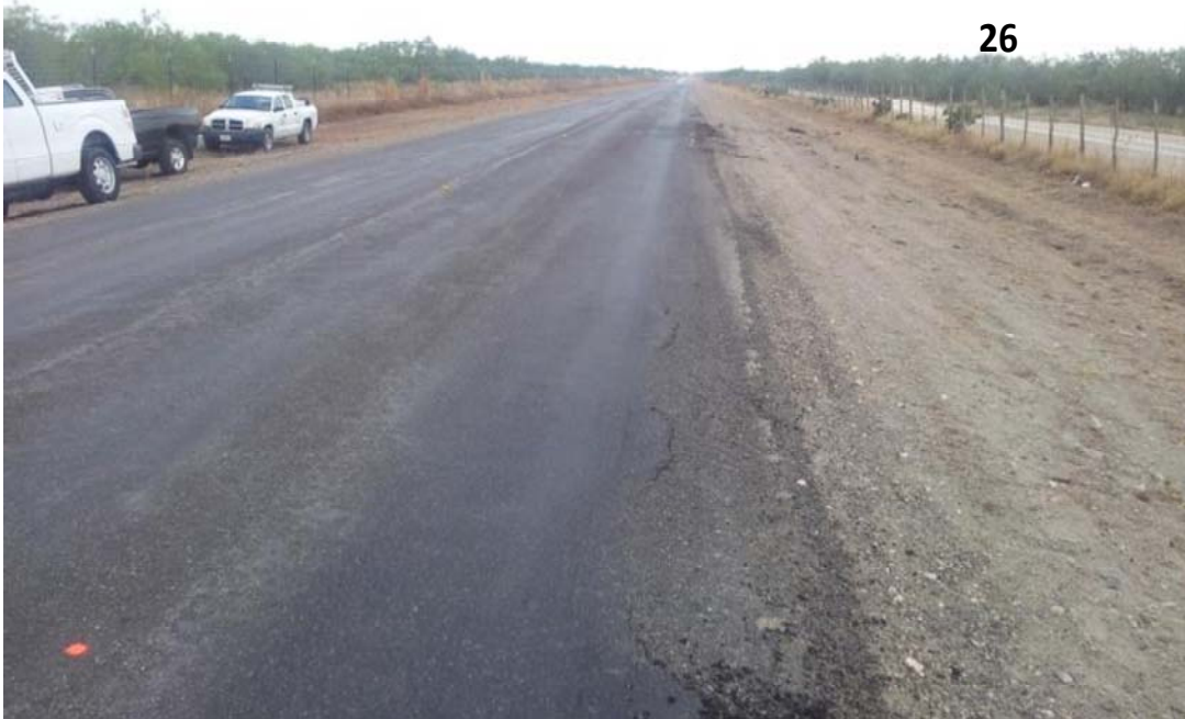
Figure 21. Rutting Failure of LRA Overlay in Dimmit County, Laredo District.
