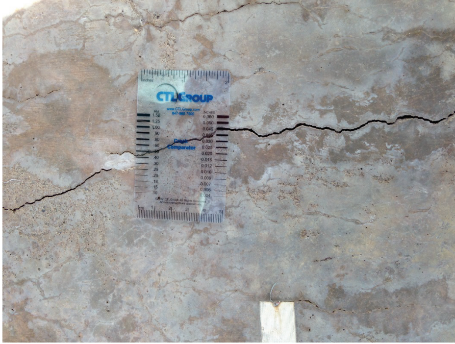
Figure 3-9. Larger Longitudinal Crack Width on Specimen LSC4.
