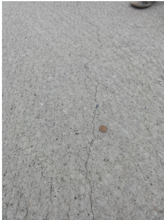
Figure C-3 Cracking in Dannon Way northbound internally cured concrete deck at 1 year.
