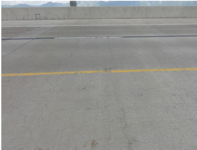
Figure C-10 Reflection and map cracking in 8200 South northbound conventional concrete deck at 2 years.
