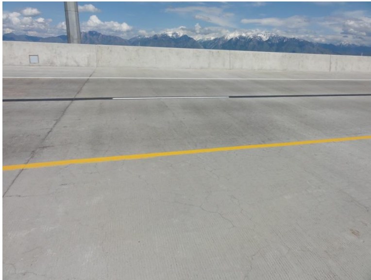
Figure C-9 Reflection and map cracking in 8200 South northbound conventional concrete deck at 1 year.
