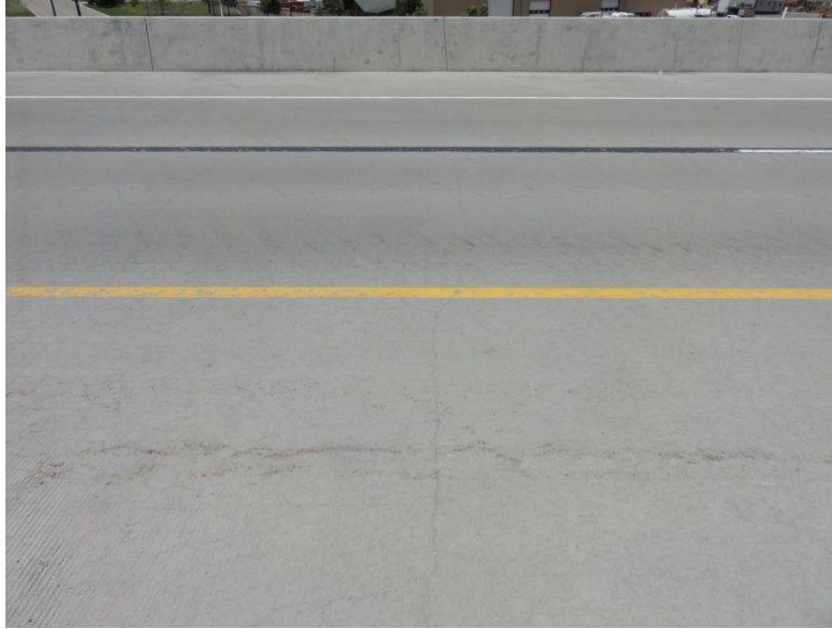
Figure C-2 Reflection cracking from half-deck concrete panels in Dannon Way northbound internally cured concrete deck at 2 years.
