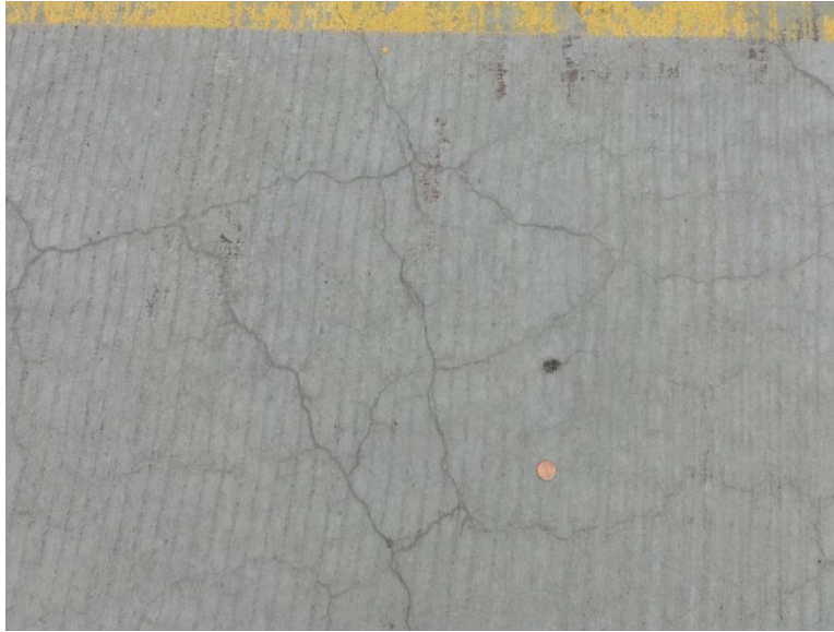
Figure C-8 Cracking in 8200 South northbound conventional concrete deck at 2 years.
