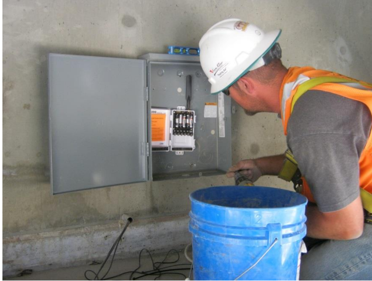
Figure 3-8 Data logger mounted in box.
