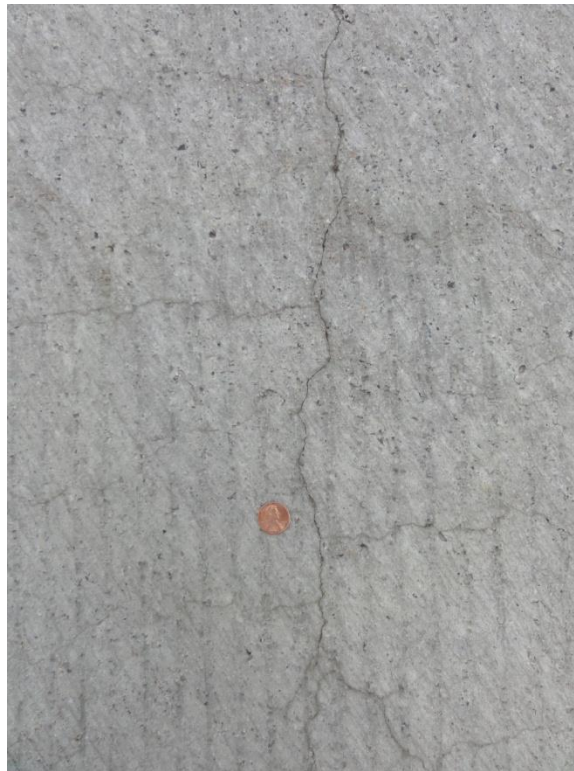
Figure C-4 Cracking in Dannon Way northbound internally cured concrete deck at 2 years.
