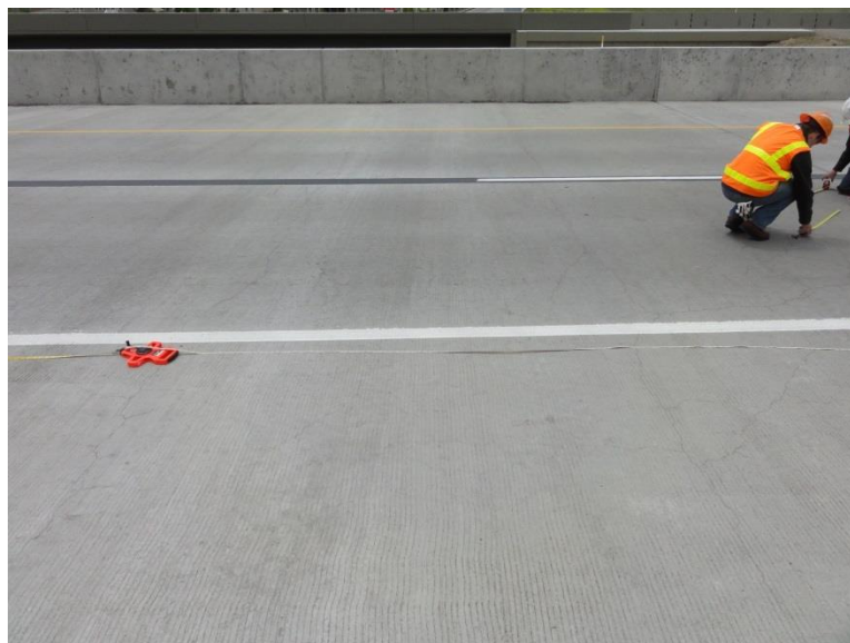
Figure C-5 Reflection cracking from half-deck concrete panels in 8200 South northbound conventional concrete deck at 1 year.
