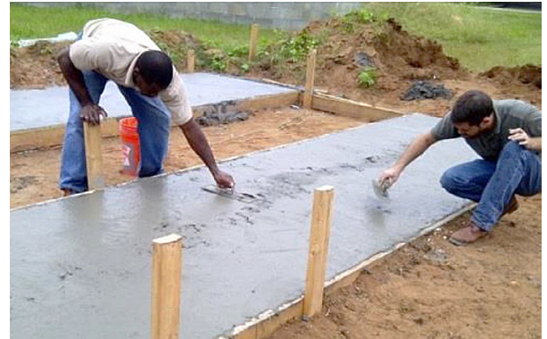
Workers put the finishing touches on a slab of concrete made with ground tire rubber.
