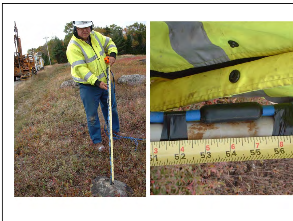
Fig E-21. Thermistor Cables Mounted on Wooden Dowel
