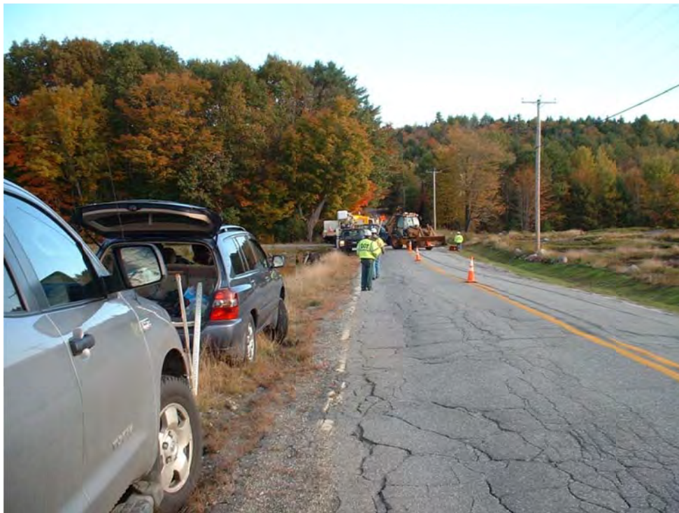
Figure 10. Cracked pavement at Mariaville site (near top of hill facing north).
