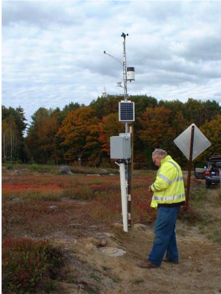
Figure 12. Completed Installation at Mariaville-1 site
