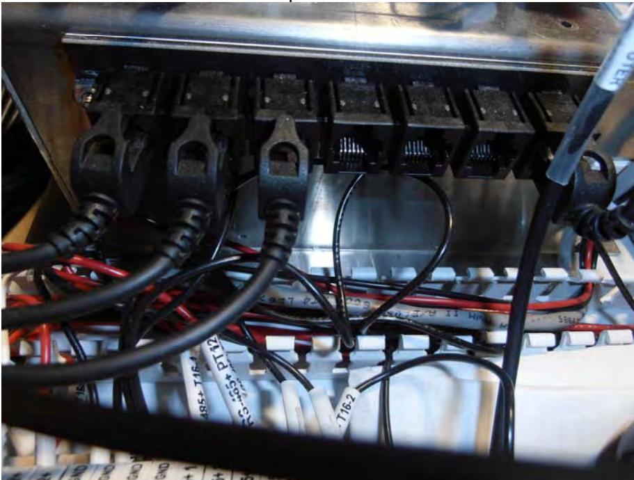
Smart Sensors connected to Expansion Module
