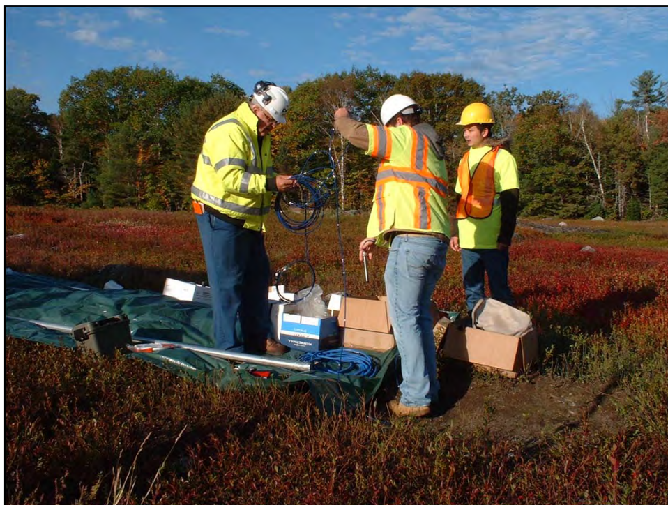
Fig E-3. Water Well Pressure Transducer
