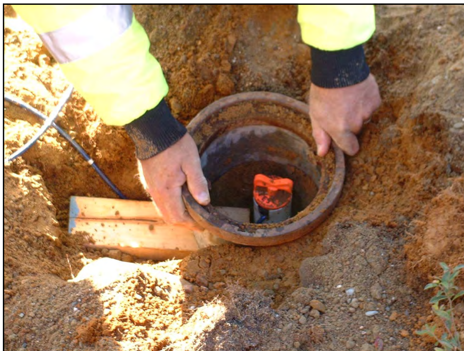
Fig E-5. Water Well Protective Casing
