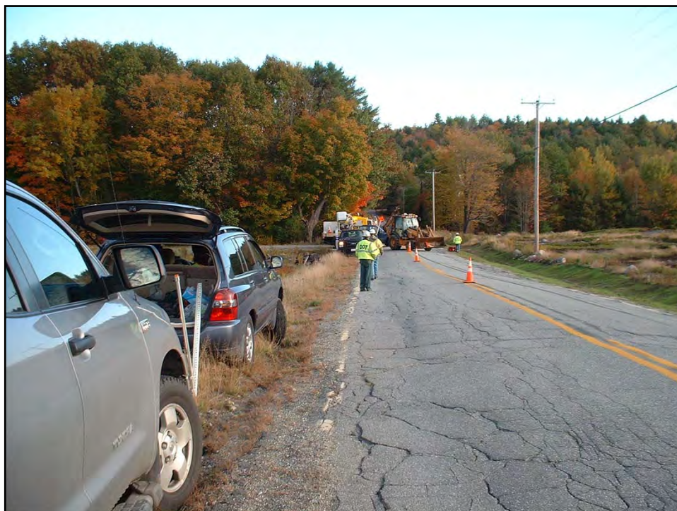
Fig E-1. Cracked Pavement Just North of Installation
