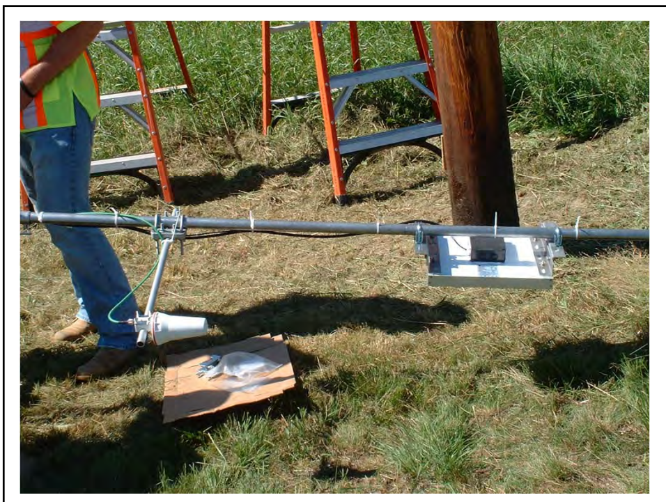
Fig D-4. Solar Panel and Air Temperature Sensor
