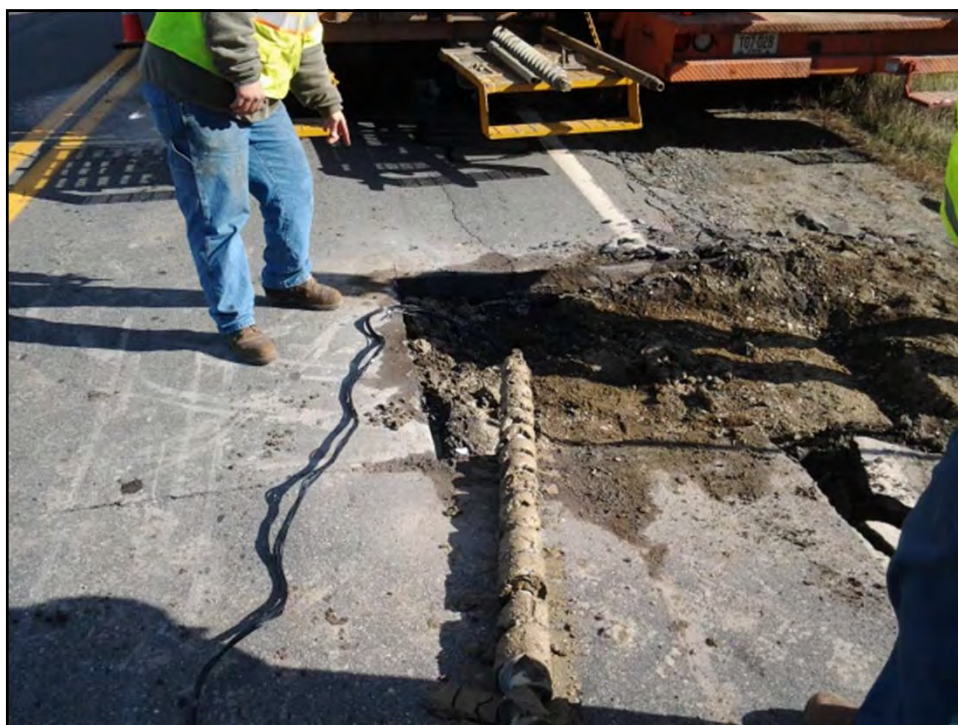
Fig F-4. Cable from Installed Temperature Sensors in Borehole
