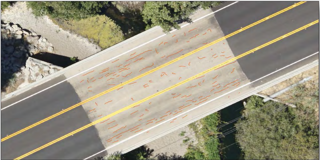
Figure C.2.11: Bridge NO. 53C0775 Crack Image
