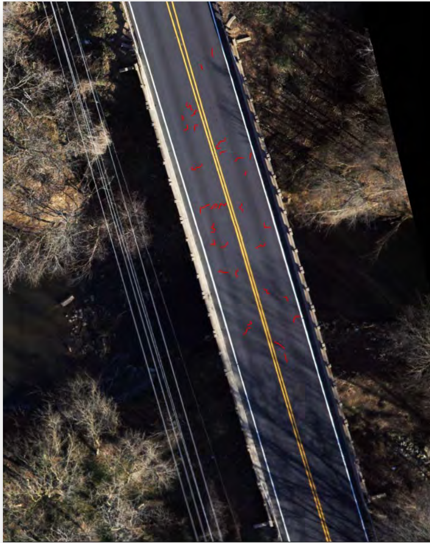
Figure C.5.9: Bridge NO. 590049 Crack Image
