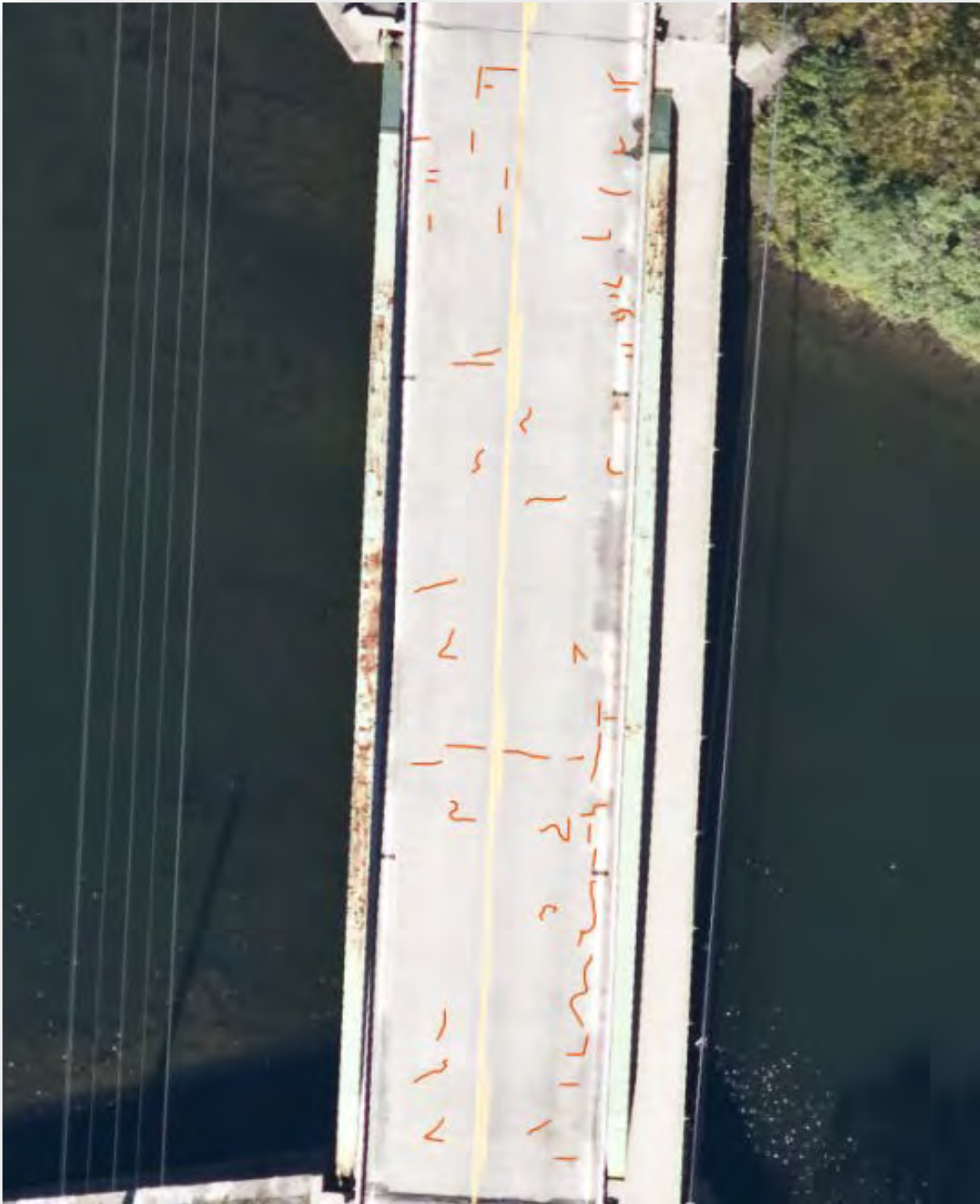
Figure C.8.30: Bridge NO. 1027090 Crack Image
