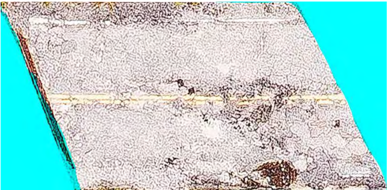
Figure 19: e.) Binary image of the area of interest with minor crack regions being identified using APBA; f.) Original image of the area of study being marked with minor cracks in red pixels
