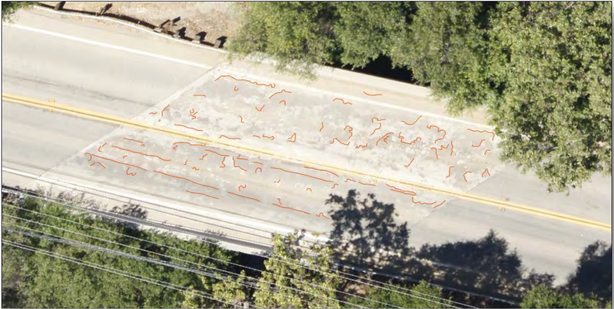
Figure C.2.22: Bridge NO. 53C0981 Crack Image
