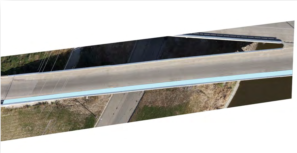
Figure C.4.20: Bridge NO. 42761 Obstruction Image
