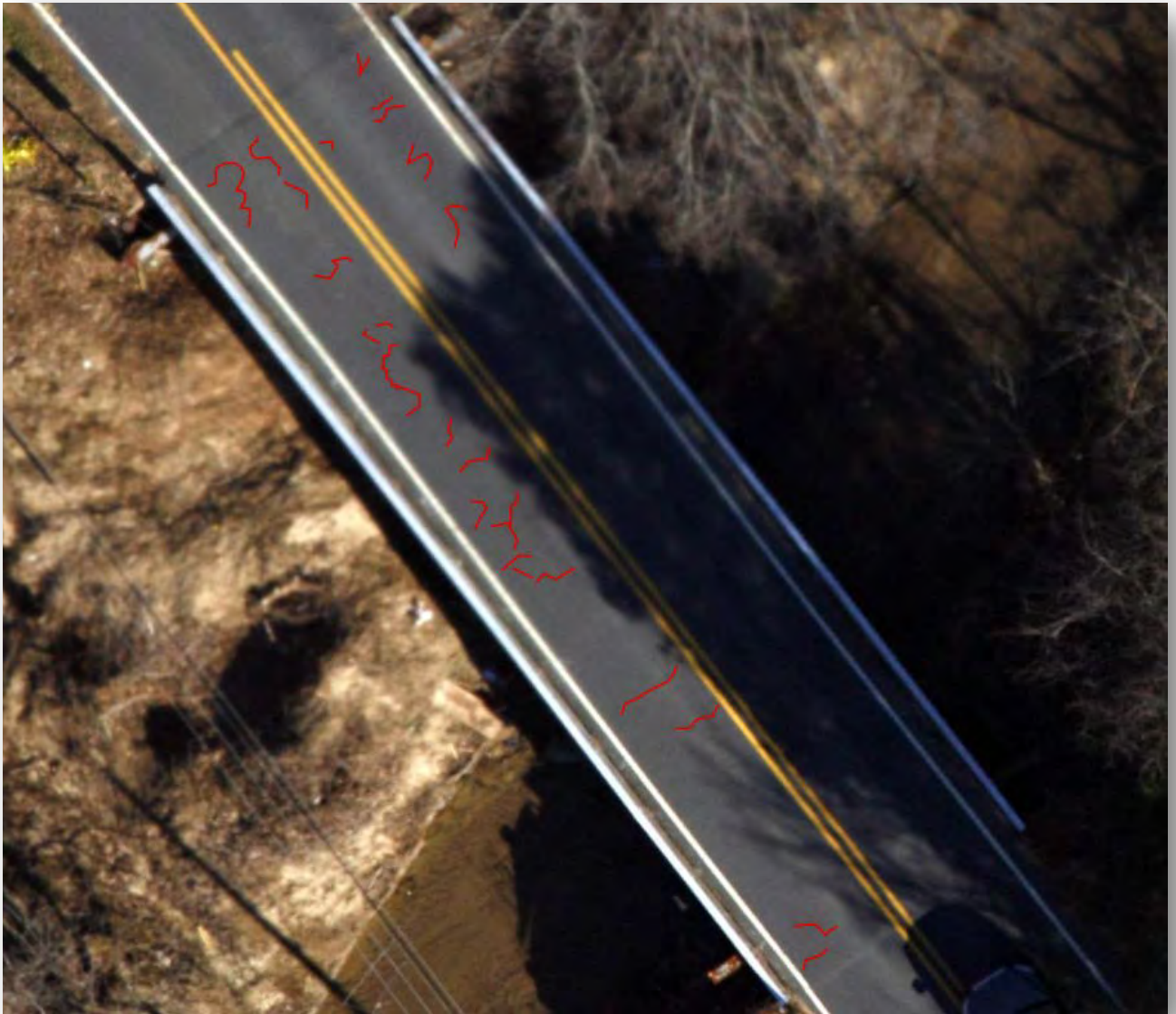
Figure C.5.12: Bridge NO. 590059 Crack Image
