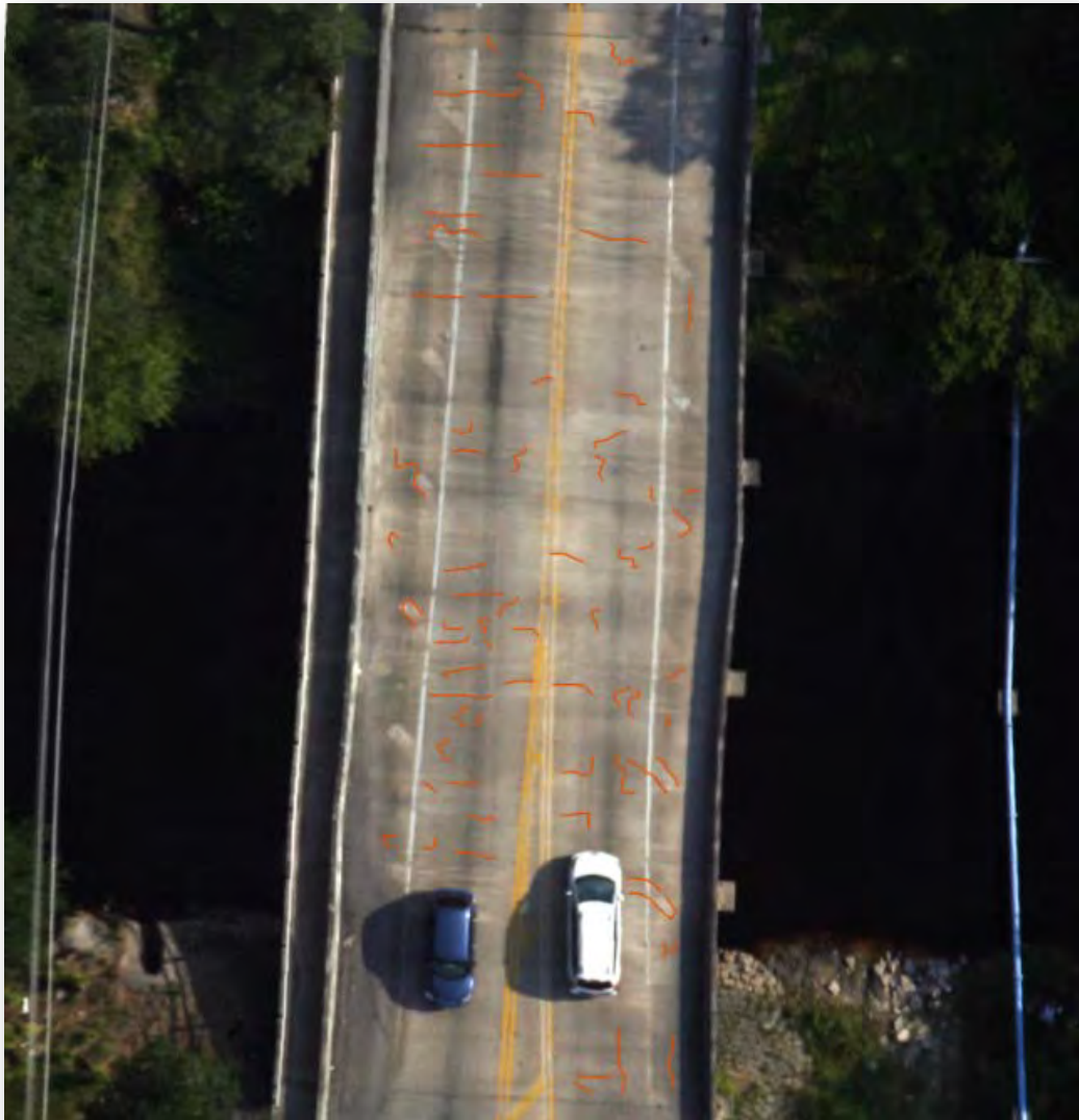
Figure C.3.22: Bridge NO. 924153 Crack Image
