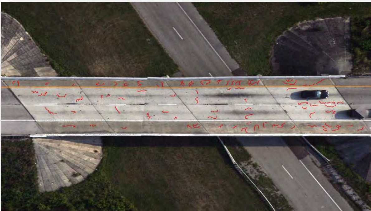
Figure C.3.6: Bridge NO. 750143 Crack Image
