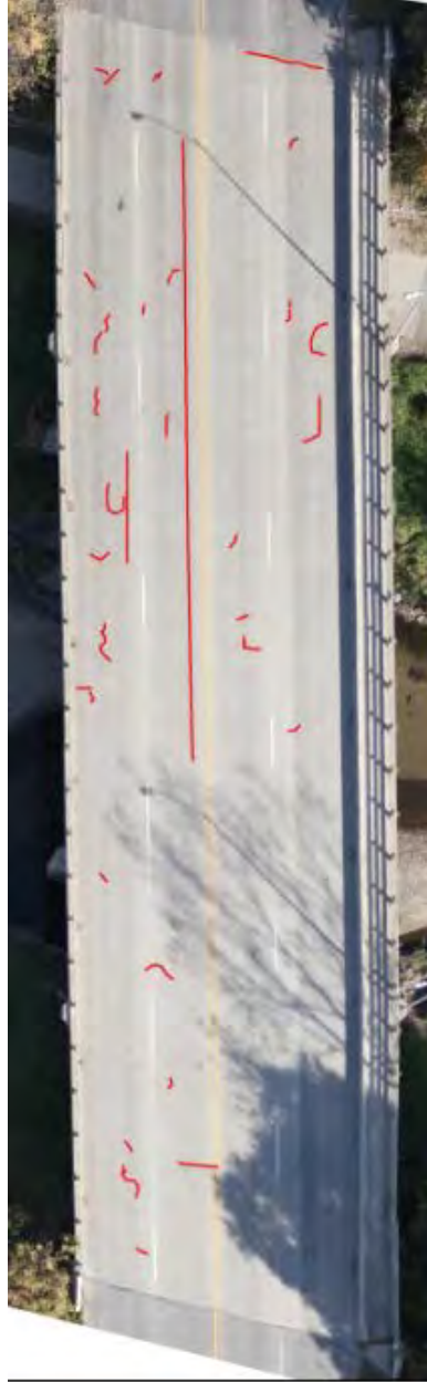
Figure C.4.3: Bridge NO. 3826 Crack Image
