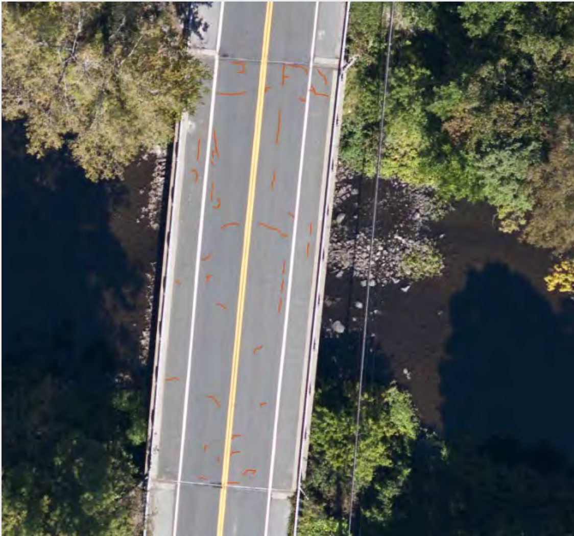
Figure C.8.33: Bridge NO. 1034880 Crack Image
