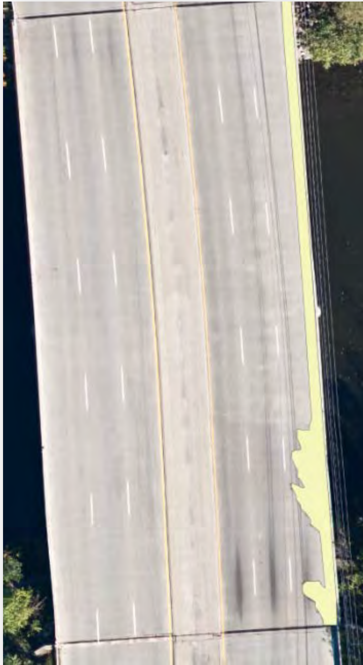
Figure C.8.2: Bridge NO. 1005220 Obstruction Image
