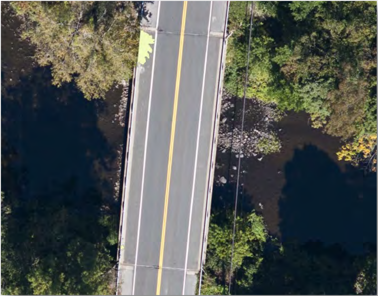
Figure C.8.32: Bridge NO. 1034880 Obstruction Image
