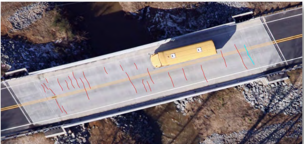
Figure C.6.6: Bridge NO. 374000000001790223 Crack Image
