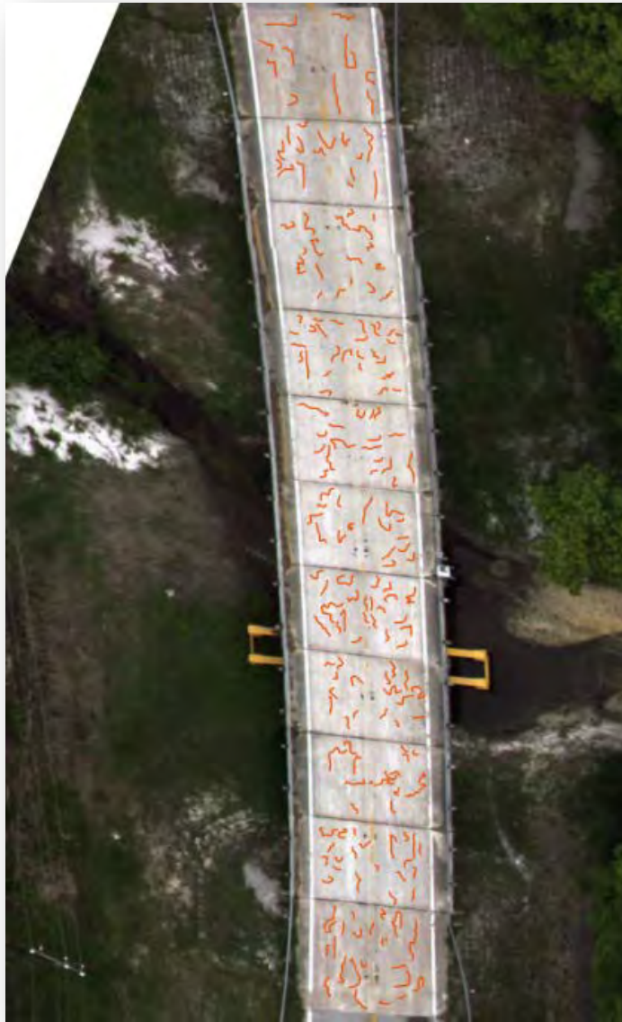
Figure C.3.17: Bridge NO. 924046 Crack Image
