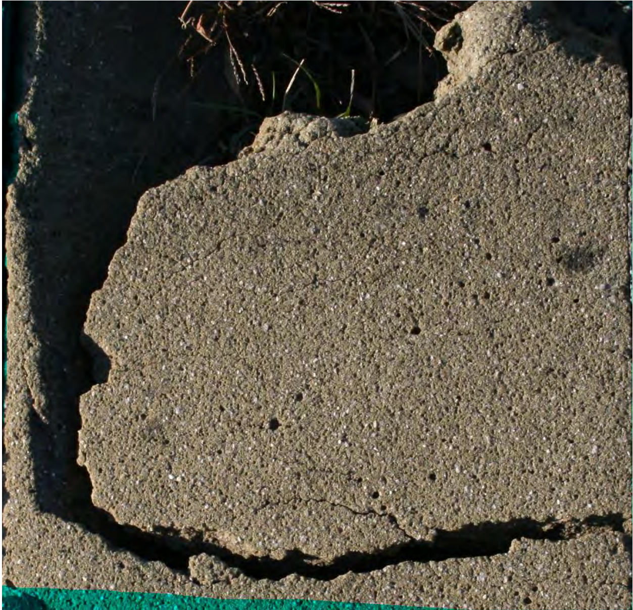
B.1.14: Original image of the area of study being marked with minor cracks in red pixels
