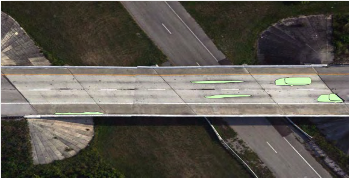
Figure C.3.5: Bridge NO. 750143 Obstruction Image
