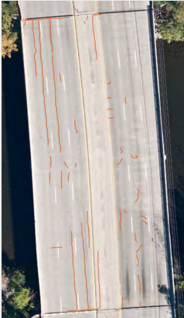
Figure C.8.3: Bridge NO. 1005220 Crack Image
