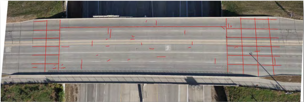
Figure C.4.6: Bridge NO. 12491 Crack Image
