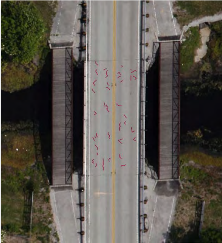
Figure C.3.15: Bridge NO. 924038 Crack Image
