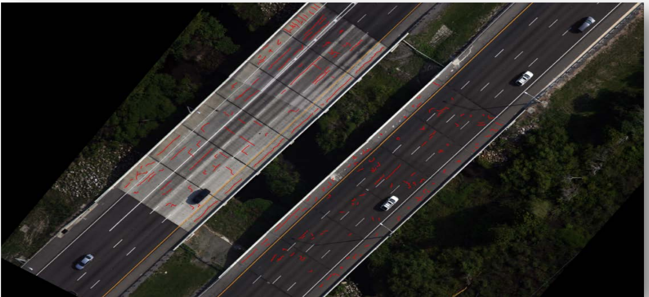
Figure C.3.12: Bridge NO. 920099 Crack Image
