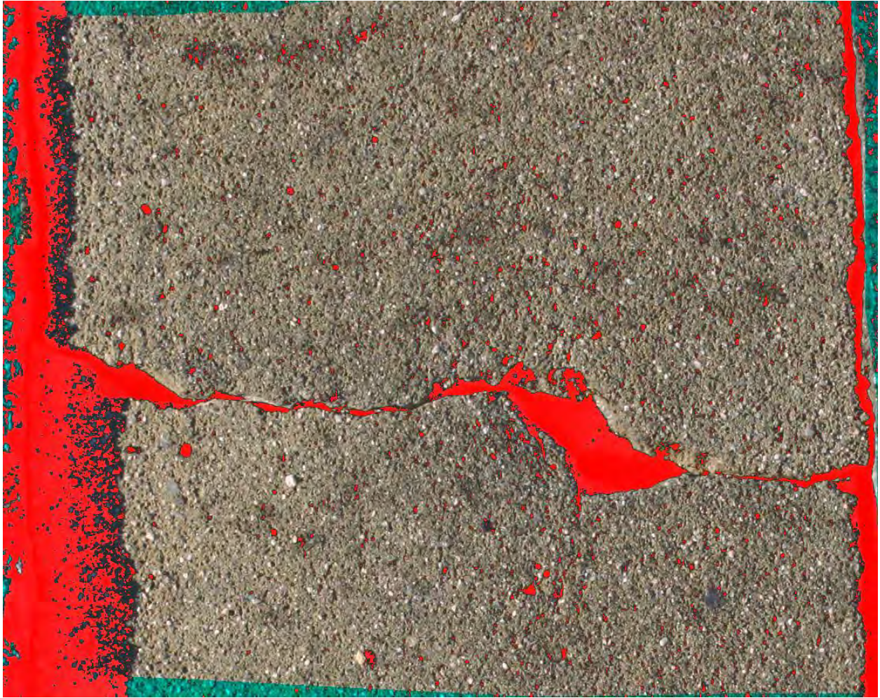
B.1.3: Original image of the area of study being marked with total damages in red pixels.
