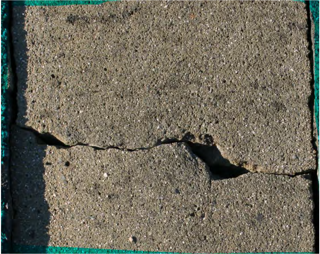
B.1.7: Original image of the area of study being marked with minor cracks in red pixels
