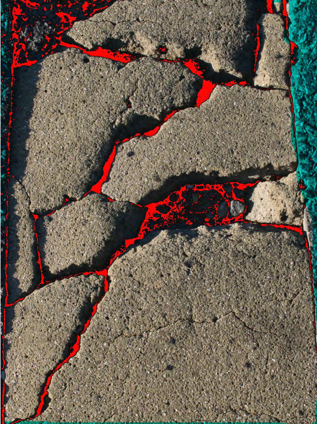
B.1.26: Original image of the area of study being marked with major cracks in red pixels
