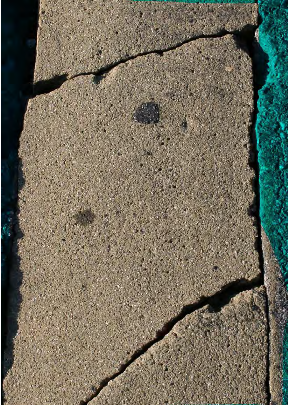
B.1.21: Original image of the area of study being marked with minor cracks in red pixels
