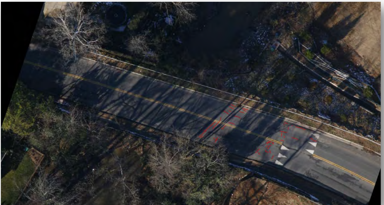
Figure C.6.3: Bridge NO. 1190447 Crack Image
