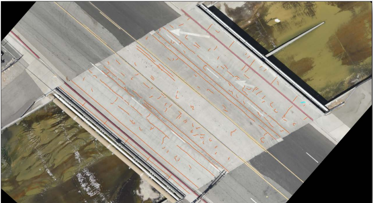
Figure C.2.25: Bridge NO. 53C1008 Crack Image
