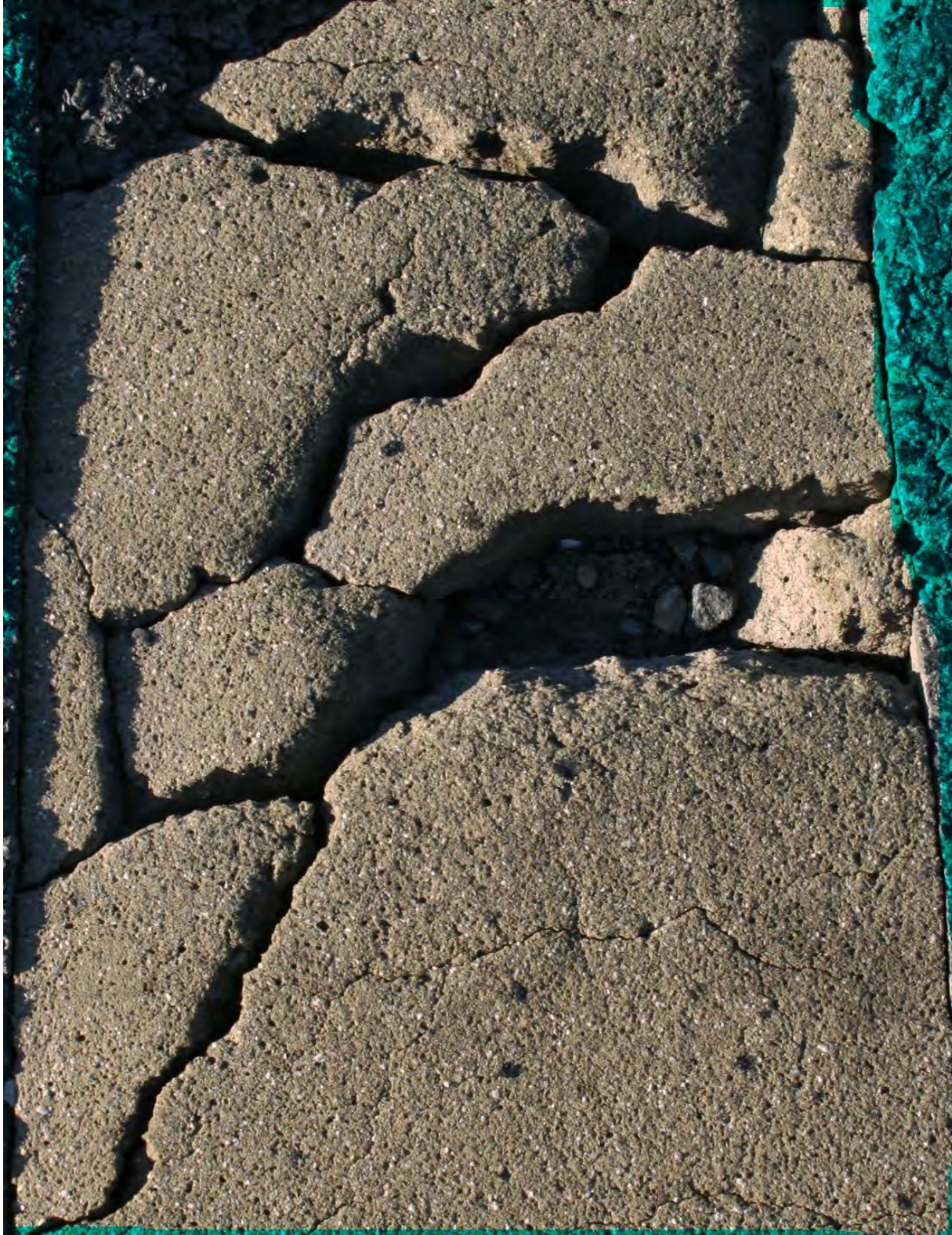
B.1.28: Original image of the area of study being marked with minor cracks in red pixels
