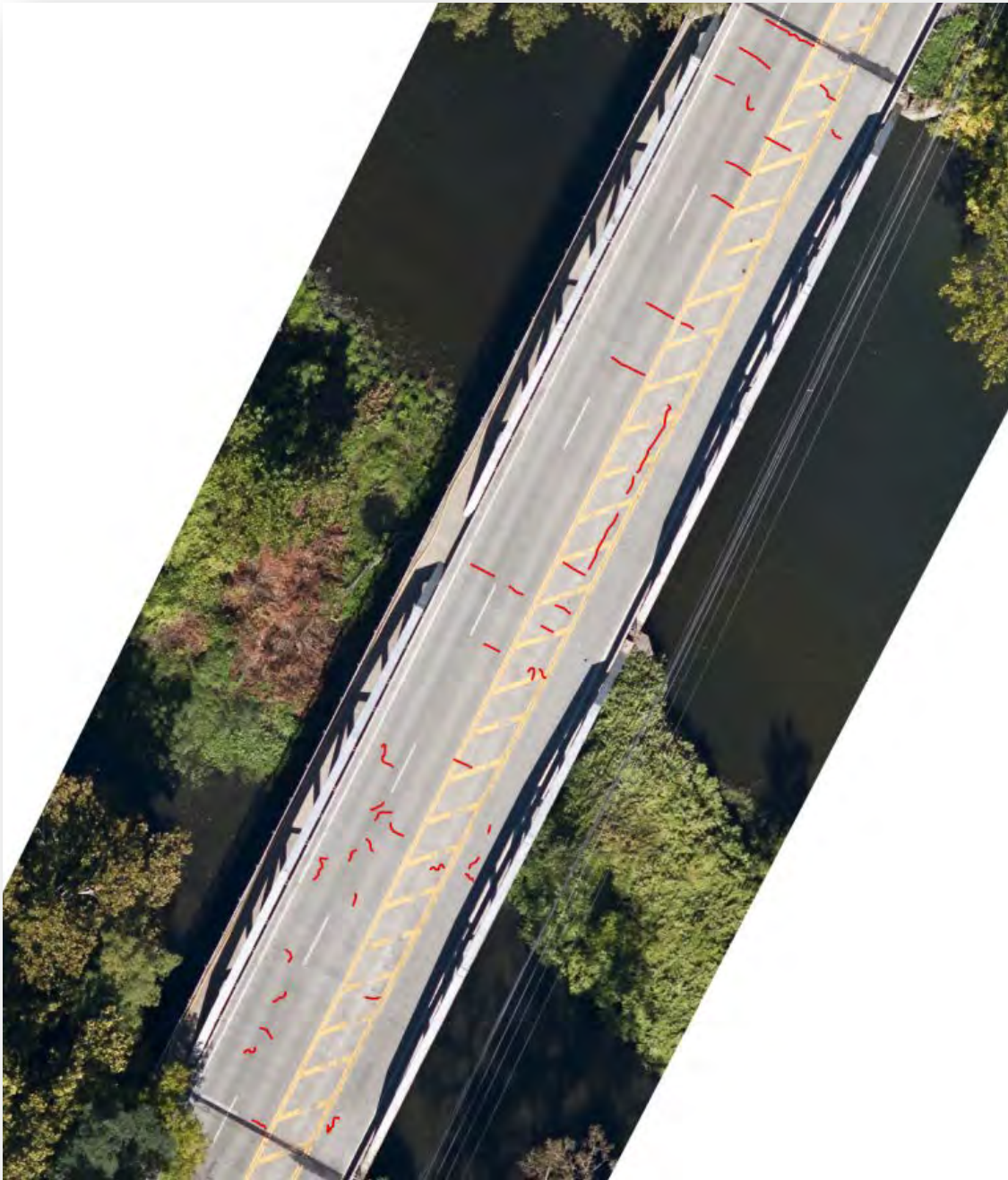
Figure C.8.1525: Bridge NO. 1007260 Crack Image
