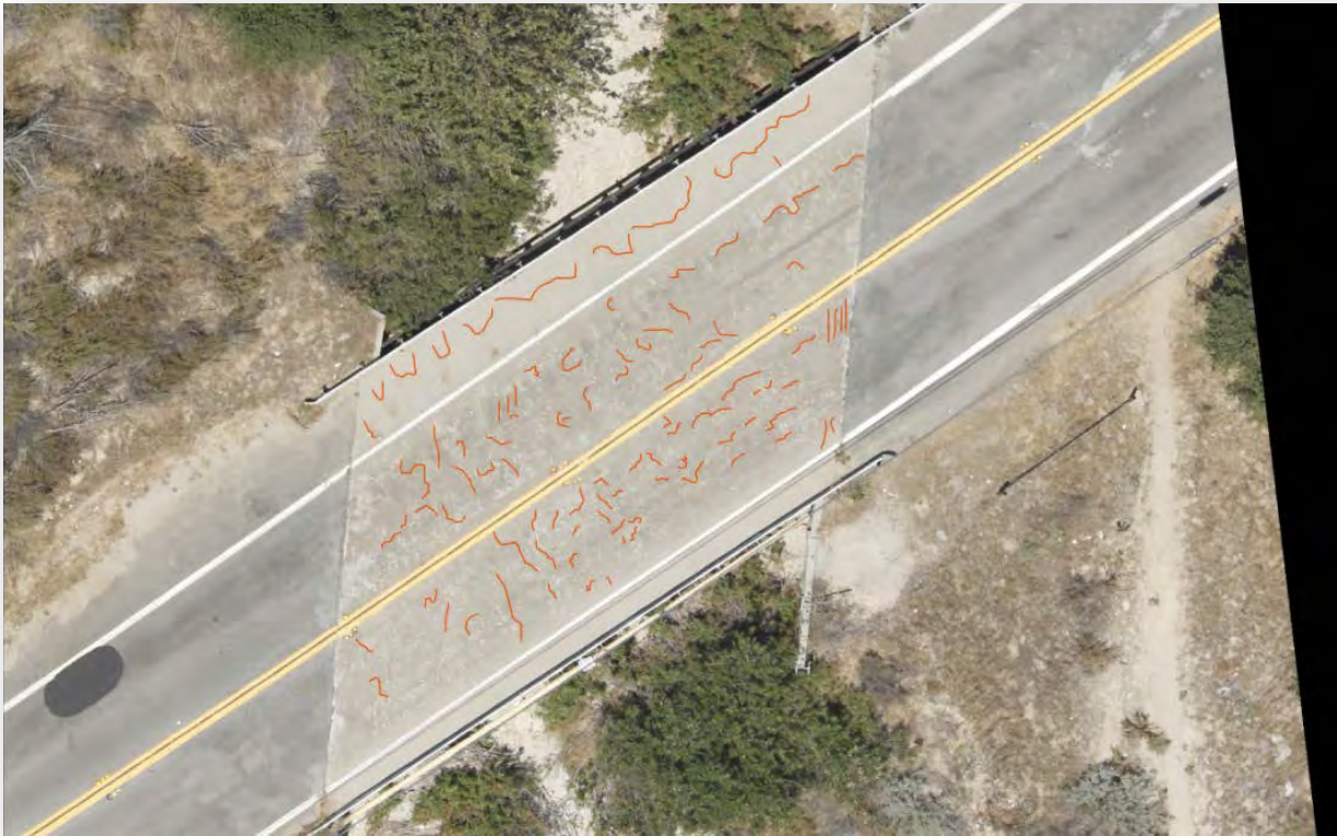
Figure C.2.1612: Bridge NO. 53C1527 Crack Image
