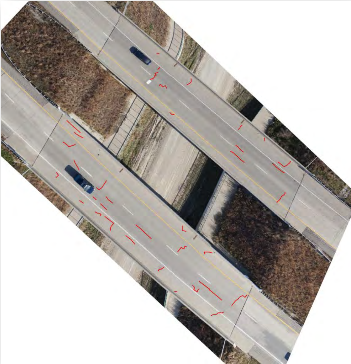
Figure C.4.36: Bridge NO. 608660 Crack Image
