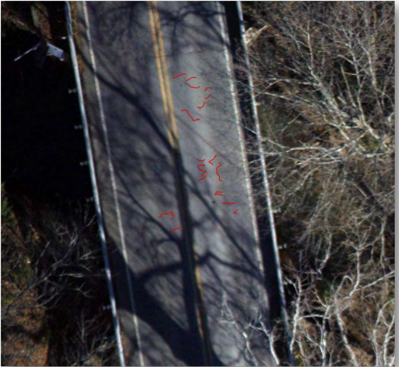
Figure C.5.15: Bridge NO. 590038 Crack Image
