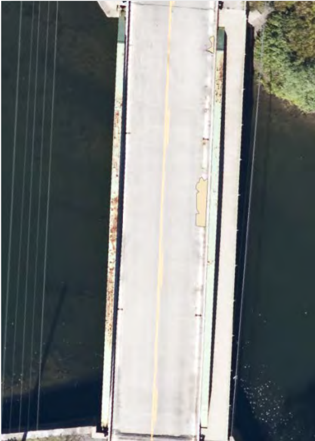
Figure C.8.29: Bridge NO. 1027090 Obstruction Image
