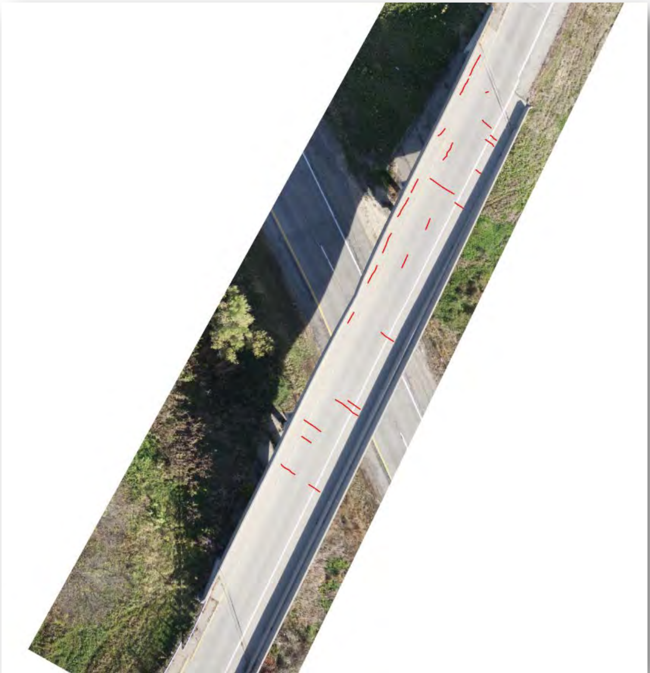
Figure C.4.24: Bridge NO. 605405 Crack Image
