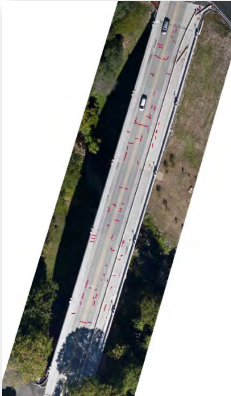
Figure C.8.9: Bridge NO. 1007140 Crack Image
