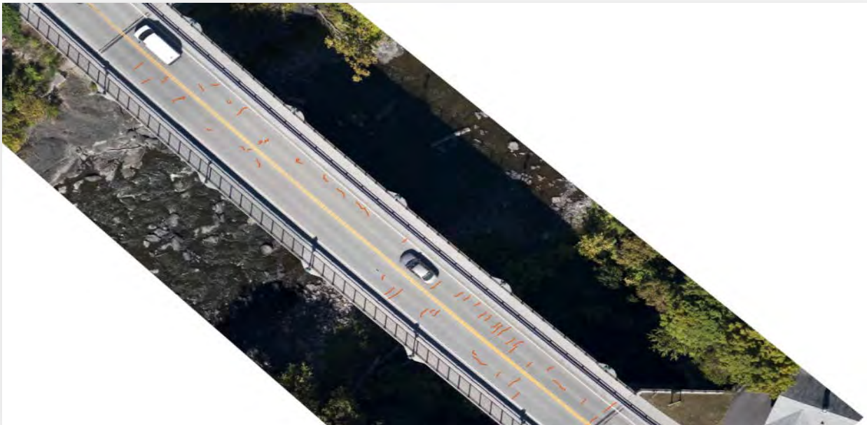
Figure C.8.27: Bridge NO. 1026680 Crack Image
