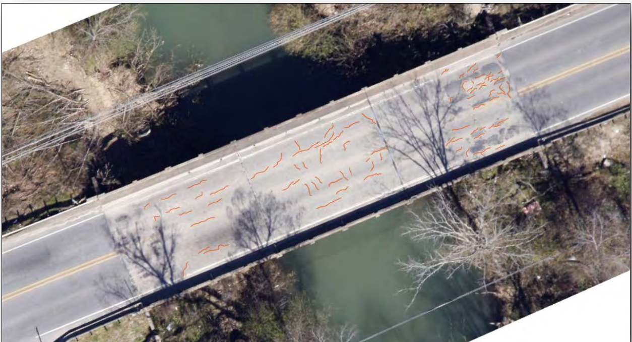
Figure C.1.3: Bridge NO. 003267 Crack Image
