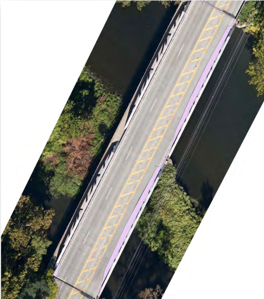
Figure C.8.14: Bridge NO. 1007260 Obstruction Image
