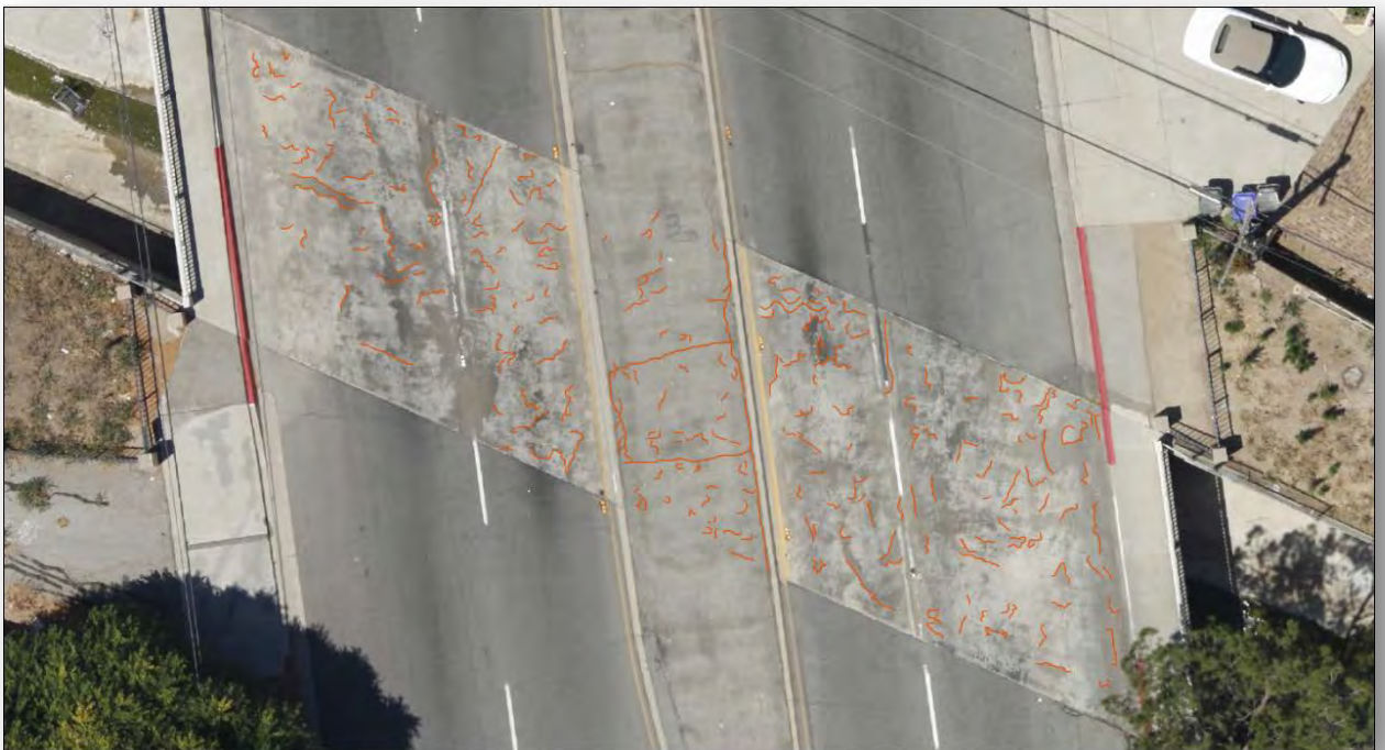
Figure C.2.14: Bridge NO. 53C0470 Crack Image
