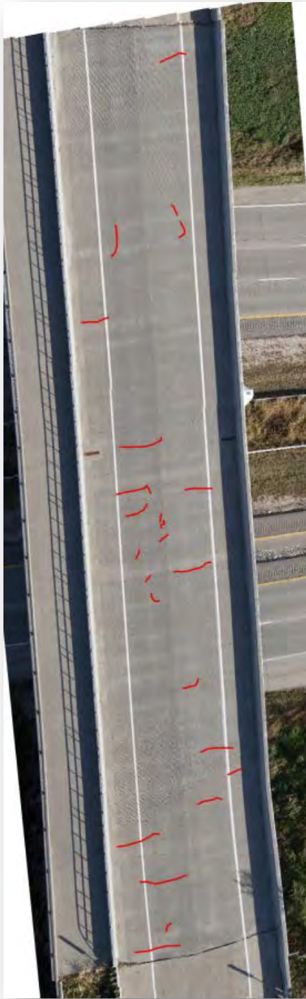
Figure C.4.30: Bridge NO. 608575 Crack Image
