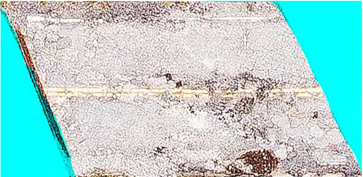
Figure 18: Cropped section (span A) of the bridge under study using APBA software
