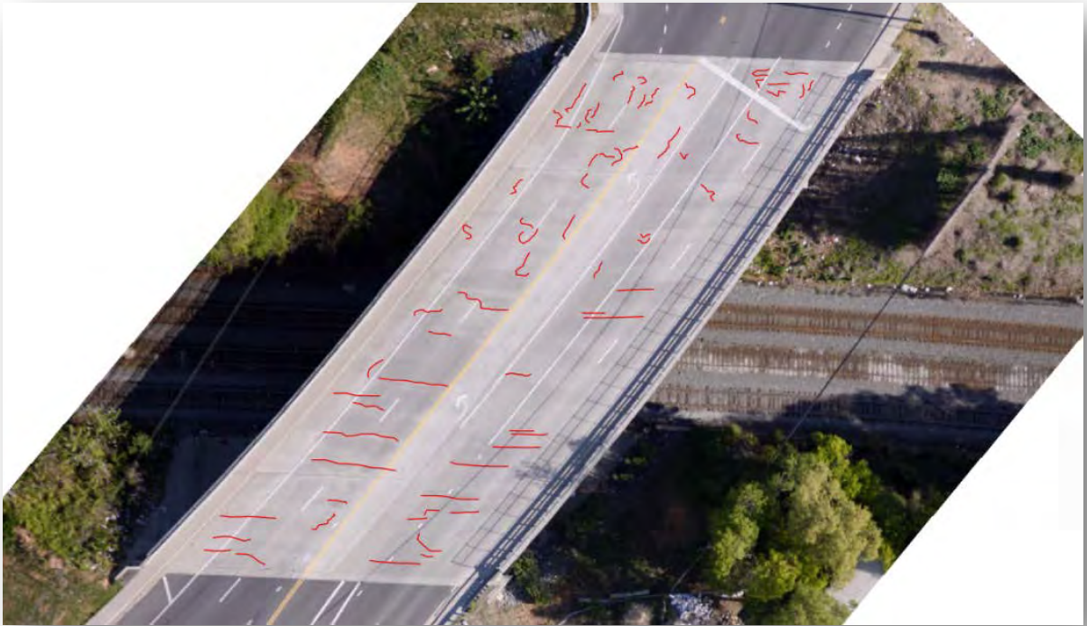
Figure C.5.622: Bridge NO. 590108 Crack Image
