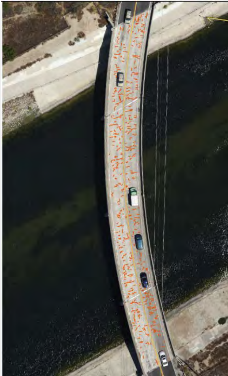
Figure C.2.8: Bridge NO. 53C0602 Crack Image
