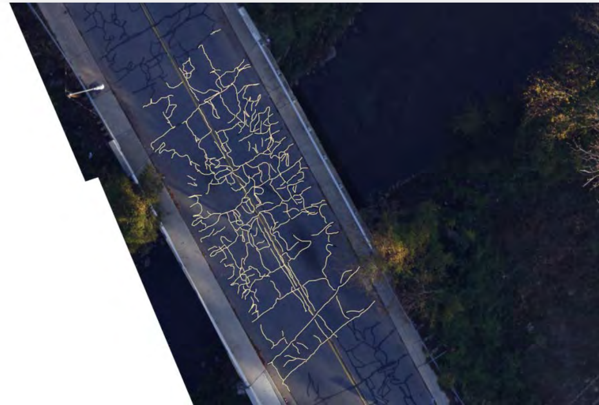
Figure C.7.4: Bridge NO. 590376 Crack Image
