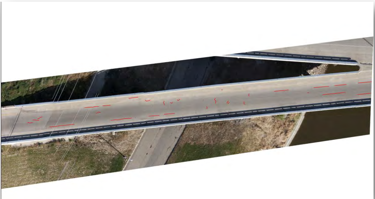
Figure C.4.21: Bridge NO. 42761 Crack Image
