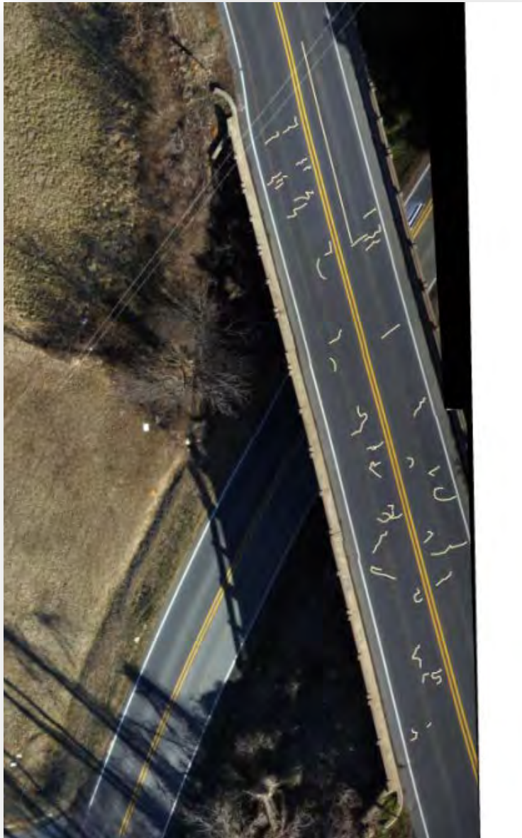
Figure C.5.24: Bridge NO. US21 St. 2004 Crack Image
