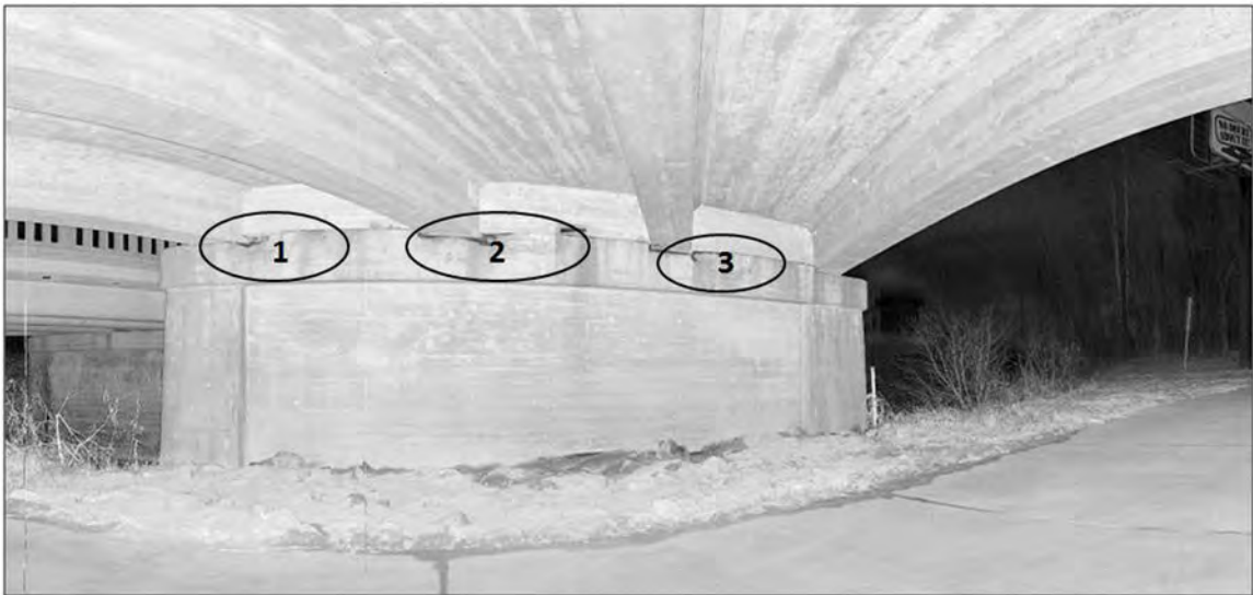
Figure 11. The LiDAR scan result of the damage
