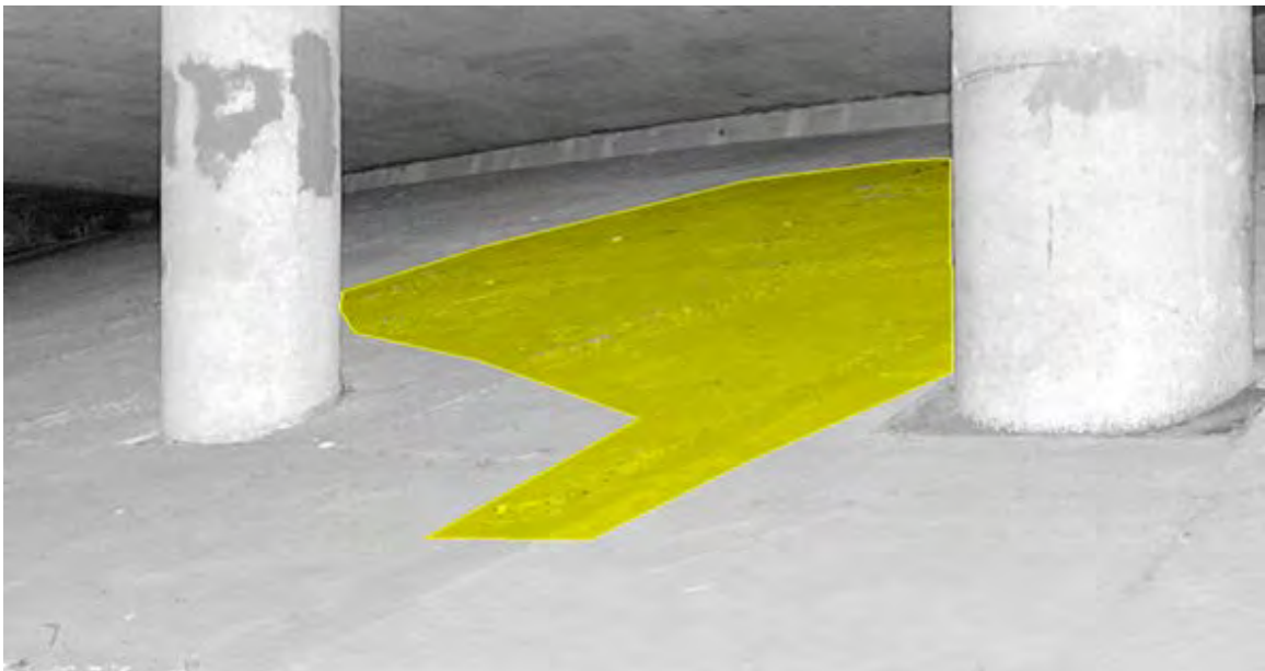
Figure 22. The large scale mass loss in Bridge 42300
